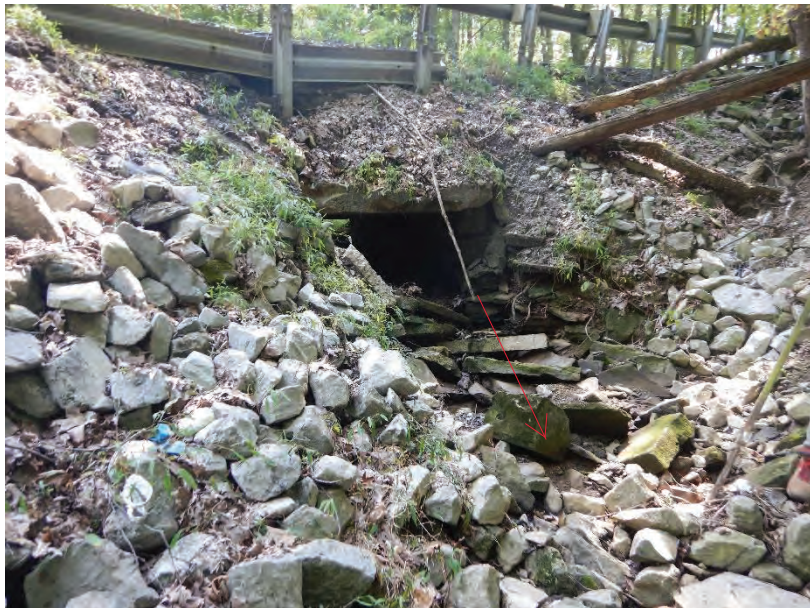
Photo 15: Within UNT 1 to Tipton Creek Facing South Towards Structure on Northside of SR 58
