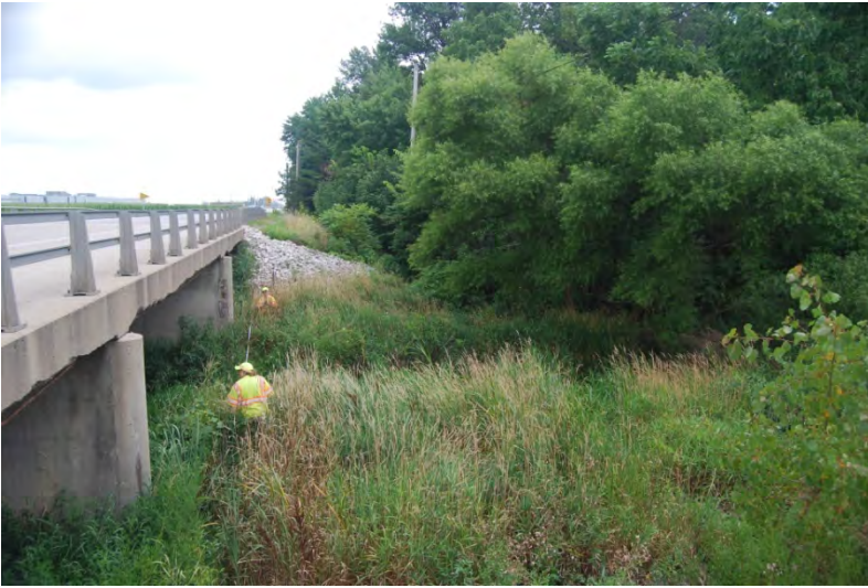
113 – View E of Dixon Cr at SR 28 from SW quad of bridge.
