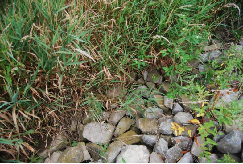
005 – View of riprap bottom of ditch in NE quad of Dixon Cr, E of NB US 31.
