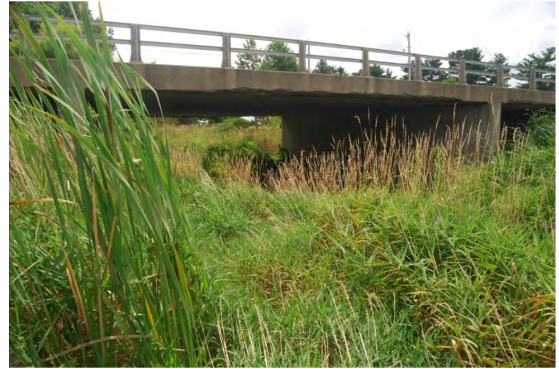
134 – View S from NE quad of Dixon Cr and SR 28; Wetland F.
