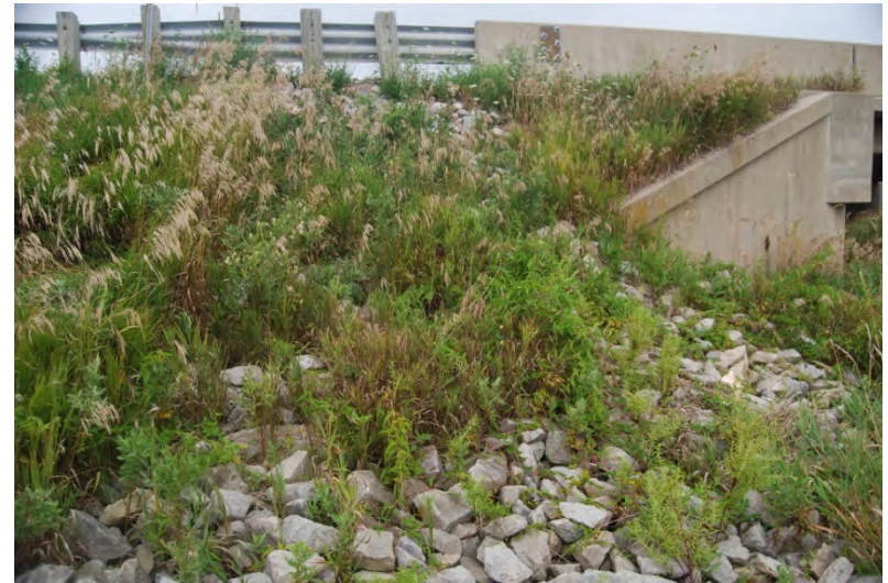
012 – View W from ditch in SE quad of Dixon Cr at E side of NB US 31.
