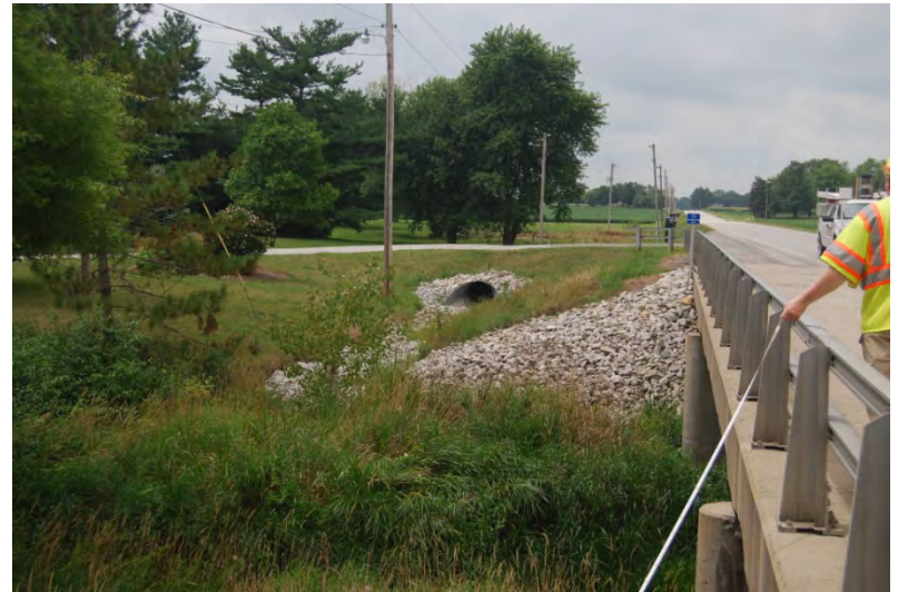
108 – View W of Dixon Cr at SR 28 from SE quad of bridge.
