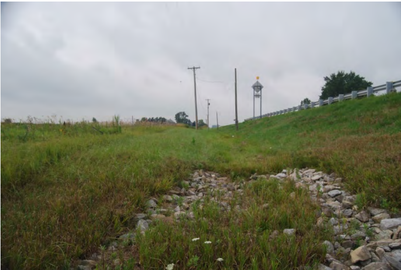
011 – View N of ditch in SE quad of Dixon Cr at E side of NB US 31.
