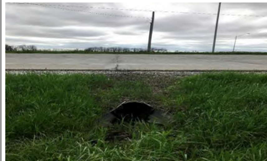
Photo 3. Looking east toward a drainage pipe that runs underneath US 421, approximately 0.02 mile north of the US 6 and US 421 intersection.
