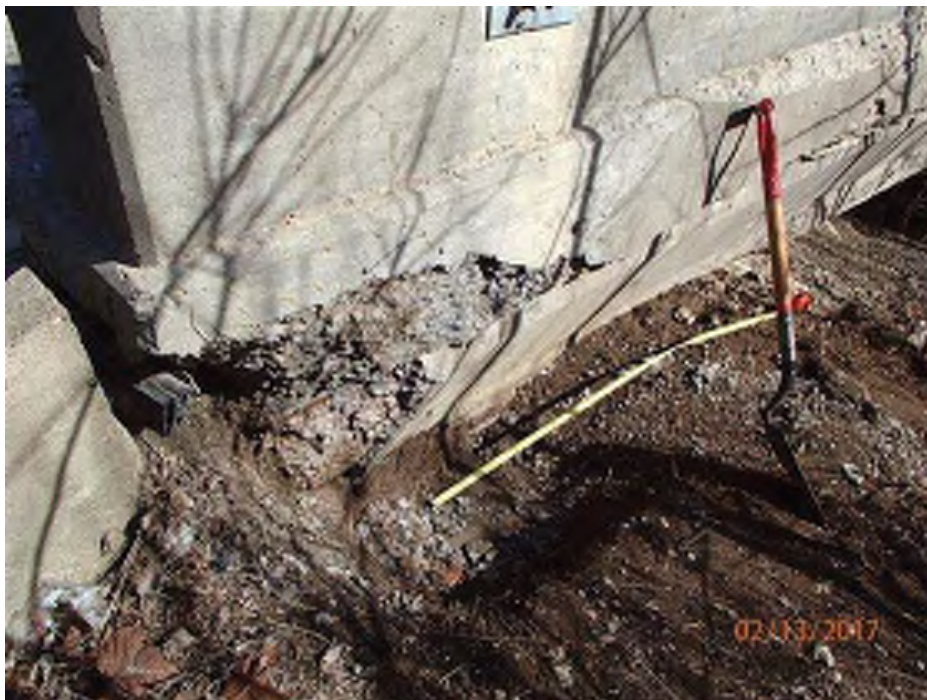
PHOTO 36 Condition Description 02-13-2017 (421)39-12-01792 B Span C beam 1 at the north bent looking southeast
