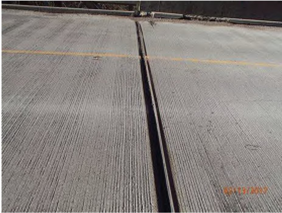
PHOTO 1 Condition Description 02-13-2017 (421)39-12-01792 B North interior joint condition
