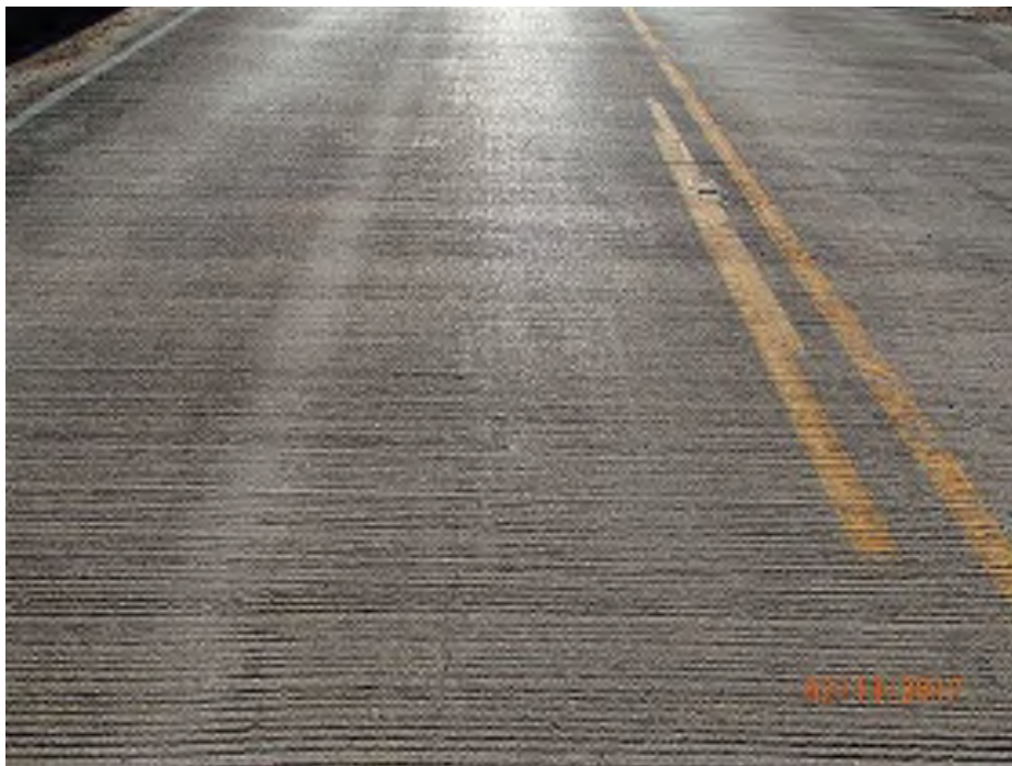
PHOTO 49 Condition Description 02-13-2017 (421)39-12-01792 B Span C wearing surface has longitudinal cracking
