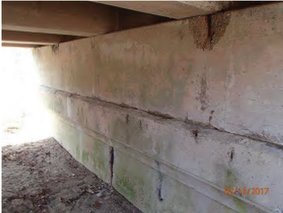
PHOTO 7 Condition Description 02-13-2017 (421)39-12-01792 B Pier 2 south face cap and stem spalling
