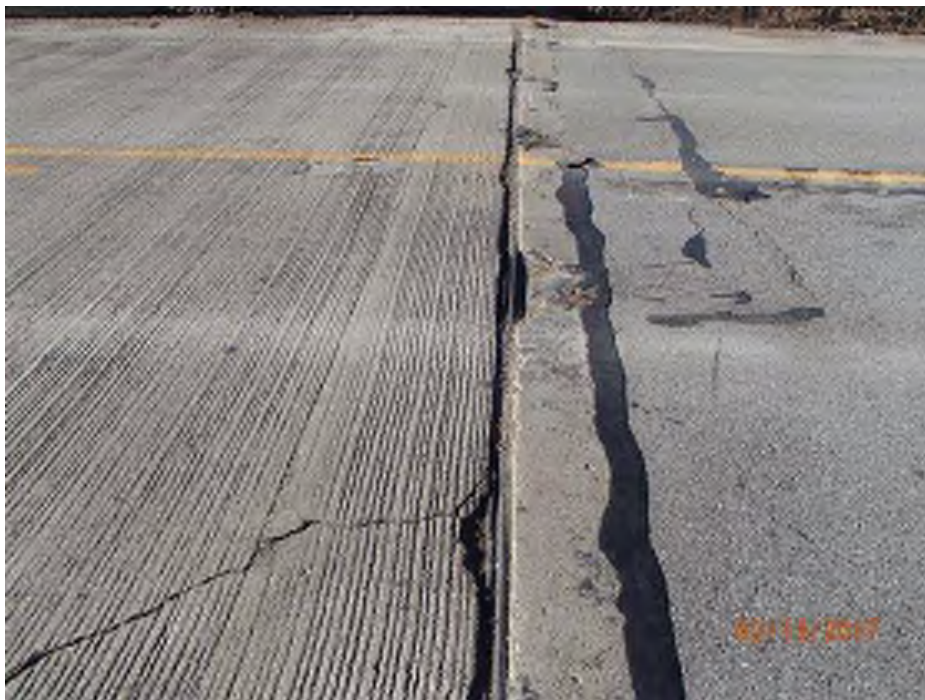
PHOTO 50 Condition Description 02-13-2017 (421)39-12-01792 B Span C wearing surface spalling and cracking at joint and north back wall spalling
