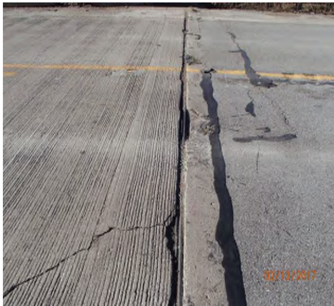
PHOTO 4 Description 02-13-2017 (421)39-12-01792 B Span C wearing surface spalling and cracking at joint and north back wall spalling
