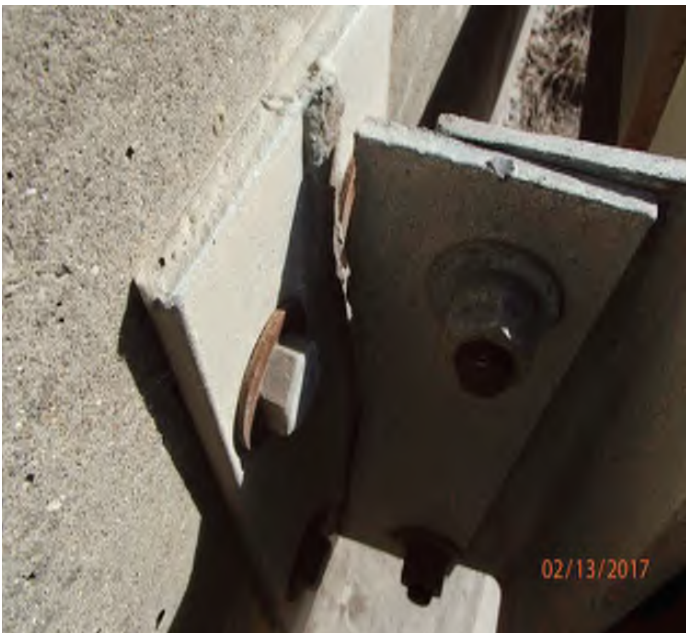
PHOTO 1 Description 02-13-2017 (421)39-12-01792 B Northeast end of guard rail has bracket broke
