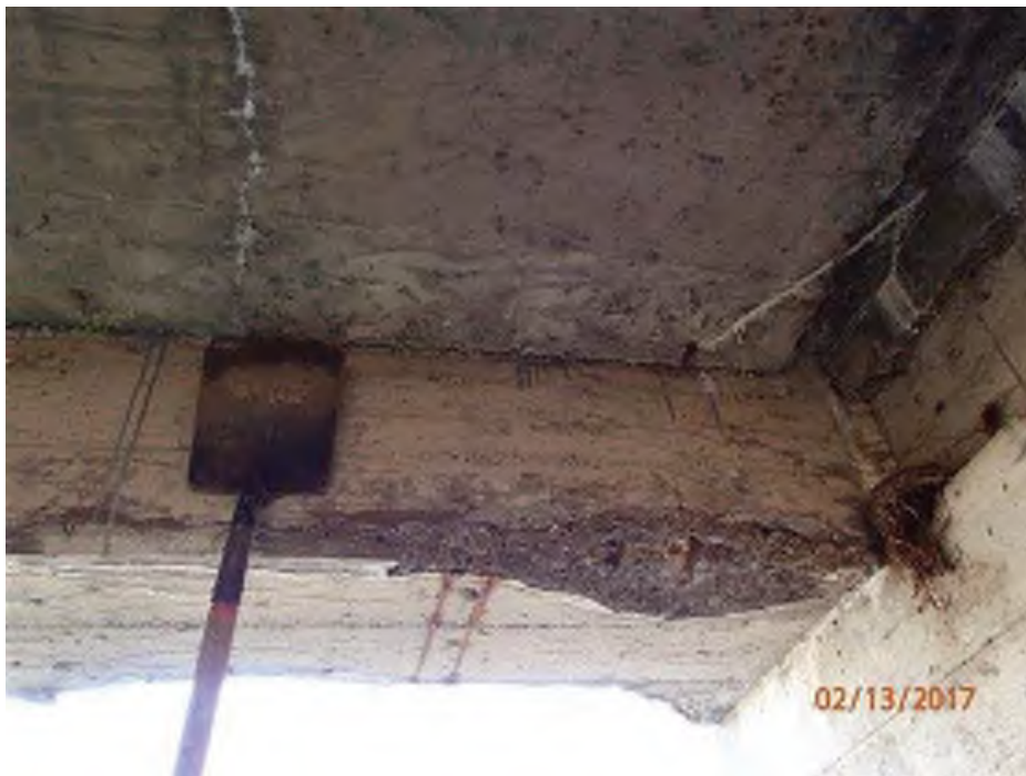
PHOTO 41 Condition Description 02-13-2017 (421)39-12-01792 B Span C beam 5 at pier 3 rebar exposed
