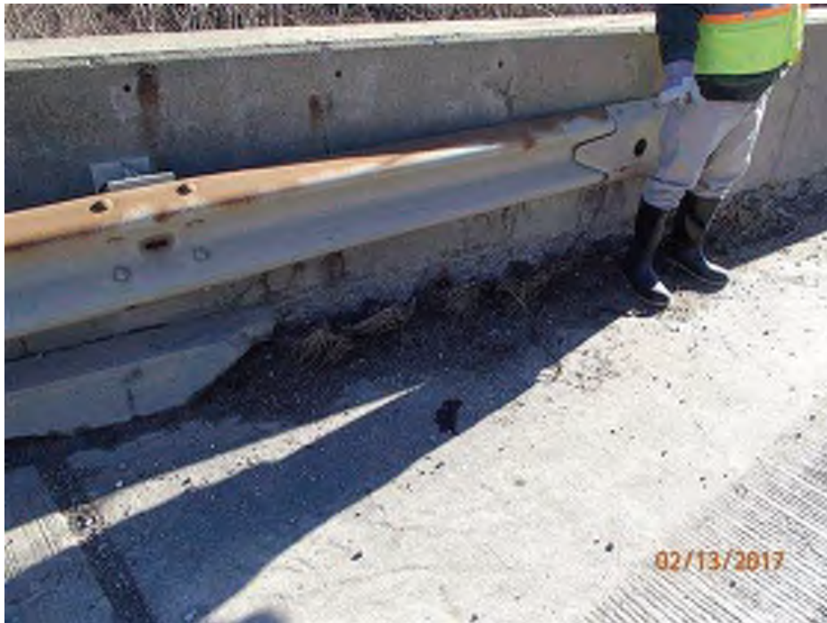
PHOTO 2 Condition Description 02-13-2017 (421)39-12-01792 B Northeast curb spalling
