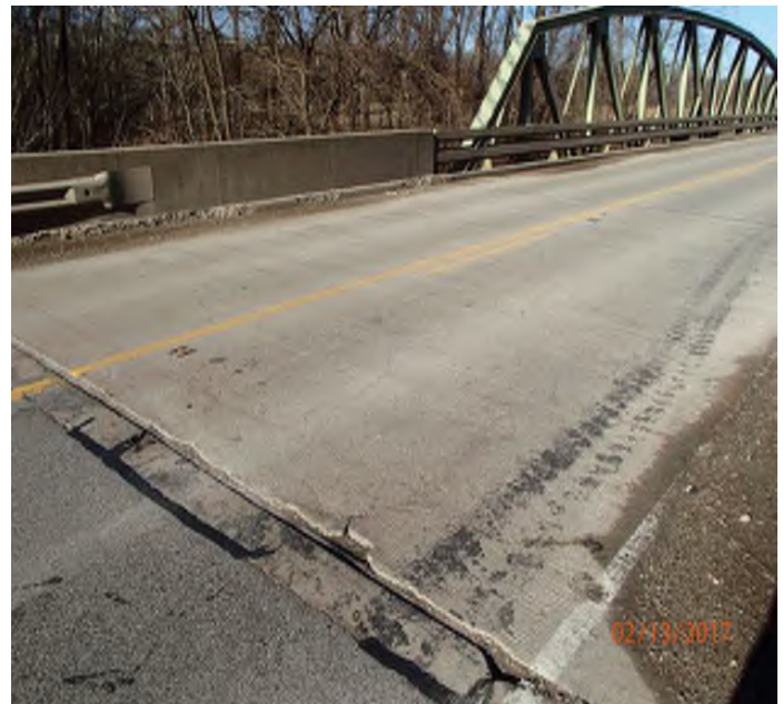
PHOTO 2 Description 02-13-2017 (421)39-12-01792 B South joint and span A deck wearing surface condition
