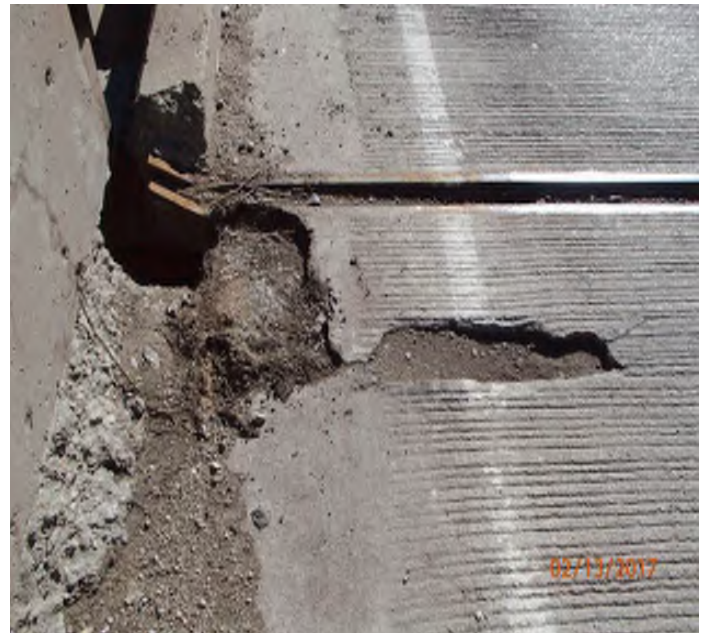
PHOTO 5 Description 02-13-2017 (421)39-12-01792 B Span C wearing surface spalling at joint above pier 3
