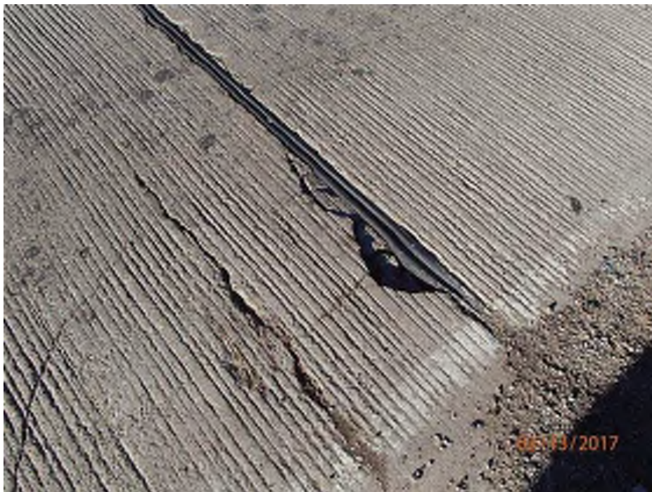
PHOTO 56 Condition Description 02-13-2017 (421)39-12-01792 B Wearing surface spalling at the south interior joint
