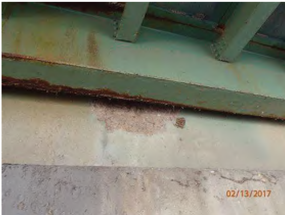
PHOTO 6 Condition Description 02-13-2017 (421)39-12-01792 B Pier 2 north face spalling
