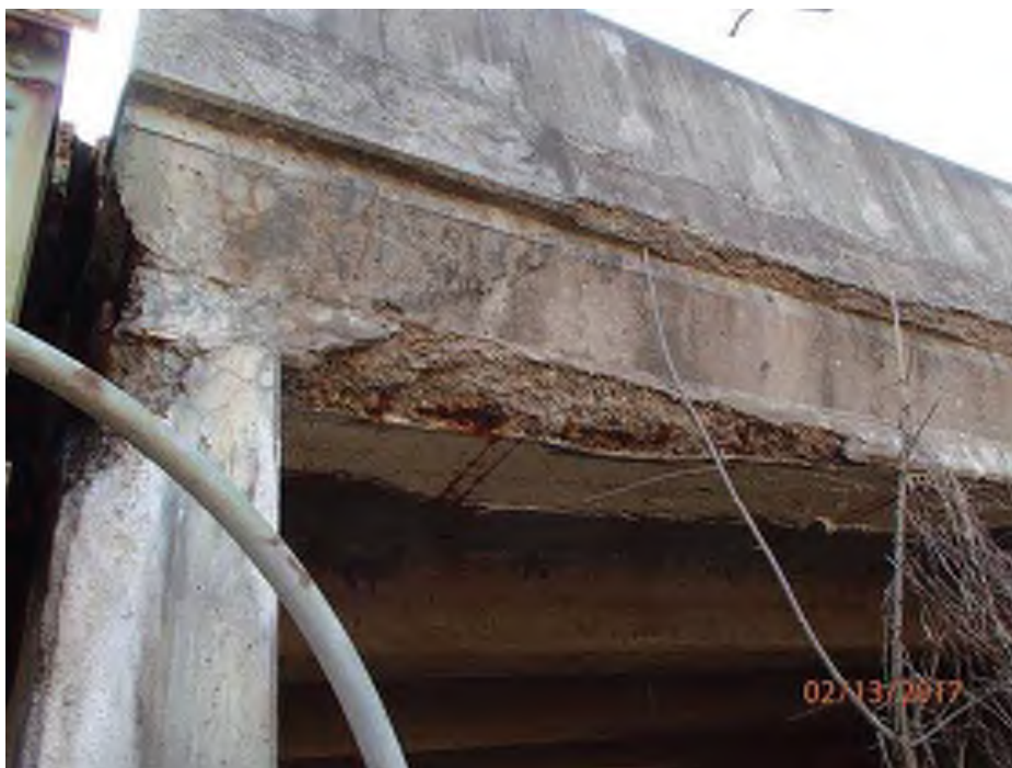
PHOTO 42 Condition Description 02-13-2017 (421)39-12-01792 B Span C beam 5 east side spalling at pier 3
