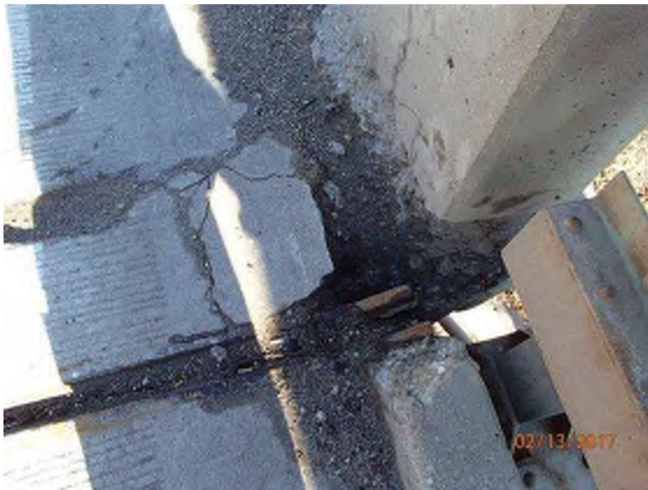
PHOTO 47 Condition Description 02-13-2017 (421)39-12-01792 B Span C deck wearing surface spalled at joint
