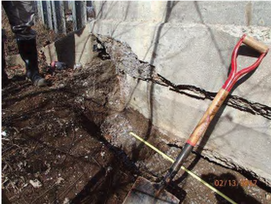
PHOTO 35 Condition Description 02-13-2017 (421)39-12-01792 B Span C beam 1 at the north bent condition
