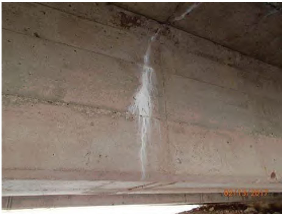
PHOTO 40 Condition Description 02-13-2017 (421)39-12-01792 B Span C beam 3 east side has vertical crack with efflorescence
