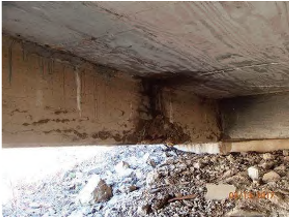
PHOTO 24 Condition Description 02-13-2017 (421)39-12-01792 B Span A beam 5 at the south bent condition
