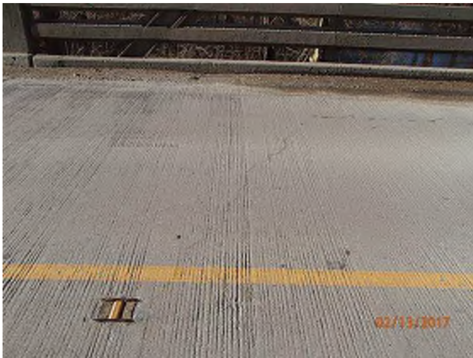
PHOTO 52 Condition Description 02-13-2017 (421)39-12-01792 B Transverse and diagonal cracking in the deck wearing surface
