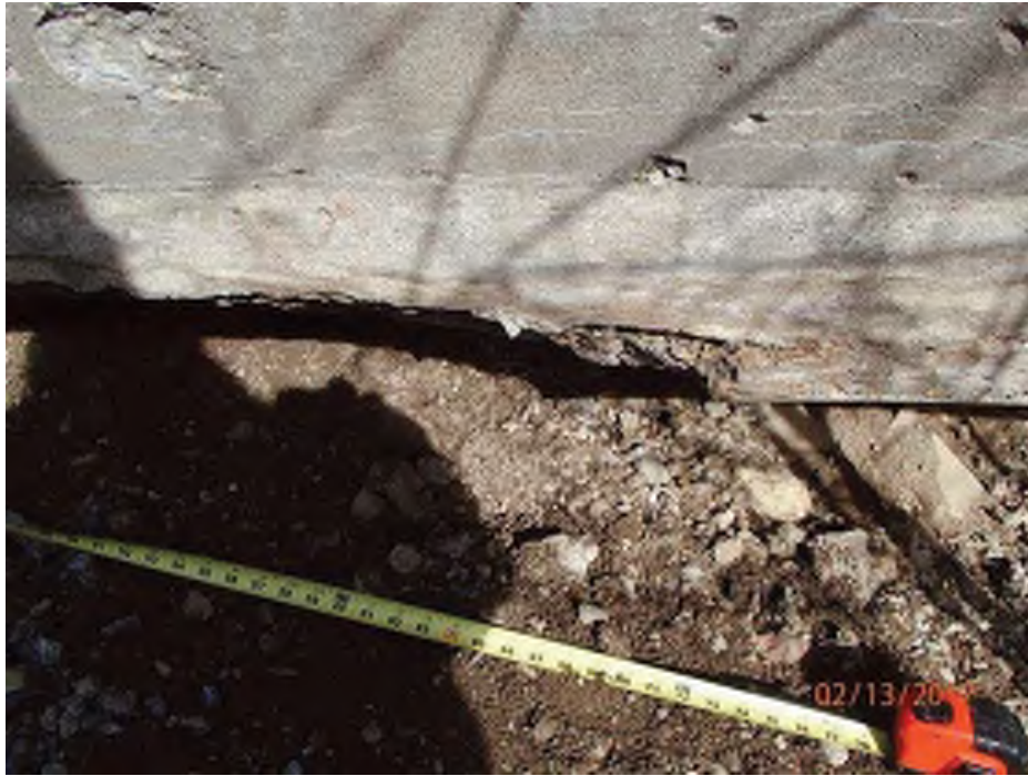
PHOTO 37 Condition Description 02-13-2017 (421)39-12-01792 B Span C beam 1 corner spall measurement
