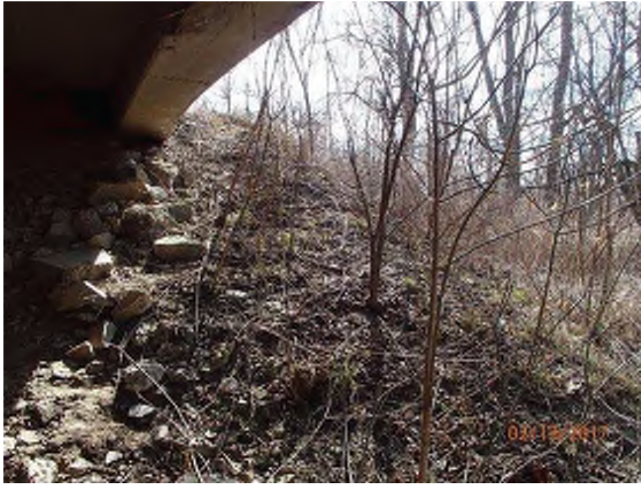
PHOTO 55 Condition Description 02-13-2017 (421)39-12-01792 B Unwanted trees around bridge
