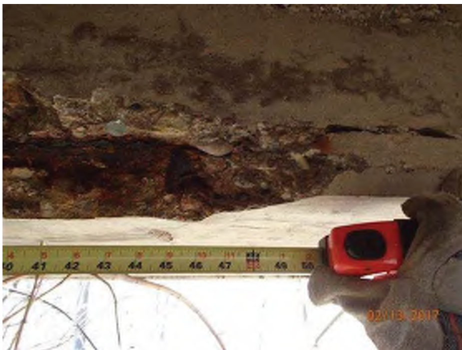
PHOTO 20 Condition Description 02-13-2017 (421)39-12-01792 B Span A beam 1 corner spalled
