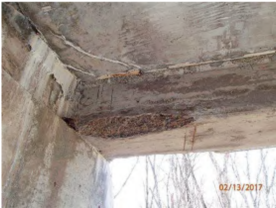
PHOTO 39 Condition Description 02-13-2017 (421)39-12-01792 B Span C beam 1 east face
