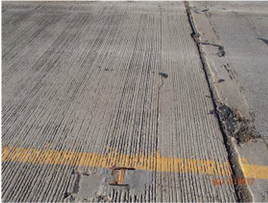
PHOTO 59 Condition Description Span C wearing surface has transverse cracking
