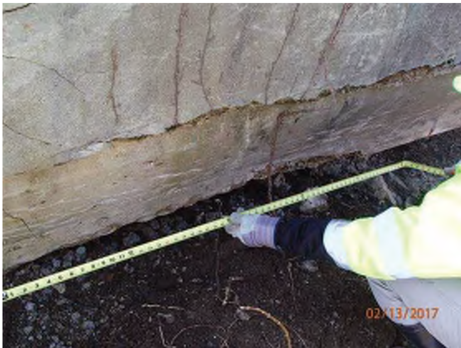
PHOTO 25 Condition Description 02-13-2017 (421)39-12-01792 B Span A beam 5 corner spalling along the east side
