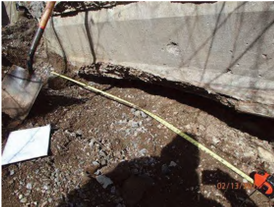
PHOTO 38 Condition Description 02-13-2017 (421)39-12-01792 B Span C beam 1 corner spalling on the west or downstream side
