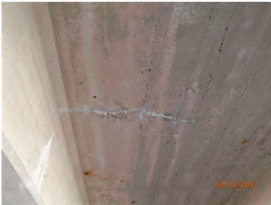
PHOTO 30 Condition Description 02-13-2017 (421)39-12-01792 B Span A deck underside has transverse cracking with efflorescence
