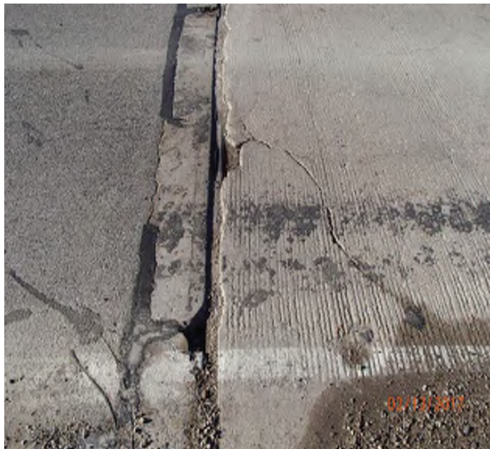
PHOTO 1 Description 02-13-2017 (421)39-12-01792 B South back wall spalling wearing surface cracking and spalling
