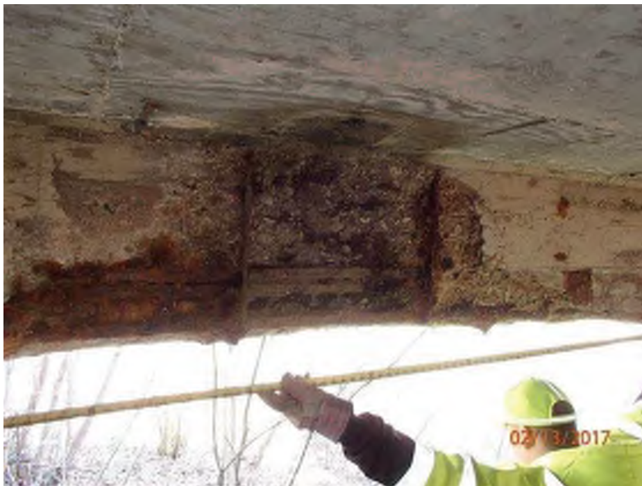
PHOTO 45 Condition Description 02-13-2017 (421)39-12-01792 B Span C beam 5 west side rebar exposed
