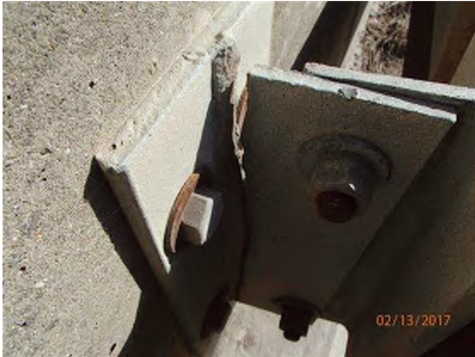
PHOTO 3 Condition Description 02-13-2017 (421)39-12-01792 B Northeast end of guard rail has bracket broke
