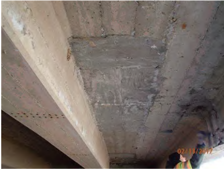
PHOTO 31 Condition Description 02-13-2017 (421)39-12-01792 B Span A full depth patching
