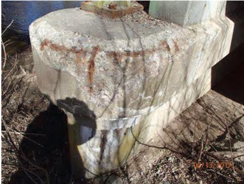
PHOTO 9 Condition Description 02-13-2017 (421)39-12-01792 B Pier 2 west nose spalling
