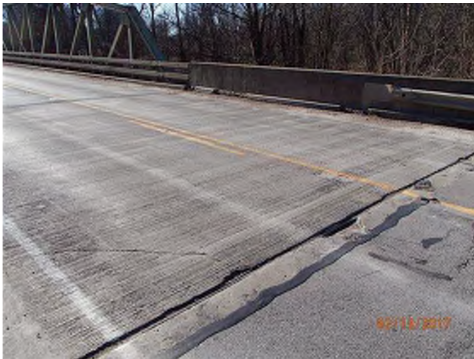
PHOTO 48 Condition Description 02-13-2017 (421)39-12-01792 B Span C wearing surface and north joint condition
