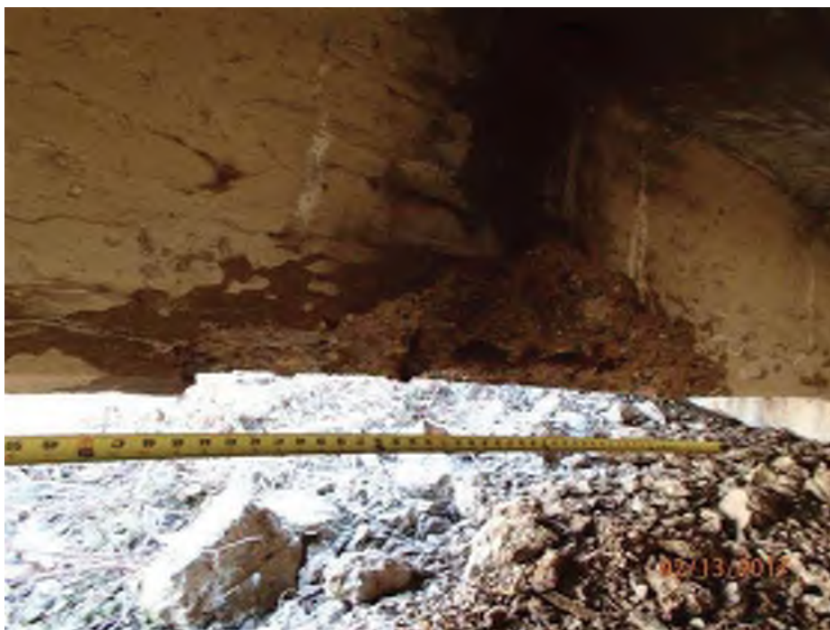
PHOTO 26 Condition Description 02-13-2017 (421)39-12-01792 B Span A beam 5 corner spalling near south bent
