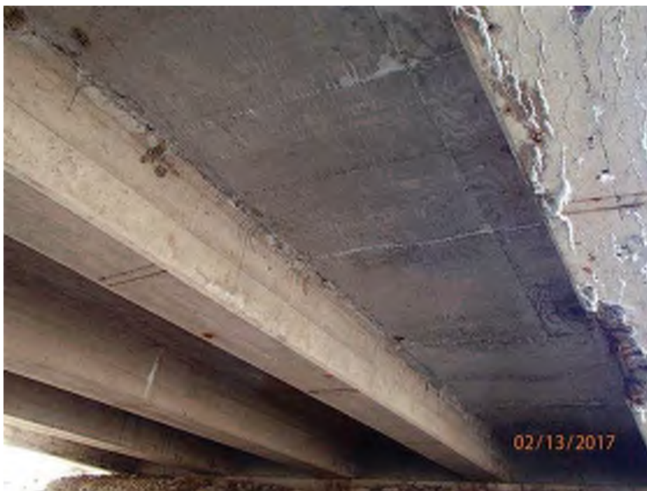
PHOTO 46 Condition Description 02-13-2017 (421)39-12-01792 B Span C deck underside transverse cracking with efflorescence
