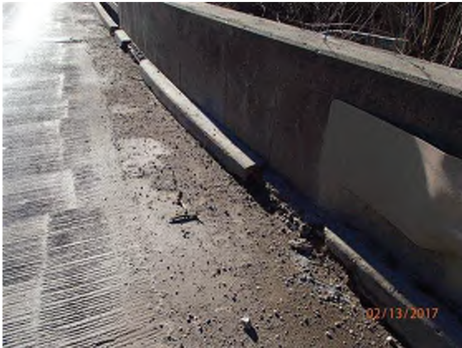
PHOTO 4 Condition Description 02-13-2017 (421)39-12-01792 B Northwest curb spalling
