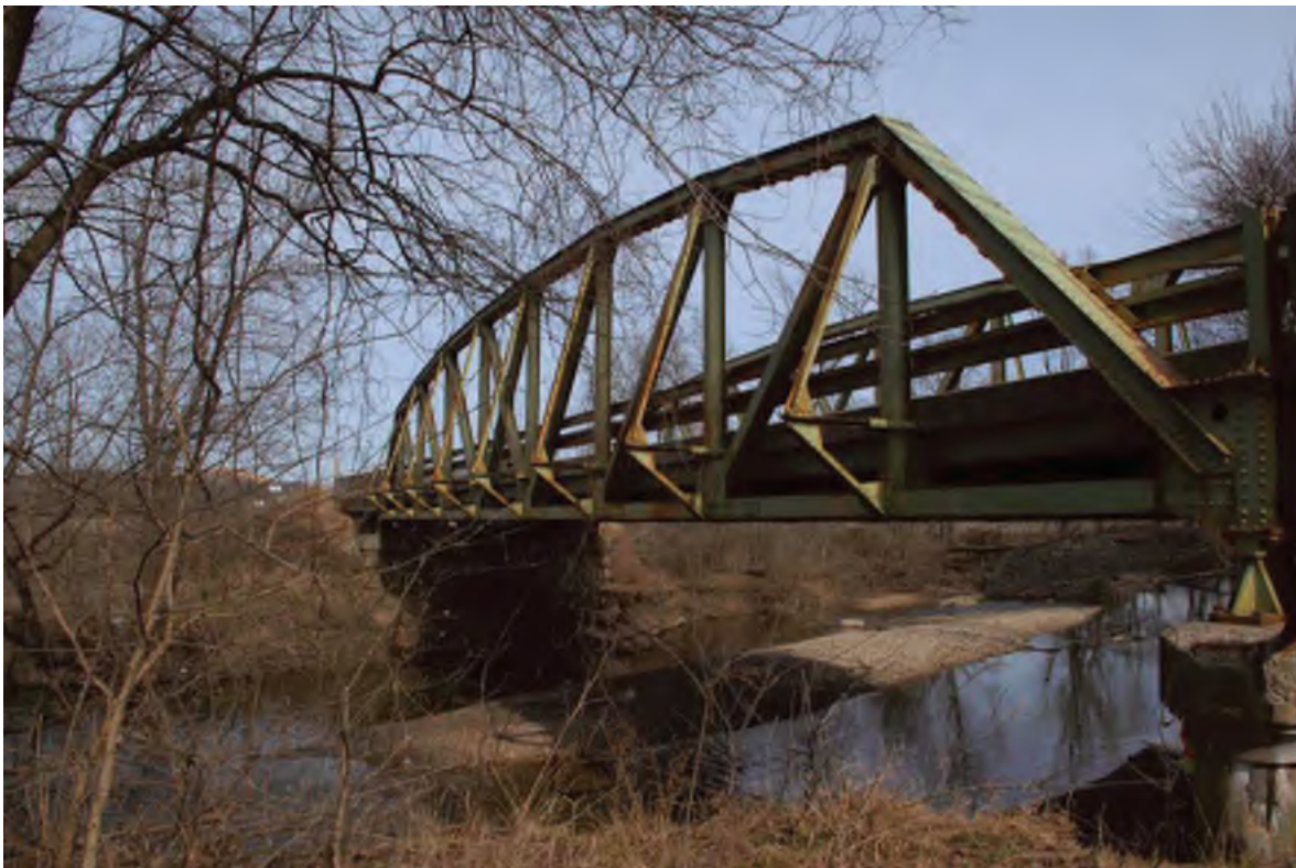
12. The view to the east elevation of the US 421 shows the central truss span
