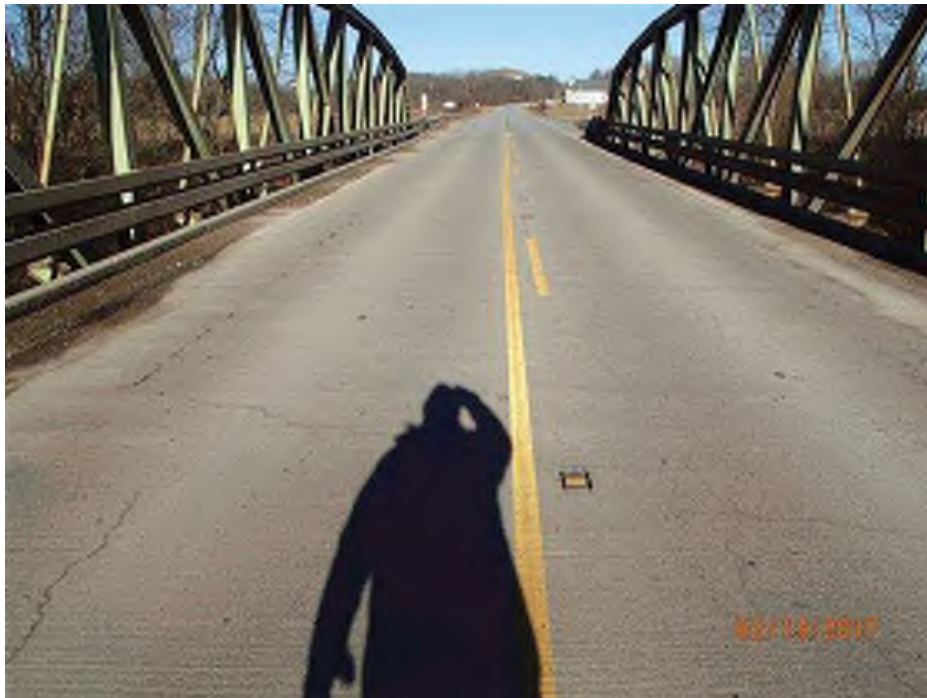
PHOTO 32 Condition Description 02-13-2017 (421)39-12-01792 B Span B deck wearing surface condition looking north
