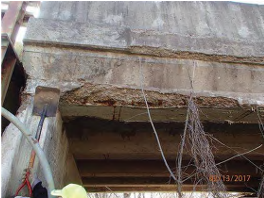
PHOTO 10 Condition Description 02-13-2017 (421)39-12-01792 B Pier 3 east side spalled and beam 5 spalled with rebar exposed
