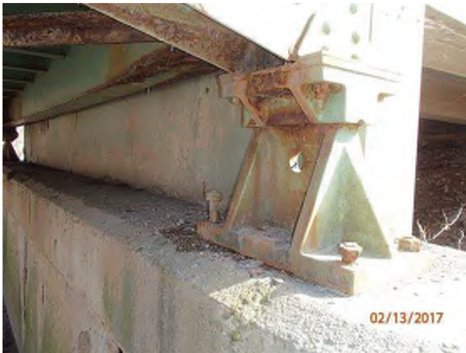
PHOTO 5 Condition Description 02-13-2017 (421)39-12-01792 B Pier 2 Downstream bearing bolts condition
