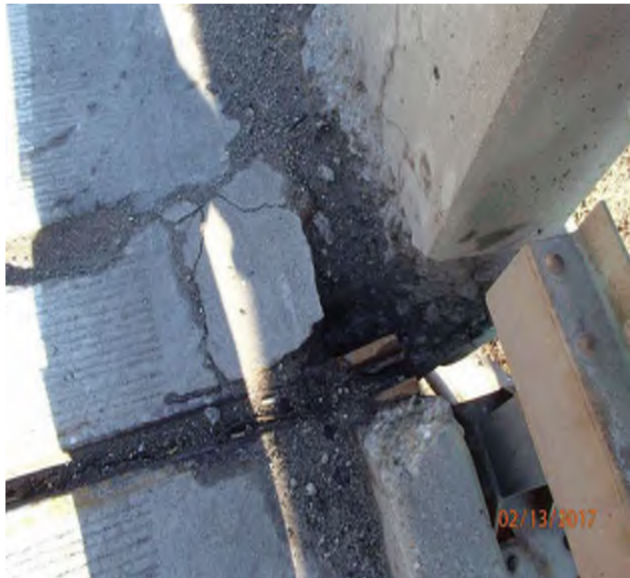
PHOTO 3 Description 02-13-2017 (421)39-12-01792 B Span C deck wearing surface spalled at joint
