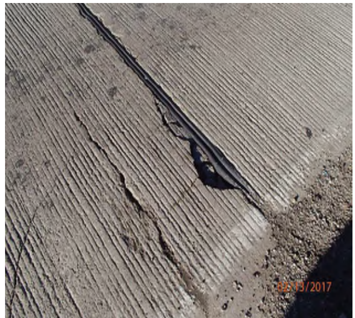
PHOTO 6 Description 02-13-2017 (421)39-12-01792 B Wearing surface spalling at the south interior joint
