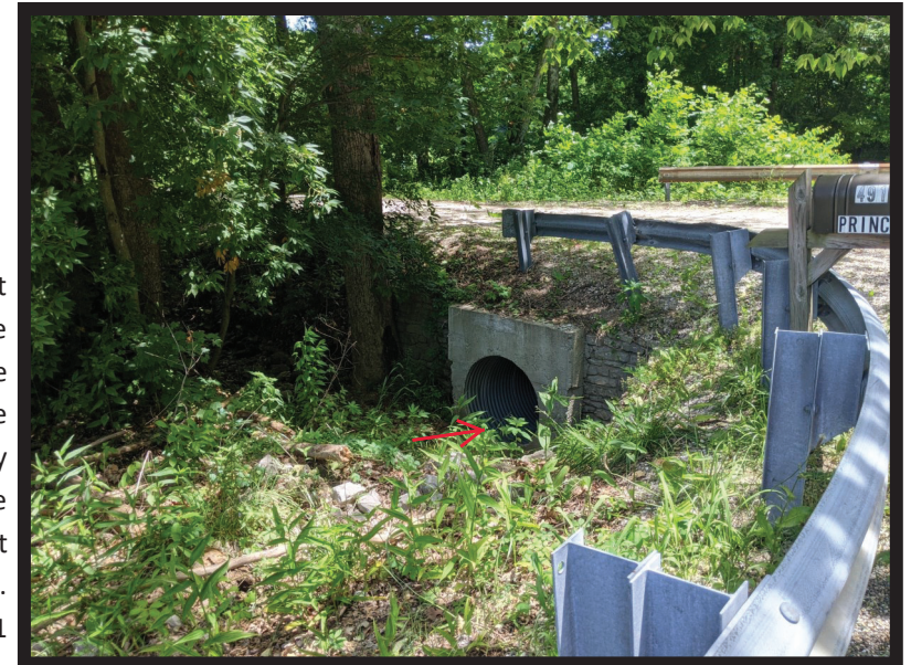
Photo 10. Looking east from SR 158 at the pipe carrying UNT Silverville Branch beneath a private drive before immediately discharging into Silverville Branch in the northwest quadrant of the bridge. 6/14/2021
