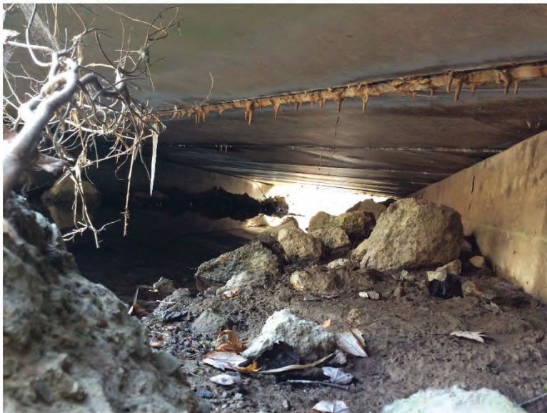
PHOTO 5 Condition Description Underside facing Southeast
