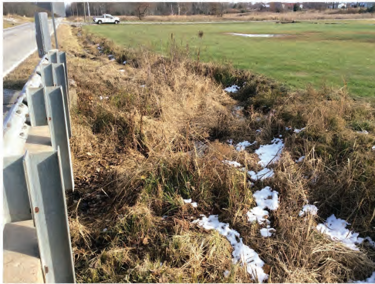
PHOTO 6 Condition Description S channel, facing e
