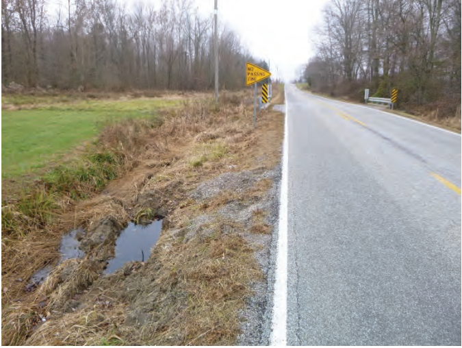
TYPICAL CONDITION OF SHOULDER AT SOUTHEAST CORNER OF STRUCTURE
