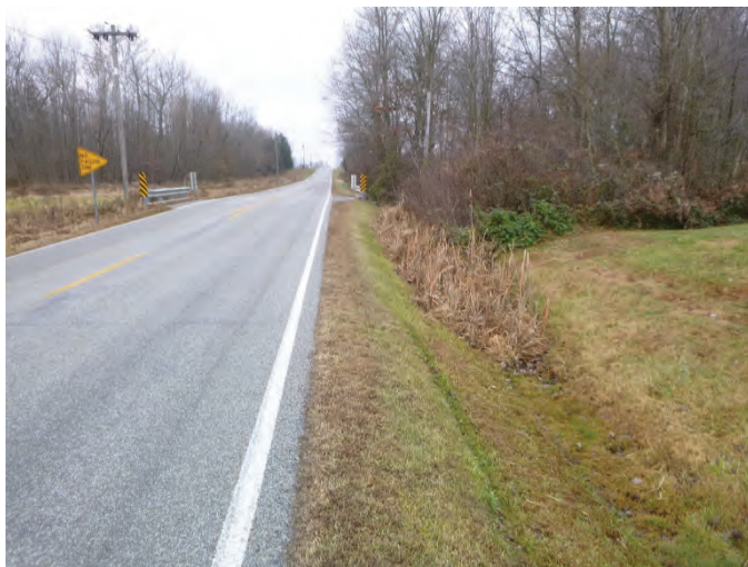
TYPICAL CONDITION OF SHOULDER AT NORTHEAST CORNER OF STRUCTURE
