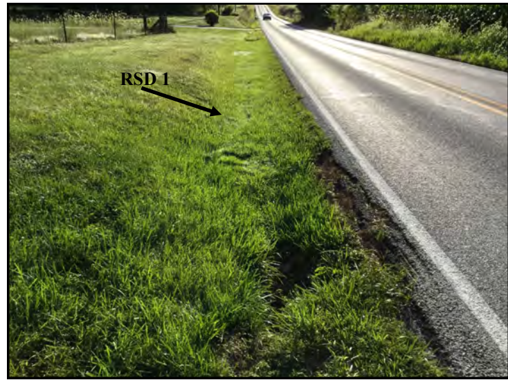
38. View of Roadside Ditch (RSD) 1 and S.R. 58 ROW from western PSL, looking northeast.
