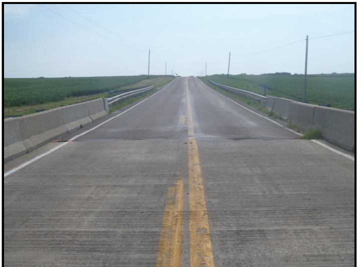
Photo 12 – Greenwood Ditch Bridge: Facing west along SR 18 from top of subject bridge that crosses Greenwood Ditch. Total bridge width to be widened by approximately six feet.
