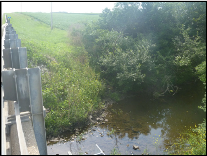
Photo 15 – Greenwood Ditch Crossing: Facing southeast quadrant of bridge and outfall of roadside ditch. Wingwalls and riprap to be installed. Wetland determination point along woods was non-wetland.
