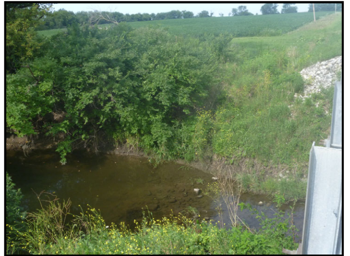
Photo 16 – Greenwood Ditch Crossing: Facing southwest quadrant of bridge and outfall of roadside ditch. Wingwalls and riprap to be installed. Per aeriels, woodlands were recently reduced and overhead utilities installed.
