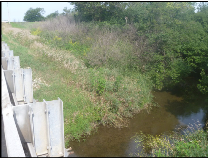
Photo 13 – Greenwood Ditch Crossing: Facing northwest quadrant of bridge and outfall of roadside ditch. Wingwalls and riprap to be installed. Wetland determination point along woods beyond ditch was non-wetland.
