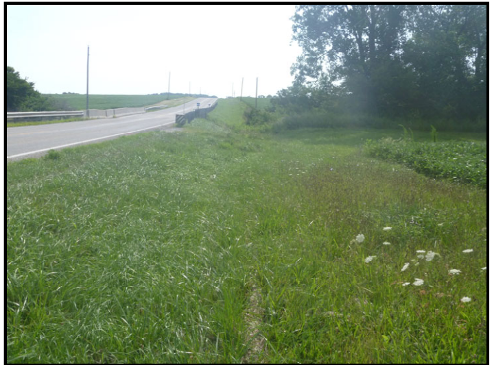
Photo 10 – Southwest Quadrant: Facing east along poorly defined roadside ditch and field access in southwest quadrant. Plans propose installing short ditch beneath field access, extending guardrail, and moving out right-of-way.
