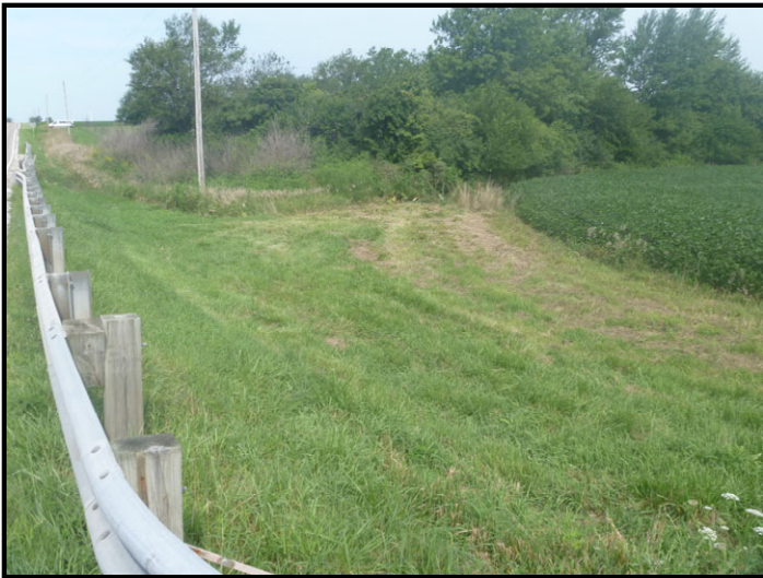
Photo 21 – Northeast Roadside Ditch: At field entrance, facing northwest toward poorly defined roadside ditch in northeast quadrant of project area. Plans propose relocating ditch away from the road.
