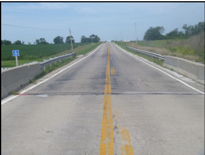
Photo 11 – Greenwood Ditch Bridge: Facing east along SR 18 from top of subject bridge that crosses Greenwood Ditch. The proposed preferred alternative is to replace the bridge with a 34-foot span 3-sided box culvert.
