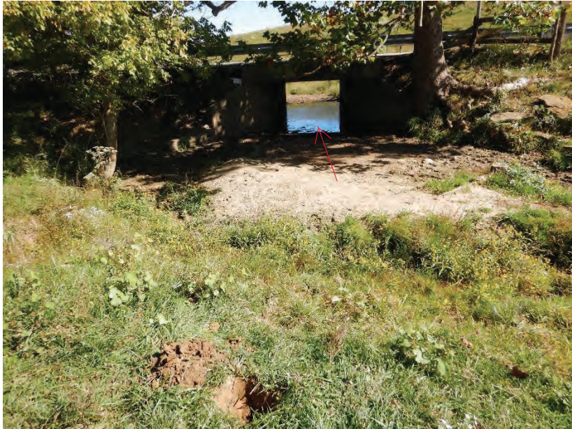
Photo 4: SP 1, on Westside of CV 056-058-187.65, Facing East Towards CV 056-058-187.65 Carrying Buck Run
