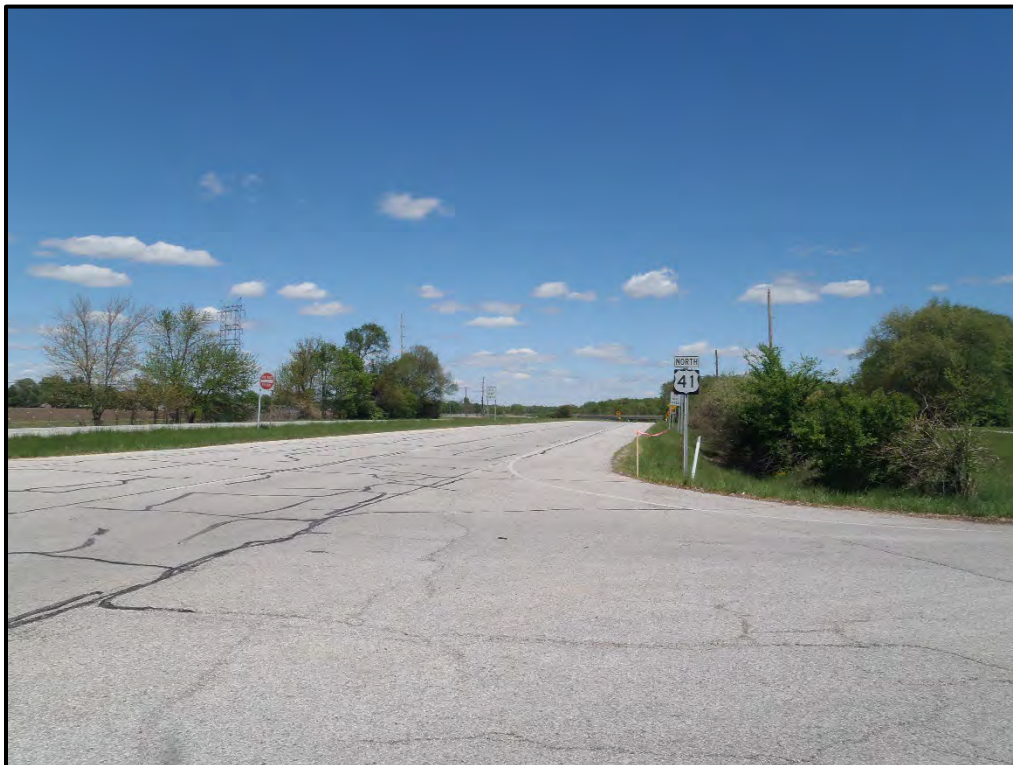
Photo 10: Looking north towards the bridge from the intersection of Budd and US 41 (5-5-21).
