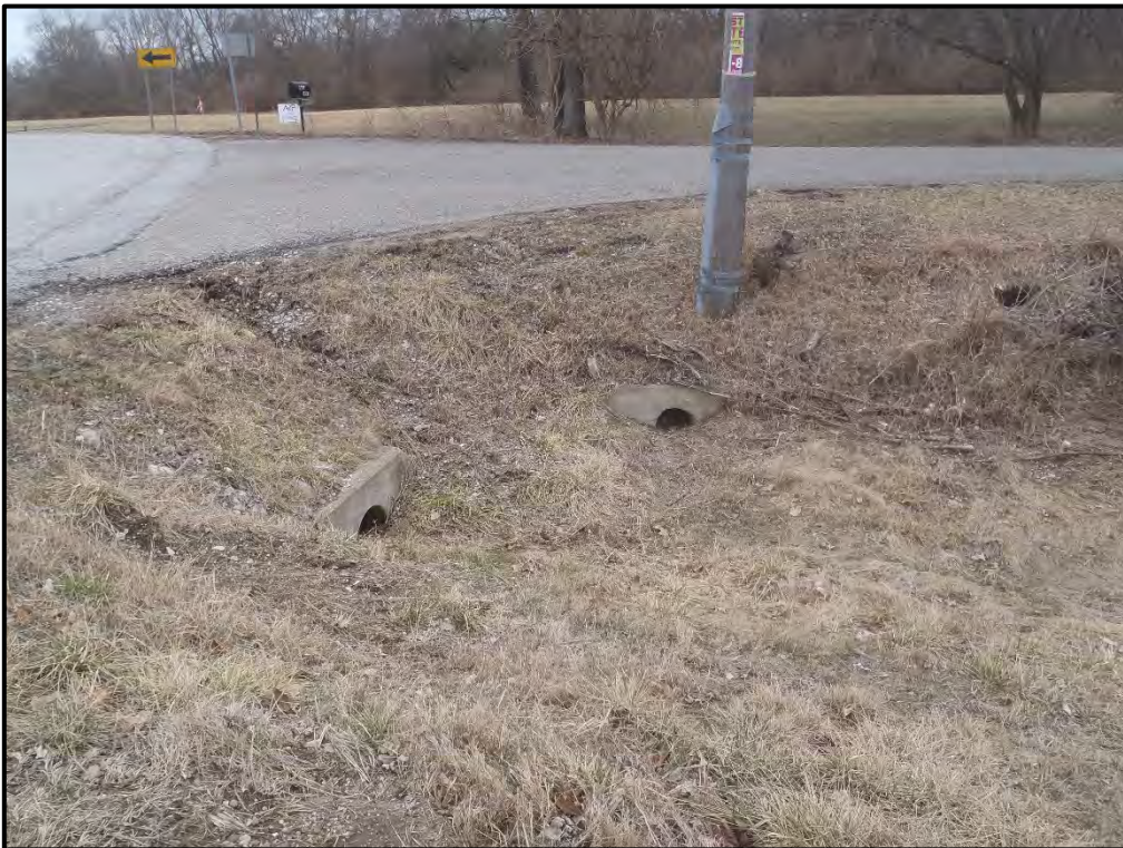
Photo 24: Overflow structures at Budd Street and US 41 NBL on the south side of Budd Street (3-8-22).
