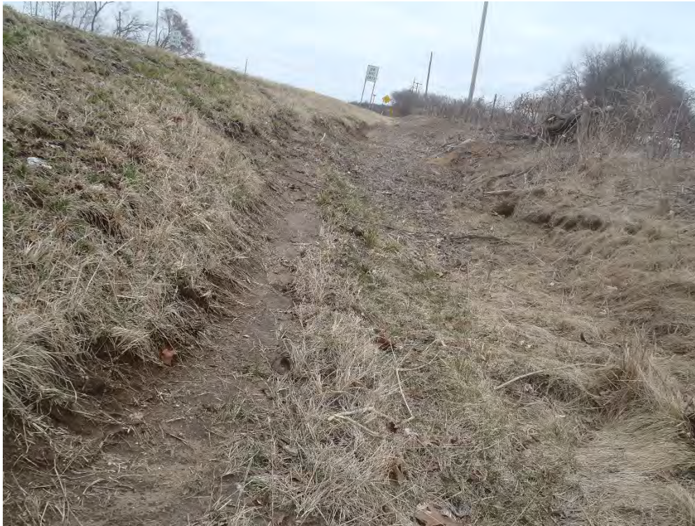
Photo 27: Looking at, what at first appeared to be an Ordinary Highwater Mark (OHWM) but was determined to be a slump or where someone had run off the road in the past. This is not an OHWM in the grassy swale on the north side of US 41 NBL from the Budd Street intersection (3-8-22).
