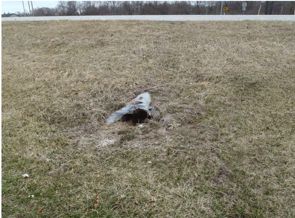
Photo 36: The overflow structure on the north side of the intersection of Quinn Avenue and US 41 SBL (3-8-22).
