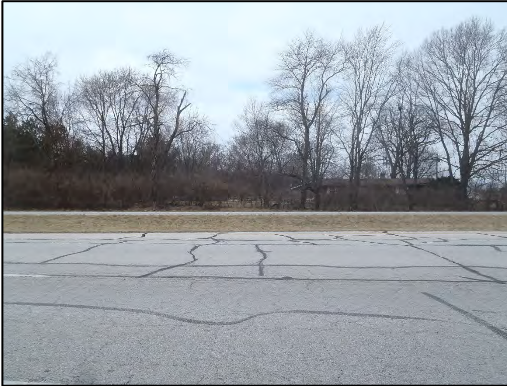
Photo 21: Looking west from the south end of the new investigated area area on the NBL of US 41 (3-8-22)
