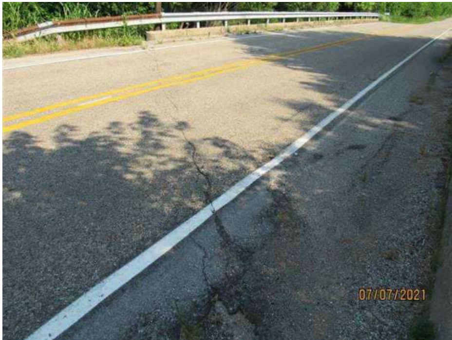
PHOTO 6 Description South Joint Cracking
