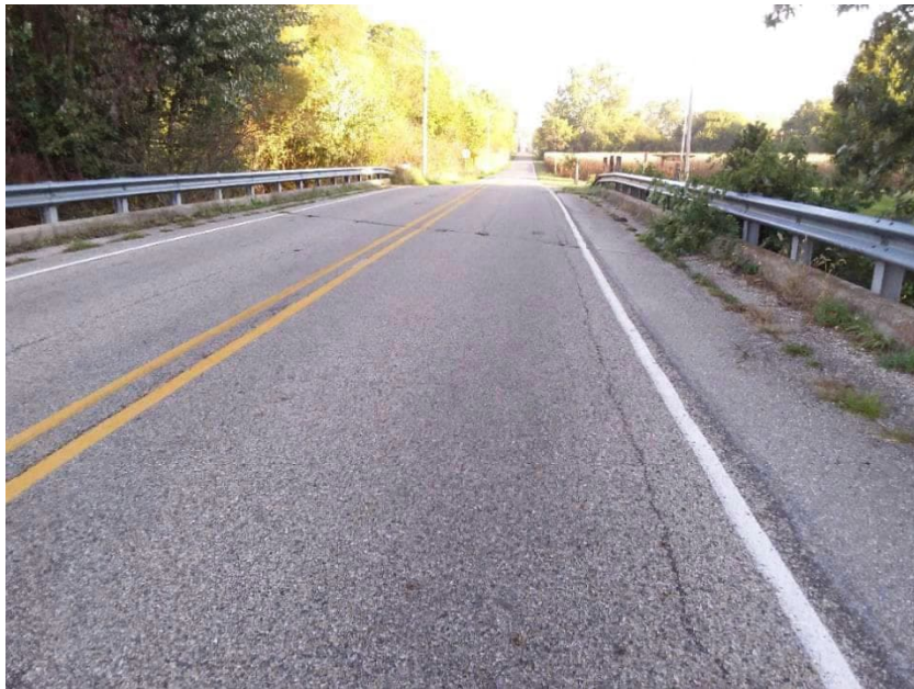
PP-2; Looking north at Johnson County Bridge 98 at the E. Urmeyville Rd and CR 700 E intersection
