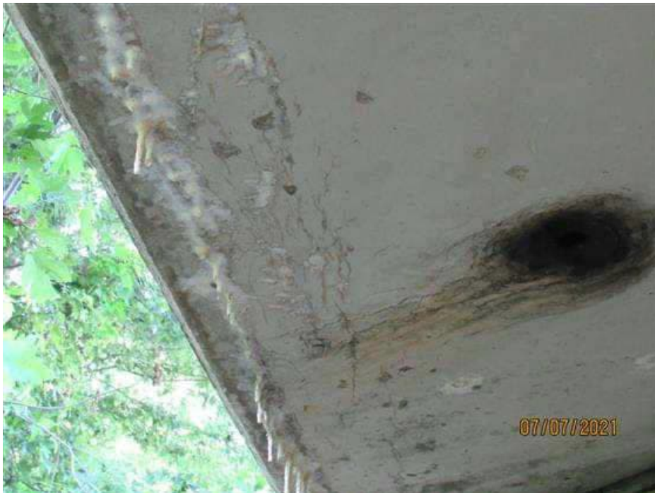
PHOTO 14 Description Cracking With Leaching in Beam 8B
