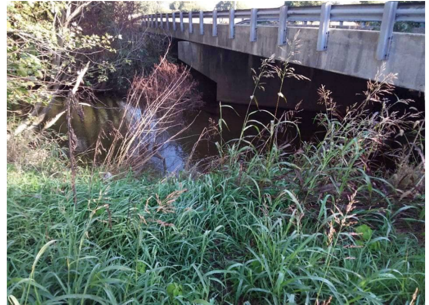
PP-3; Looking north at Johnson County Bridge 98 from the southern bank of Little Sugar Creek west of the bridge (2021-10-20)
