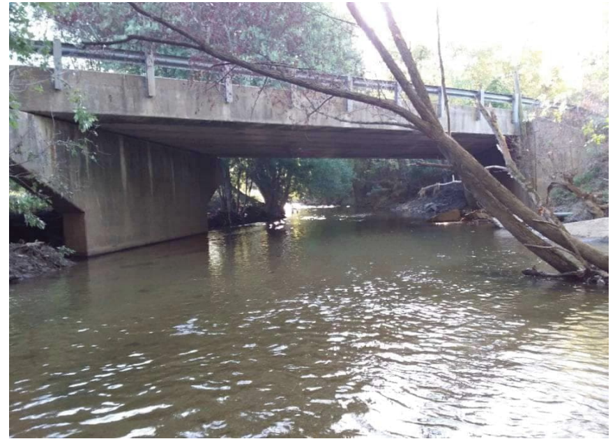
PP-4; Looking east, downstream, at Johnson County Bridge 98 from Little Sugar Creek
