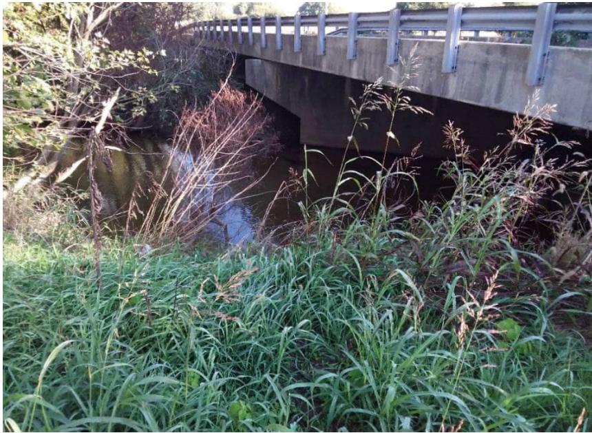
PP-3; Looking north at Johnson County Bridge 98 from the southern bank of Little Sugar Creek west of the bridge.
