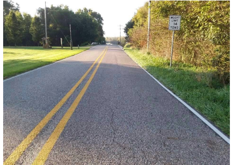
PP-7; Looking south toward Johnson County Bridge 98 from the northern portion of the project area
