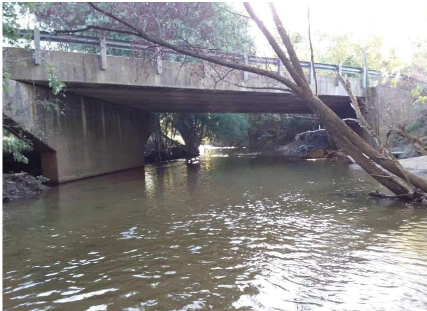
PP-4; Looking east, downstream, at Johnson County Bridge 98 from Little Sugar Creek (2021-10-20)
