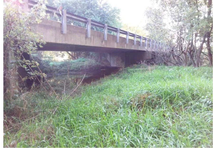
PP-7; Looking southeast at Johnson County Bridge 98 from Little Sugar Creek from the north side of Little Sugar Creek (2021-10-20)
