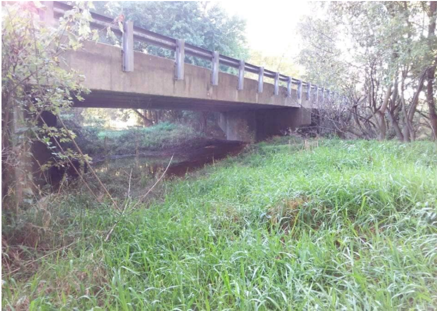
PP-6; Looking southeast at Johnson County Bridge 98 from Little Sugar Creek from the north side of Little Sugar Creek
