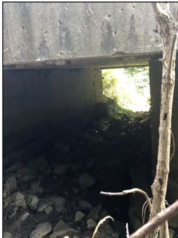
Photo 6: Underside of the culvert taken from the northwest side of culvert. There is no stream running under the culvert. Soil is saturated but no surface water is present.
