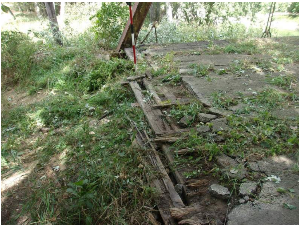
Photo 34: Deterioration on West end of Deck
