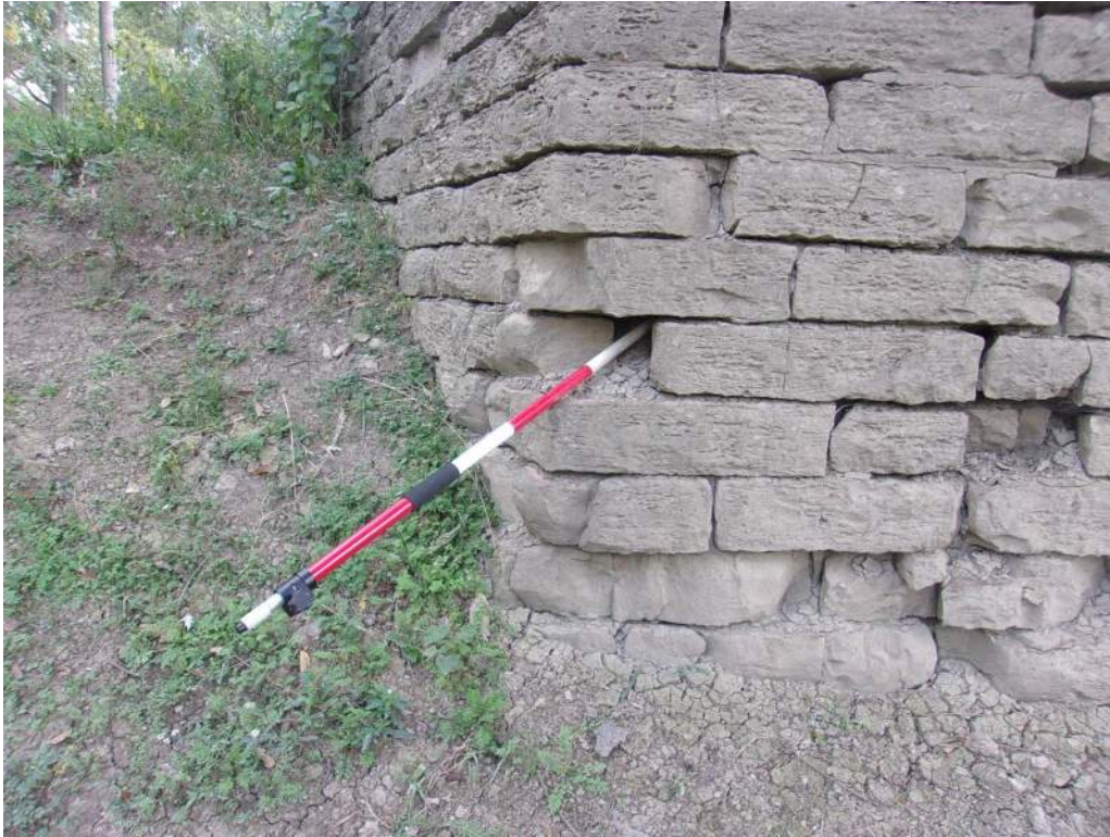
Photo 1: Missing Masonry Block; Section Loss on East Abutment, North Corner
