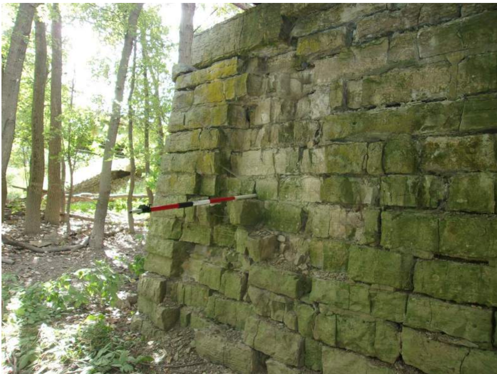
Photo 36: Masonry Block Section Loss on West Abutment
