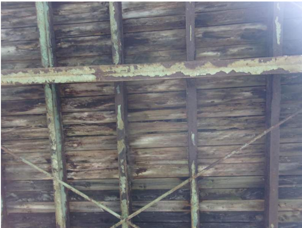
Photo 2: Timber Section Loss on underside of decking
