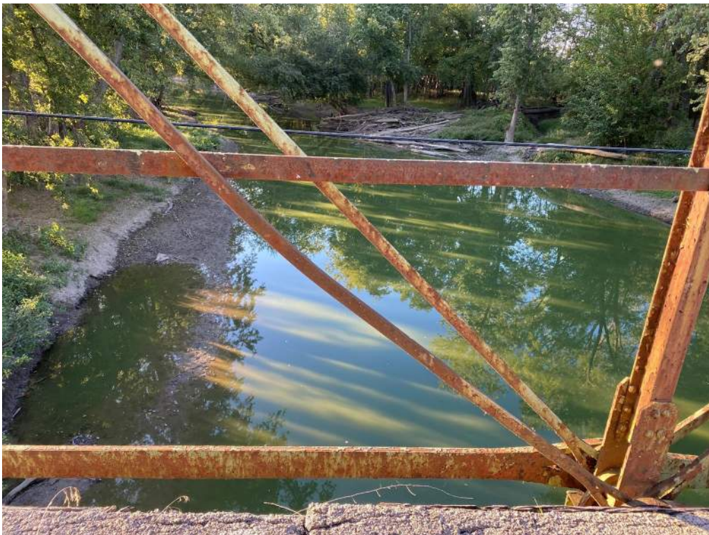
Photo 28: Out-of-Plane Distortion of U4-L6 near L6, North Truss
