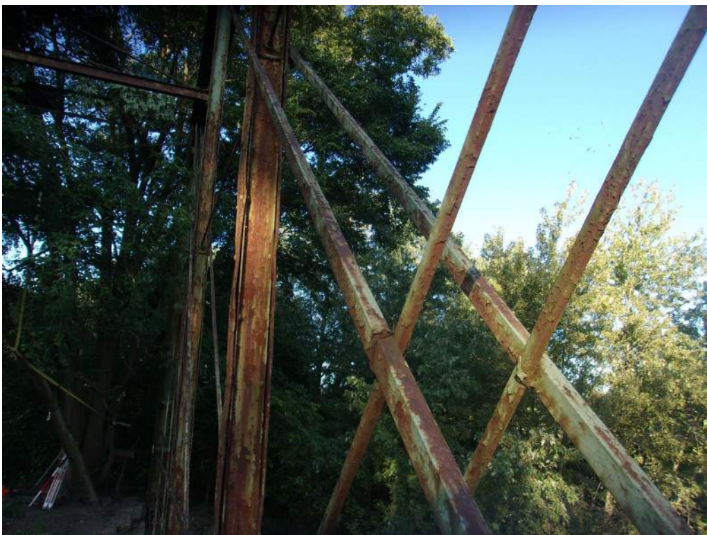
Photo 16: Typical Peeling Paint on Diagonals, South Truss
