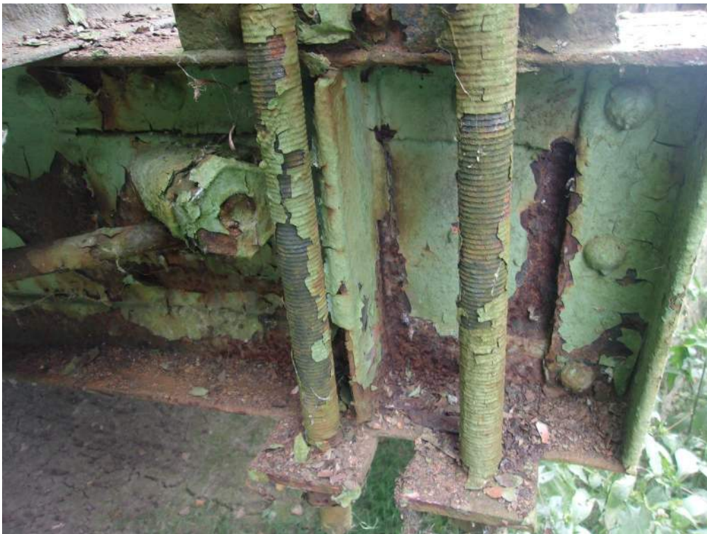
Photo 8: Section Loss on Floor Beam at L1, North Truss
