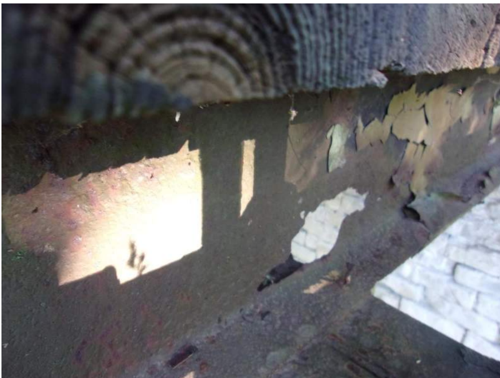
Photo 20: Hole in Stringer 1 near L11, South Truss
