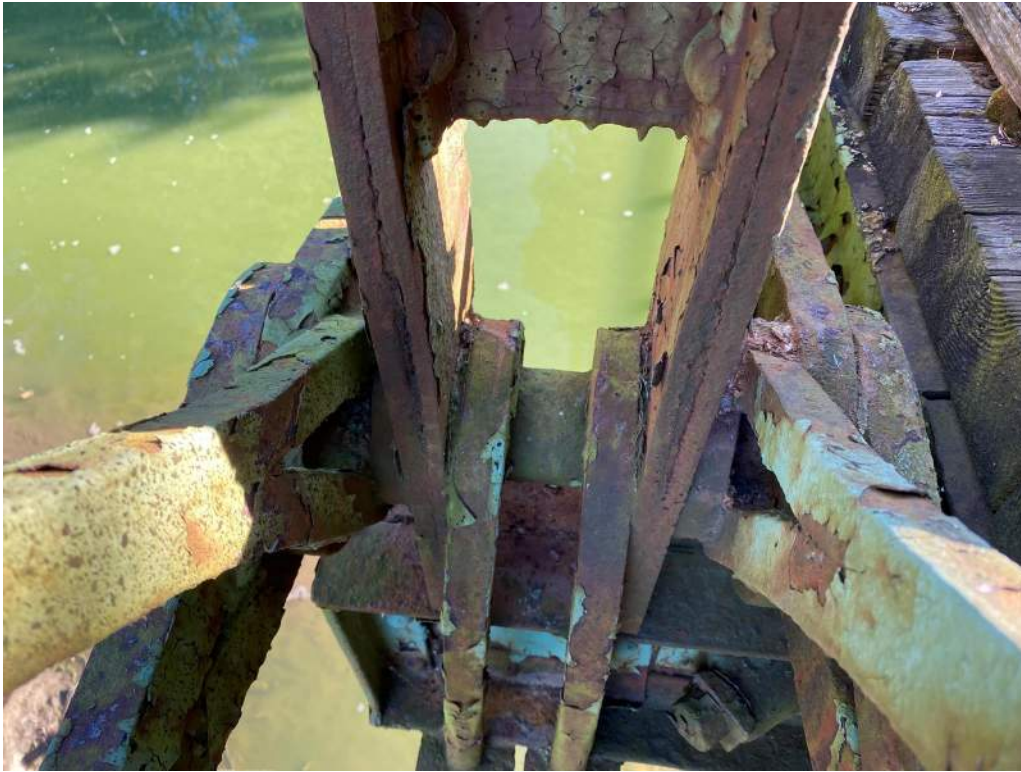
Photo 27: Pack Rust Between Plates and Heavy Rust at L4, North Truss
