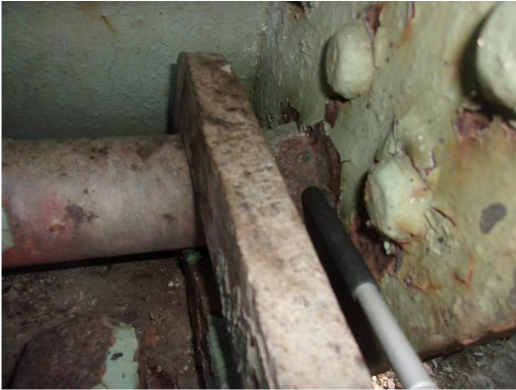
Photo 21: Section Loss on Pin at L12, South Truss
