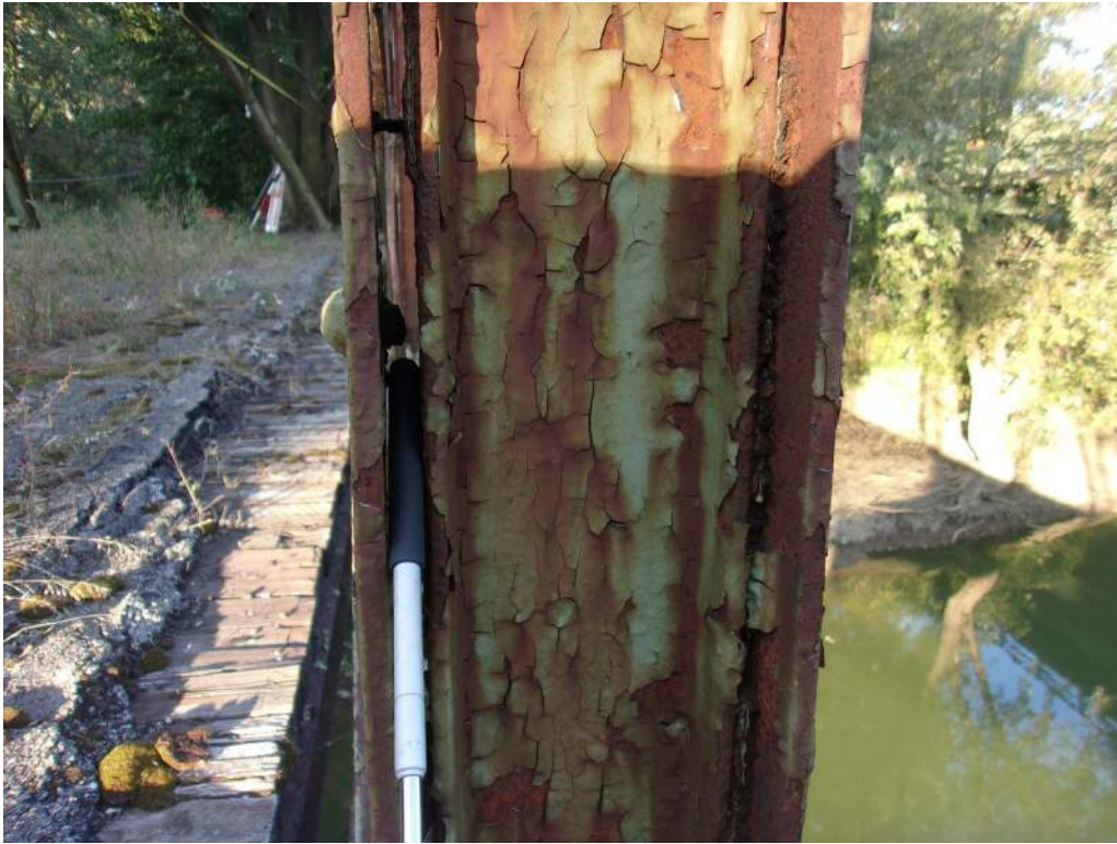
Photo 15: Broken Rivets at Pack Rust at L8-U8 at L8, South Truss
