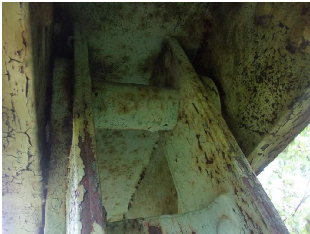
Photo 38: Typical Inside Condition on Upper Connections
