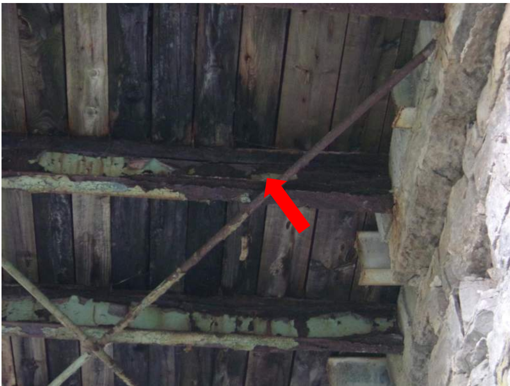
Photo 4: Hole in Stringer 3 Web, East Abutment
