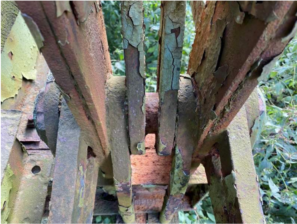
Photo 23: Surface Rust and Pitting with Section Loss on L2 Pin, North Truss
