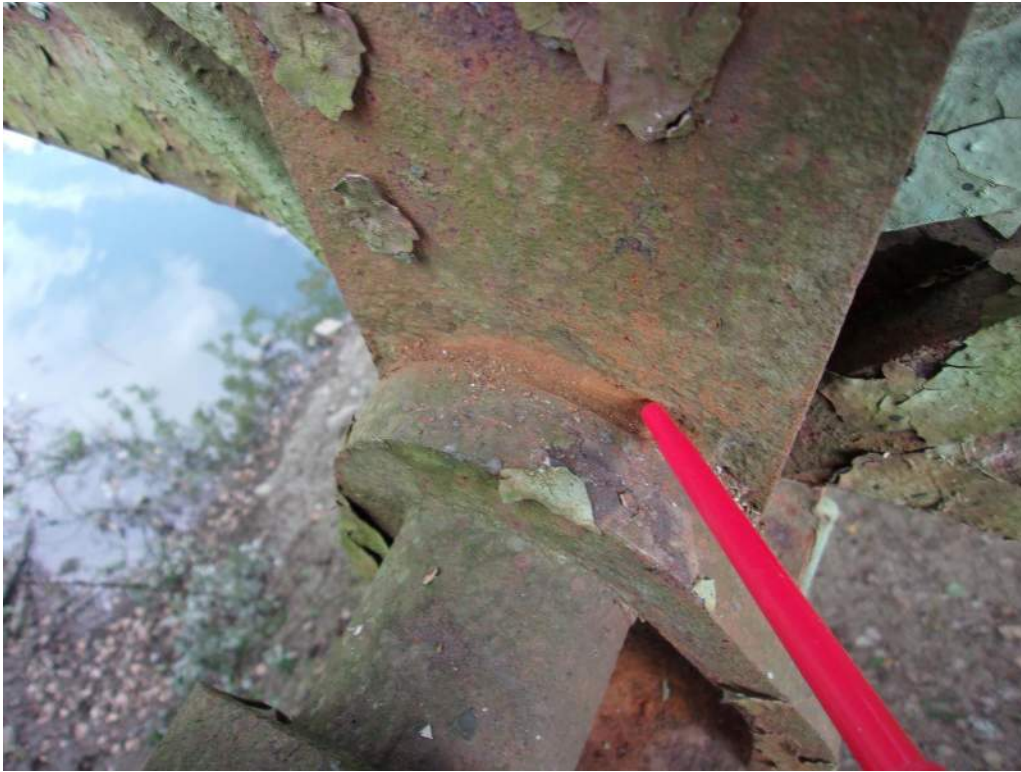
Photo 9: Pack Rust and Section Loss on L3-U3 at Threaded Rod at L3, South Truss
