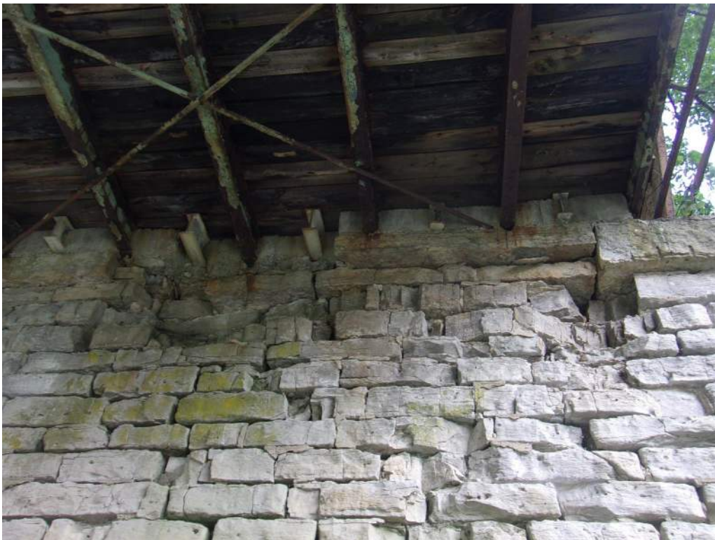
Photo 6: Section Loss of Masonry Blocks at East Abutment
