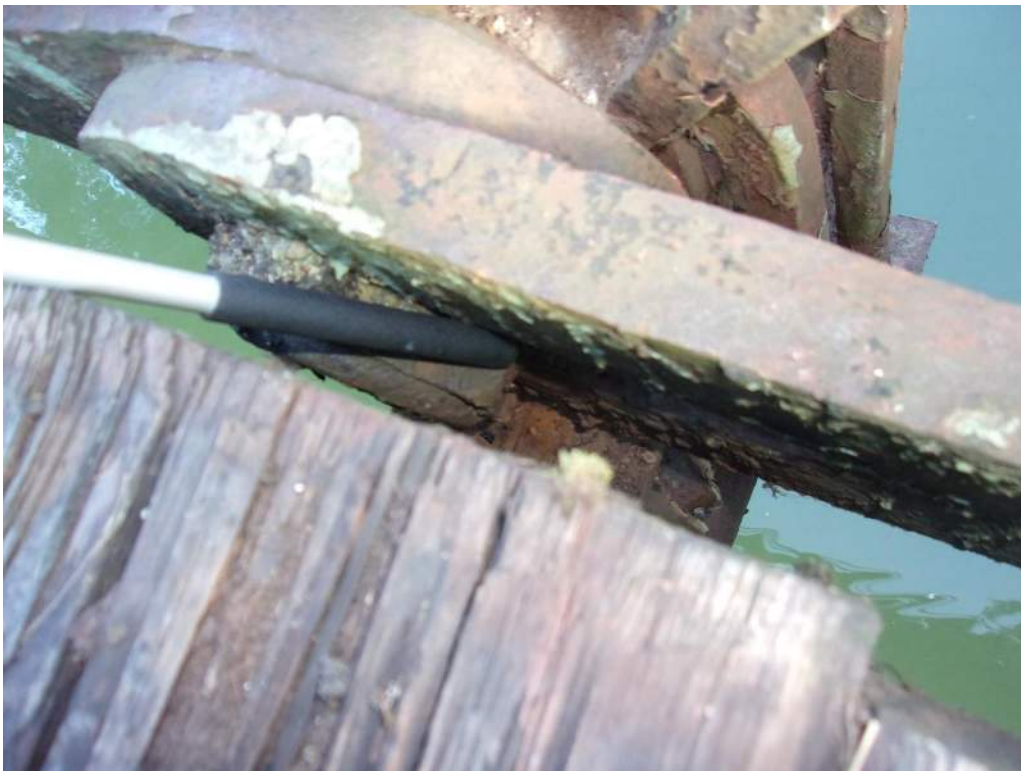
Photo 14: Section Loss on Interior nut and Pin at L6, South Truss
