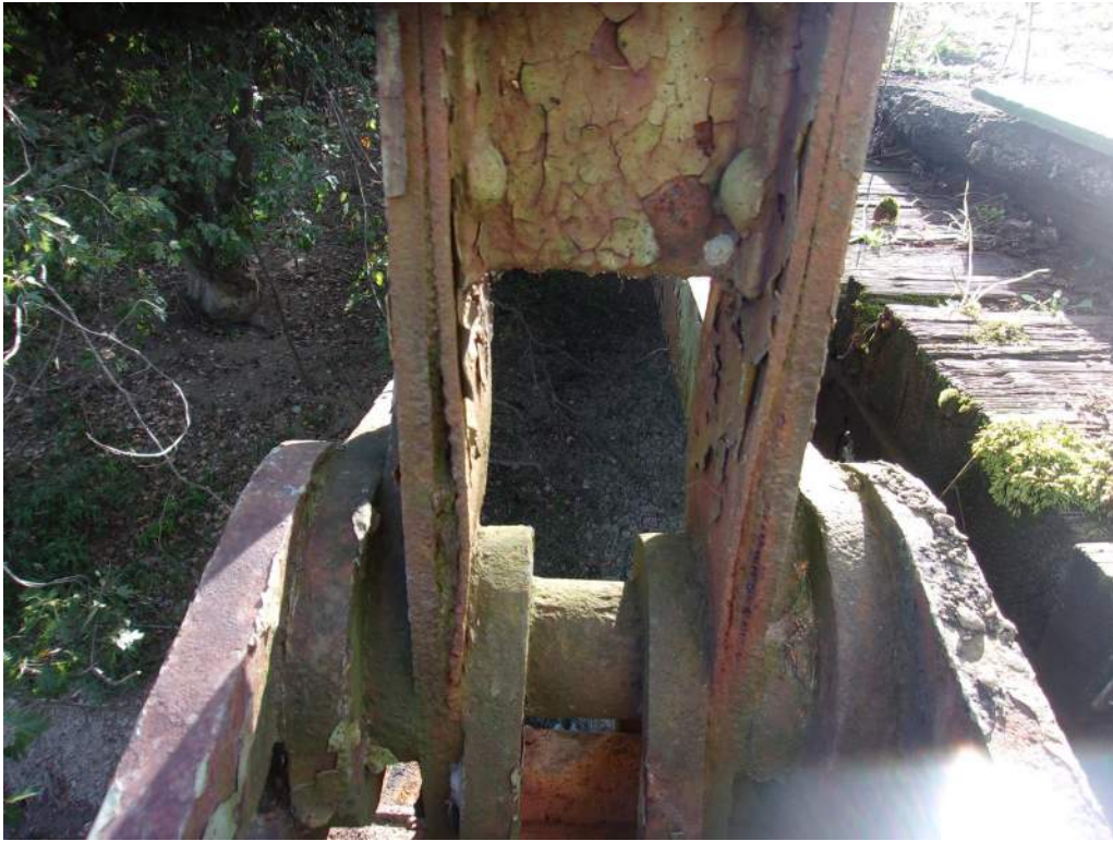
Photo 13: Out-of-Plane Distortion and Pack Rust at L5-U5 at L5, South Truss
