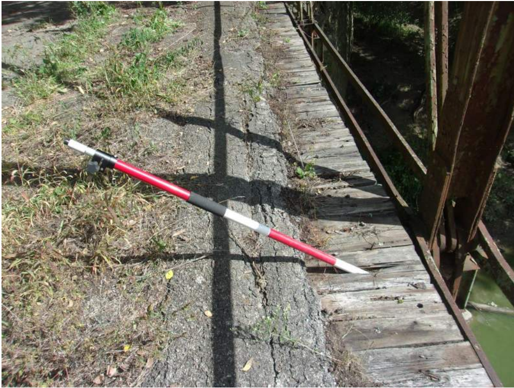
Photo 5: Damage in timber decking
