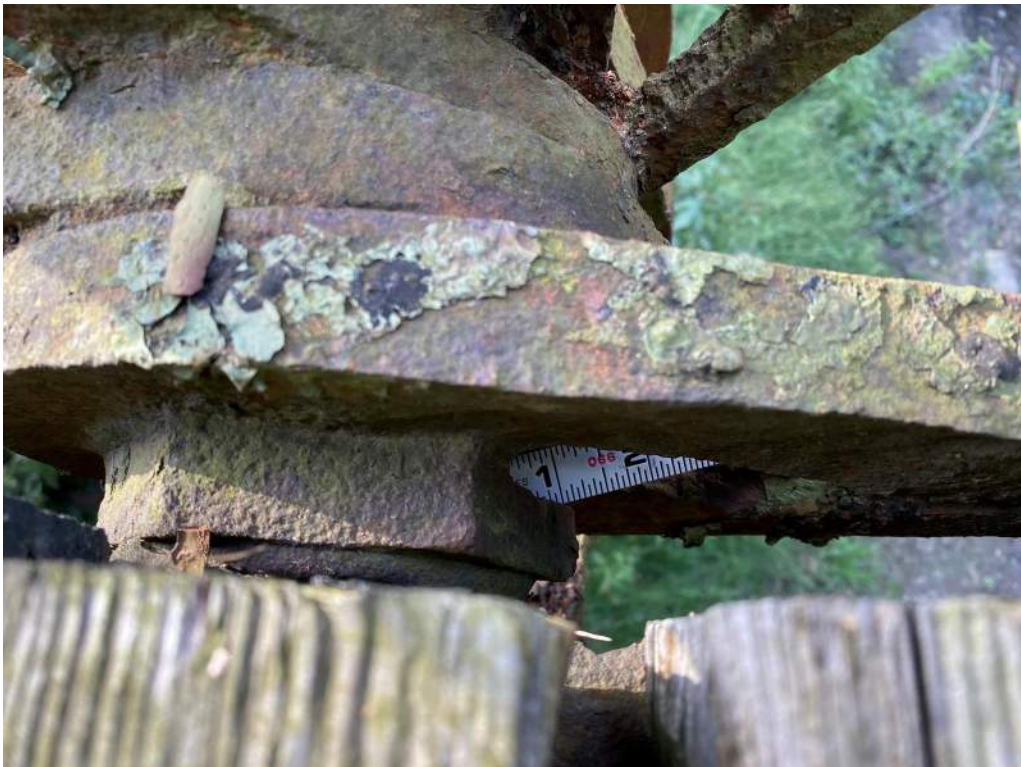
Photo 26: Section Loss on Pin and Interior nut of L3, North Truss
