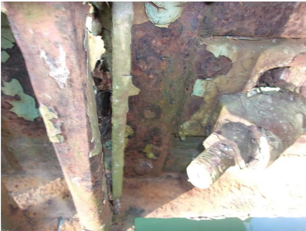
Photo 18: Missing Rivets on Floor Beam web at L9, South Truss
