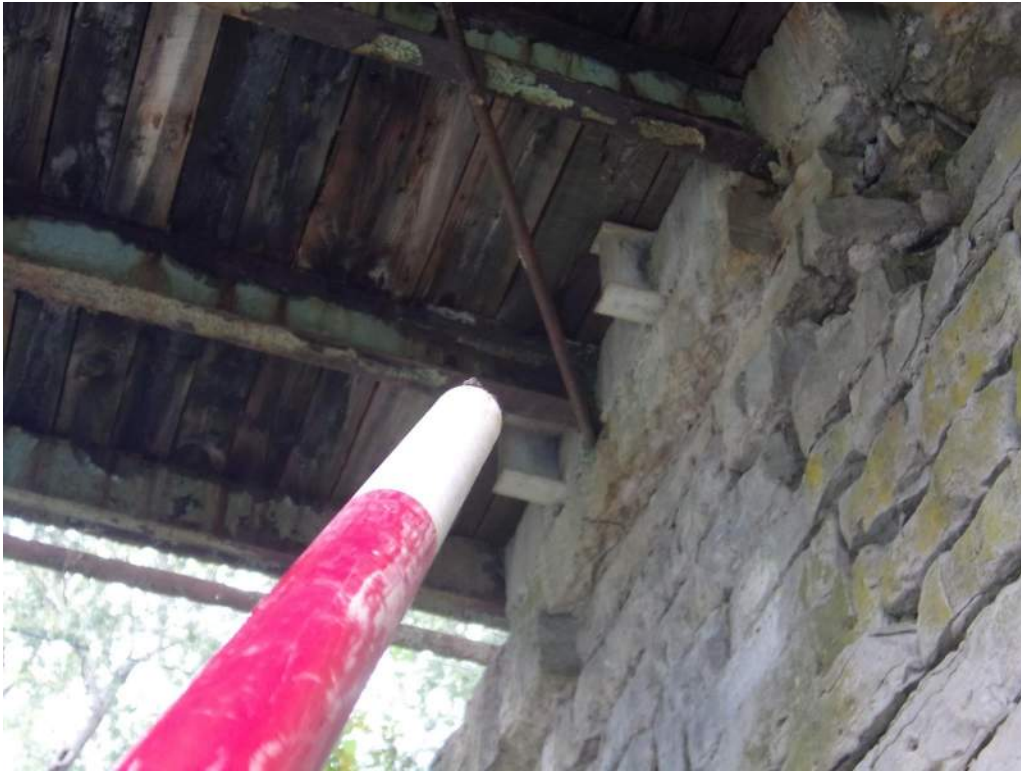
Photo 3: Hole in Stringer 6 Web, East Abutment
