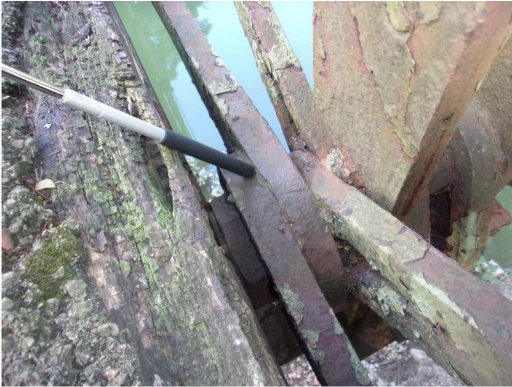
Photo 11: Typical Pack Rust and Rusting of Eyebars at Lower Connections, South Truss
