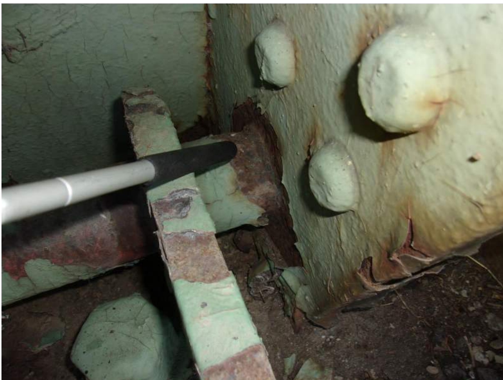
Photo 22: Section Loss on Pin at Interior Channel at L12, North Truss
