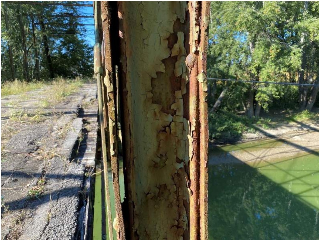
Photo 29: Out-of-Plane Distortion of Outer Plates between rivets with Broken Rivets at L9-U9, North Truss
