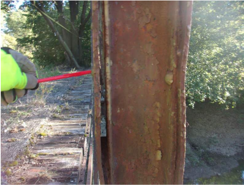
Photo 19: Out-of-Plane Distortion of Outer Plate and Broken Rivet at L9-U9, South Truss
