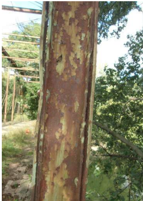
Photo 10: Broken rivets and Out-of-Plane Distortion of outer plate at L3-U3, South Truss
