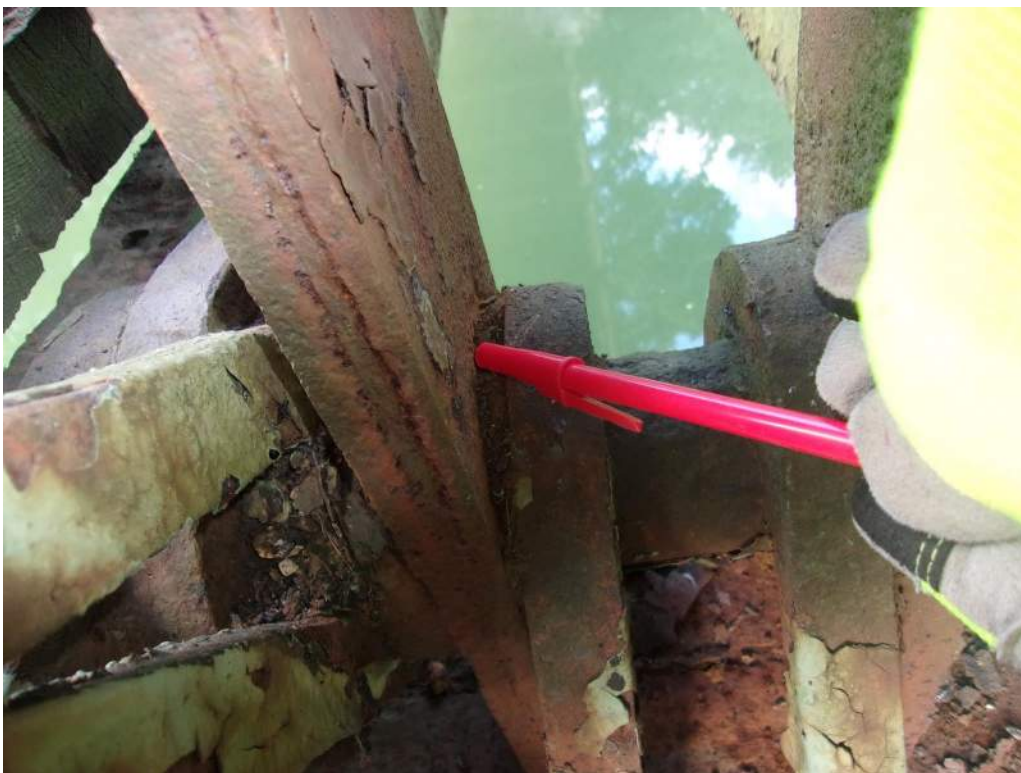
Photo 12: Pack Rust and Section Loss on Interior Plate of L4-U4, South Truss
