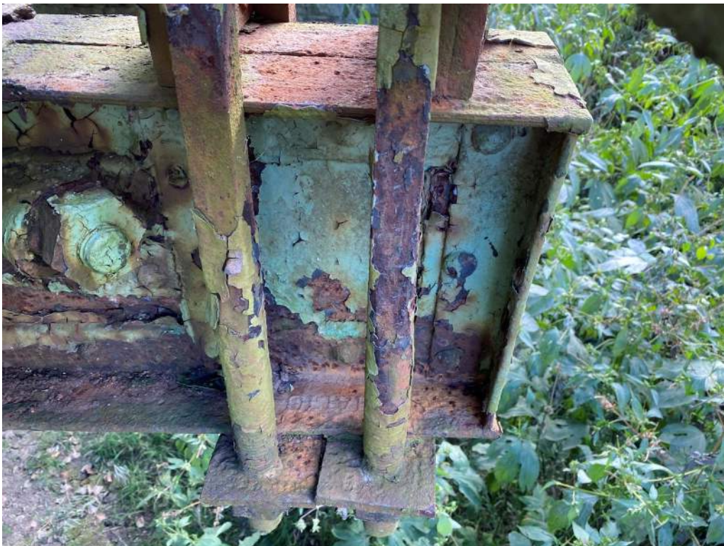
Photo 24: Heavy Pitting and Section Loss on Web and Bottom Flange on Floorbeam of L2, North Truss
