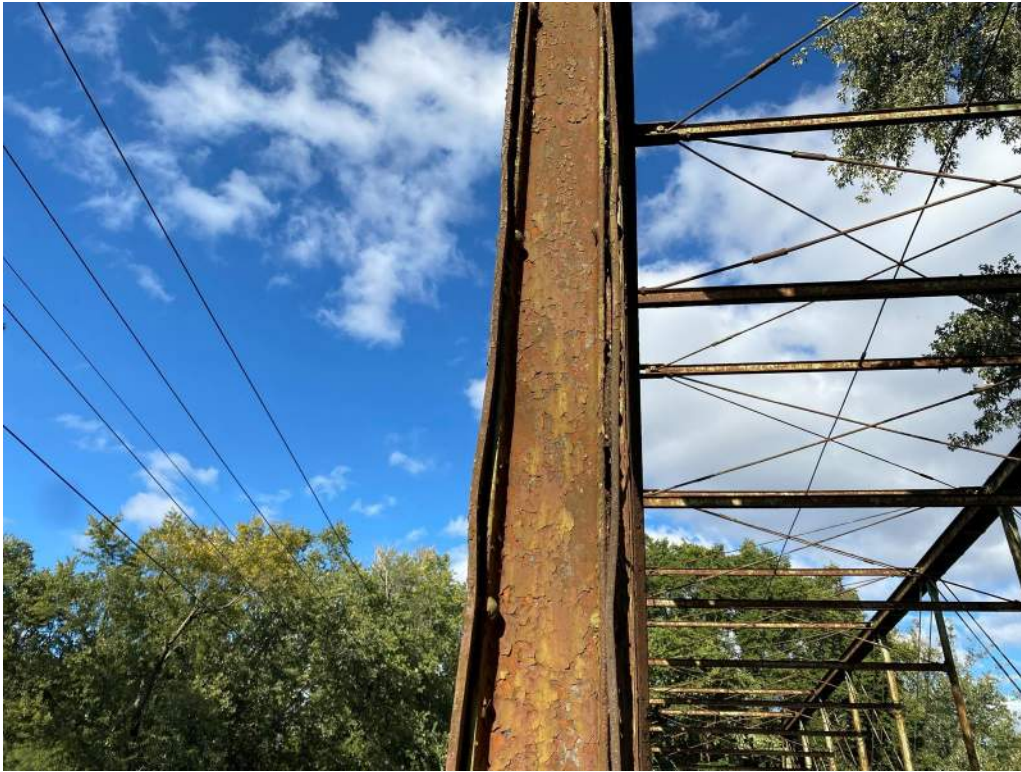
Photo 25: Out-of-Plane Distortion of Outer Plates due to Pack Rust at L2-U2, North Truss
