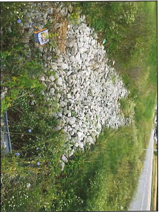
35. View of transition from vegetated swale to riprap in RSD 2 from culvert, approximately 24 inches in diameter, looking northwest.
