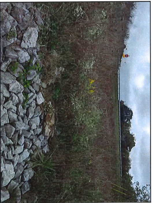
42. View of transition of riprap to vegetated swale in RSD 5, looking northeast.
