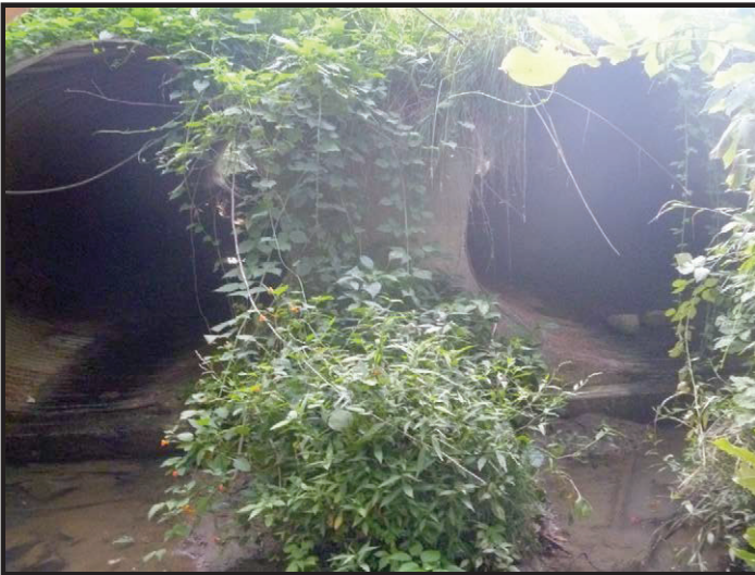
Photo 15 – SR 159 Culverts at UNT to Splunge Creek: Facing upstream to the west toward the outlet of Str. No. CV 159-084-23.30, from east of SR 159.
