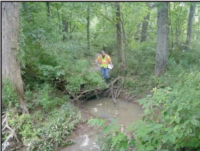
Photo 3 – UNT to Splunge Creek, Upstream from SR 159t: Facing upstream to the southwest along UNT to Splunge Creek toward the scour hole shown in Photo 2.
