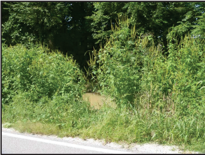
Photo 7 – SR 159 Crossing of UNT to Splunge Creek: Facing upstream to the southwest along UNT to Splunge Creek from the top of the SR 159 small structure.
