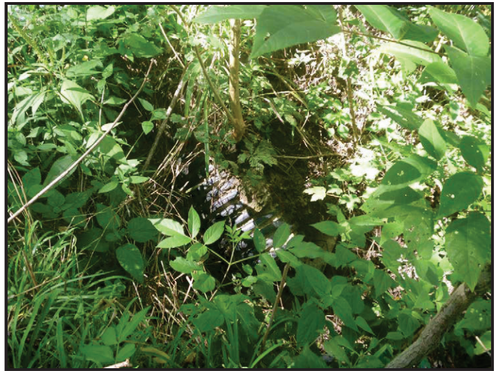
Photo 38 – Southeast Quadrant, RSD-1: Looking down at a plastic corrugated pipe, about six to eight inches in diameter within RSD-1.
