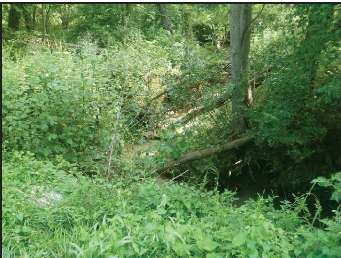
Photo 11 – SR 159 Crossing of UNT to Splunge Creek: Facing downstream to the east along UNT to Splunge Creek from the top of the SR 159 small structure. The left pipe flows freely, but the right pipe outfalls into a scour hole.
