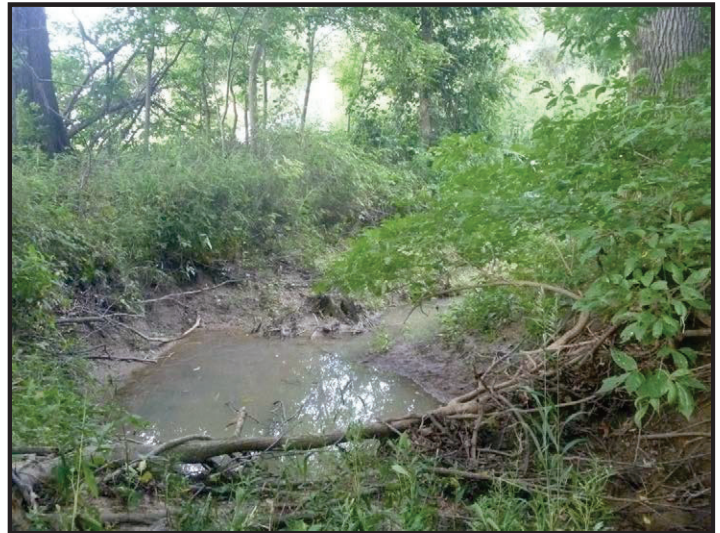
Photo 2 – UNT to Splunge Creek, Upstream from SR 159: Facing downstream to the northeast toward a scour hole at a small drop in the streambed.
