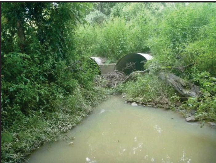
Photo 5 – SR 159 Culverts at UNT to Splunge Creek: Facing northeast toward inlet of SR 159 small structure, Str. No. CV 159-084-23.30, a set of twin, elliptical 47-foot-long steel pipes, each 8.5 feet wide and 6 feet high. The structure is proposed for replacement.
