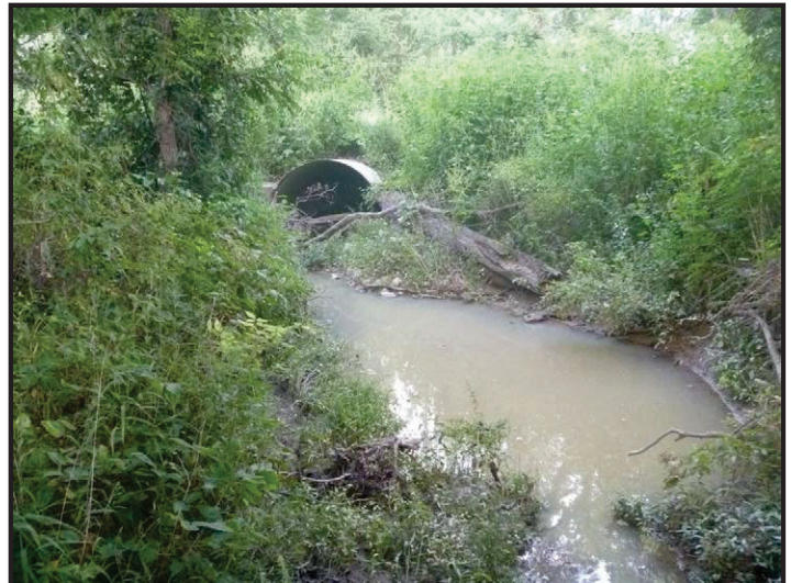
Photo 4 – UNT to Splunge Creek, Upstream from SR 159: Facing downstream to the northeast toward the scoured area at the inlet of the SR 159 small structure.
