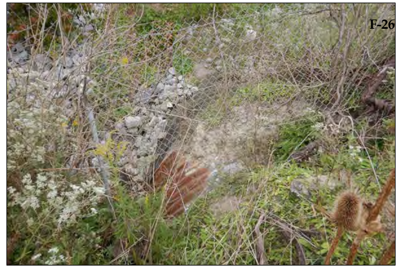
Photo 18: Flaugh Ditch culvert exposed within right-of-way south of Illinois Road, facing north.
