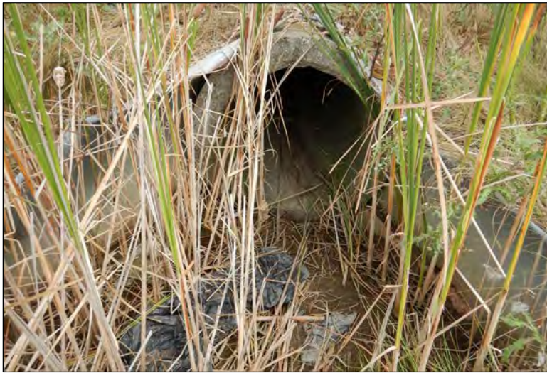
Photo 45: Culvert opening to Wetland 5 beneath I-69 North to SR 14 West exit ramp.
