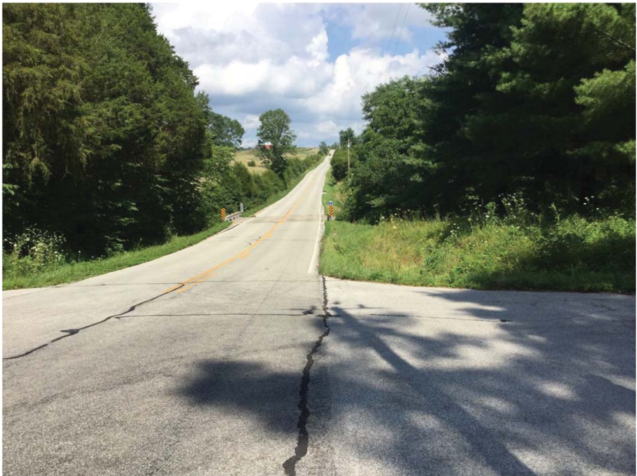
20. View of investigated area and the SR 250/South County Road 550 West intersection looking east
