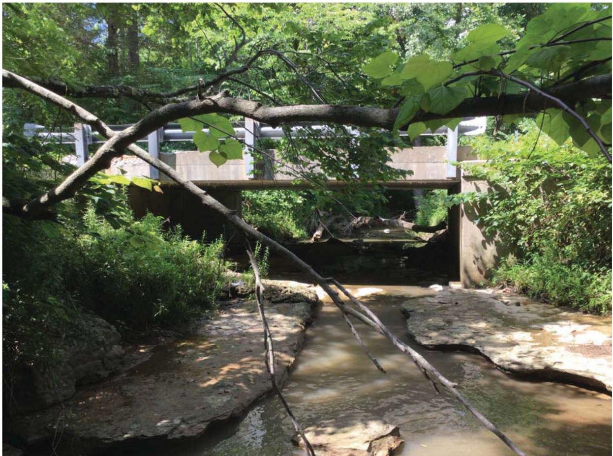
6. View of Slate Creek, the SR 250 structure and investigated area looking north
