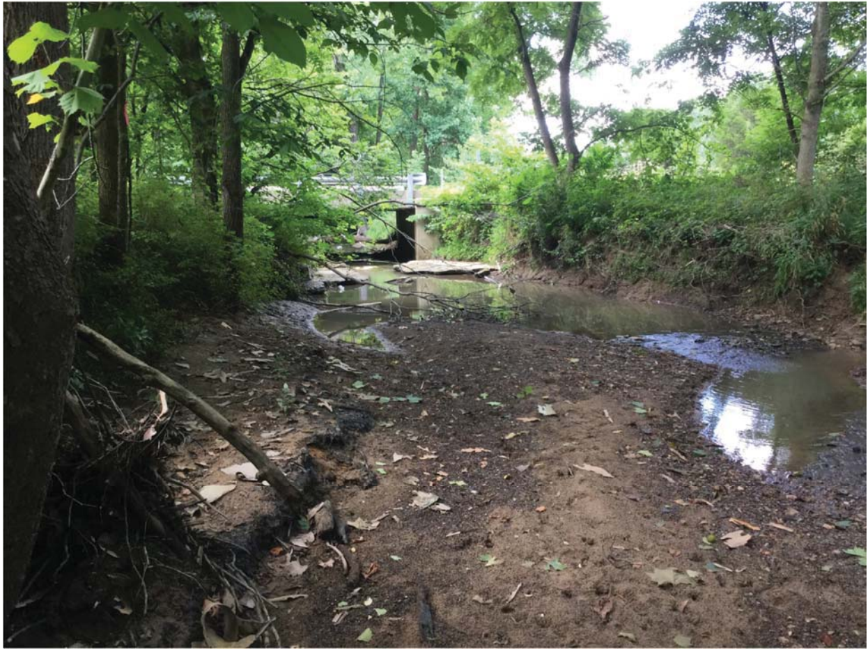
9. View of Slate Creek, the SR 250 structure and investigated area looking north
