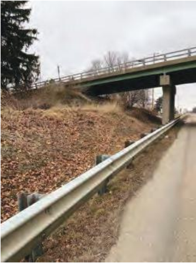
Photo 13. Facing north from west side of SR 9 to bridge proposed to be removed.
