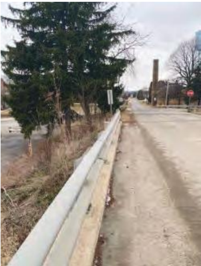
Photo 22. Facing west from western side of bridge to be removed; evergreen tree removal likely.
