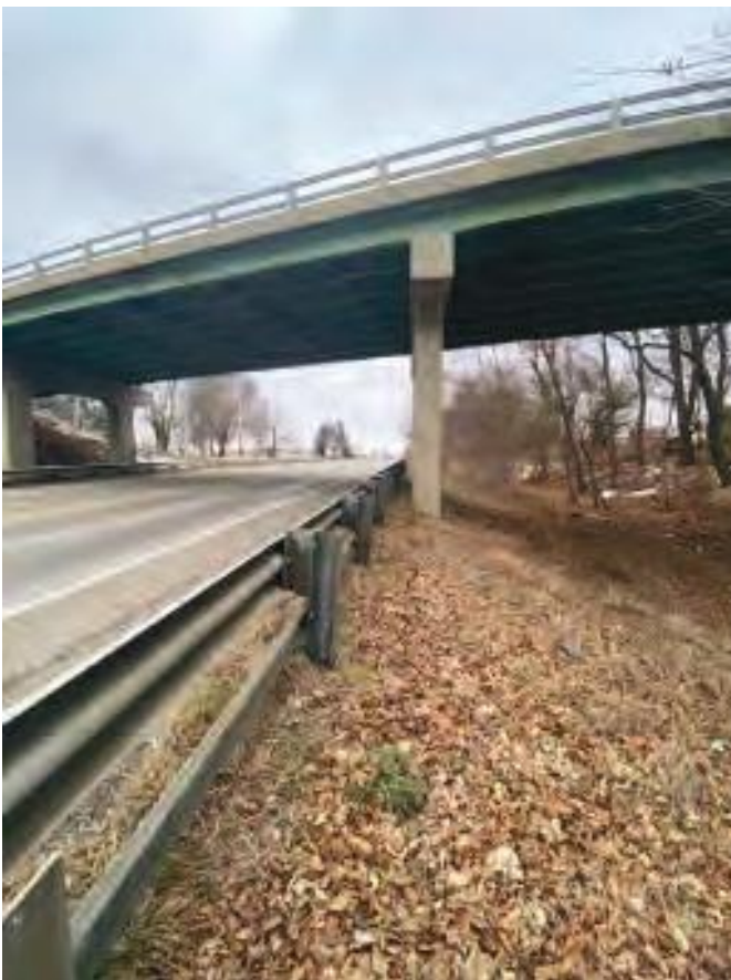
Photo 6. Facing north from the east side of SR 9 to bridge proposed for removal.
