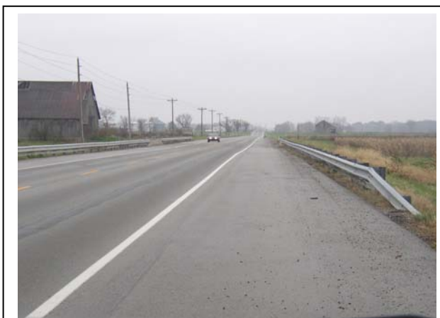
SR 9 is a relatively good two-lane highway through most of Shelby County, with ample shoulder width.
