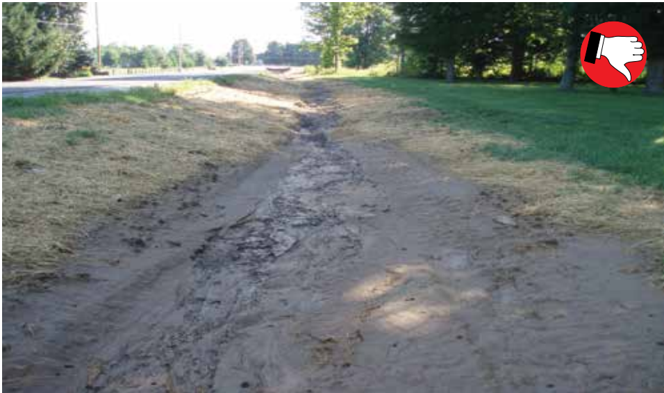
Ditches without blankets will wash the mulch away, disabling grass from growing and leading to erosion.
