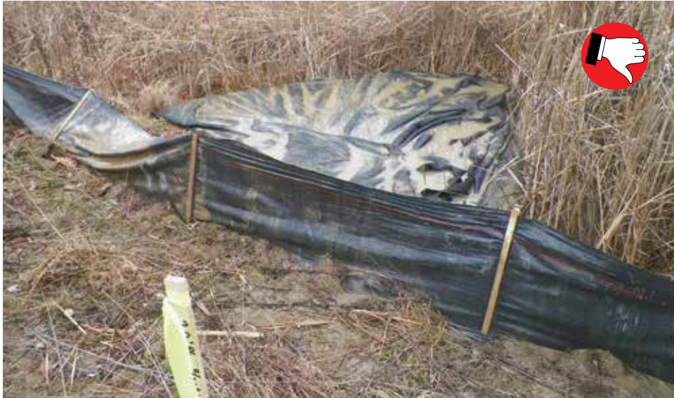
Filter bag has been placed outside construction limits and in a jurisdictional wetland. This would be considered a permit violation and cause for work stoppage and possible fines.
