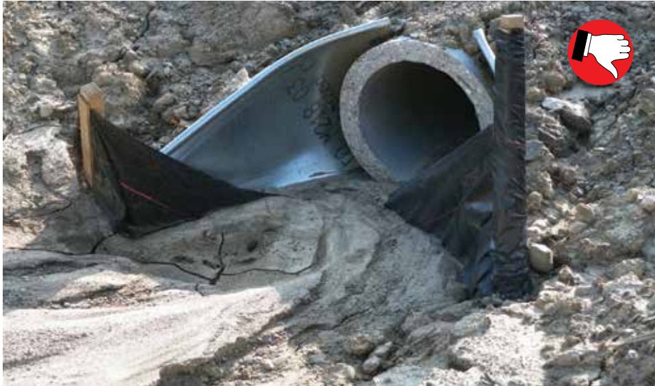
Silt fence should not be located in concentrated flow areas and is not appropriate as culvert inlet protection.
