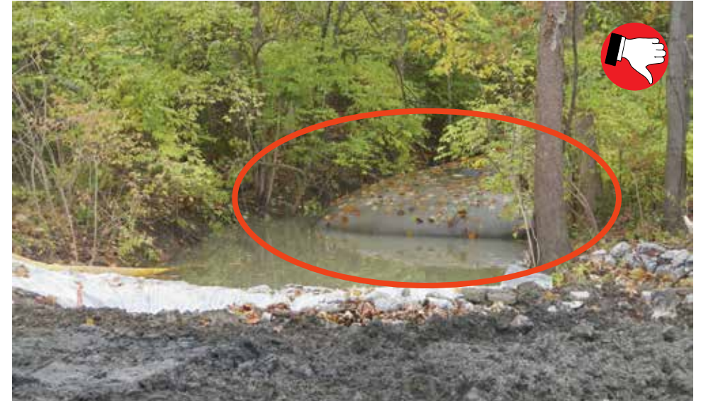
Filter bags should not be placed in waterways. Bags often break or become dislodged sending sediment downstream.
