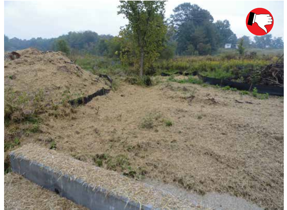
Blown mulch covering and clogging a jurisdictional waterway.
