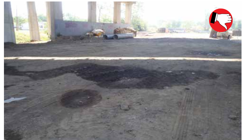
Prevent fuel or other toxic spills. Locate spill cleanup kits in accessible areas and clean up immediately.
