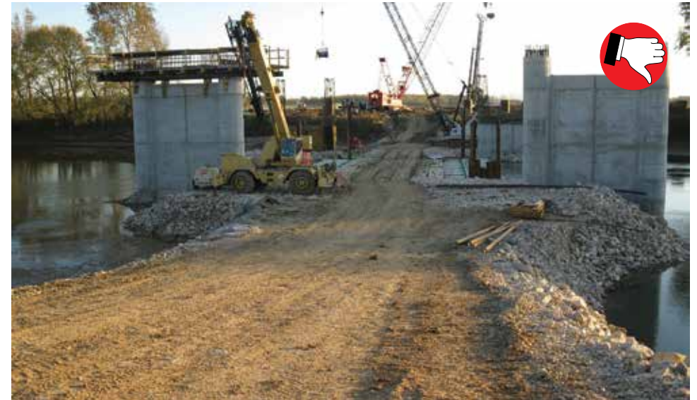
#2 stone on temporary crossing needs to be redressed to reduce sediment entering creek during rain events.
