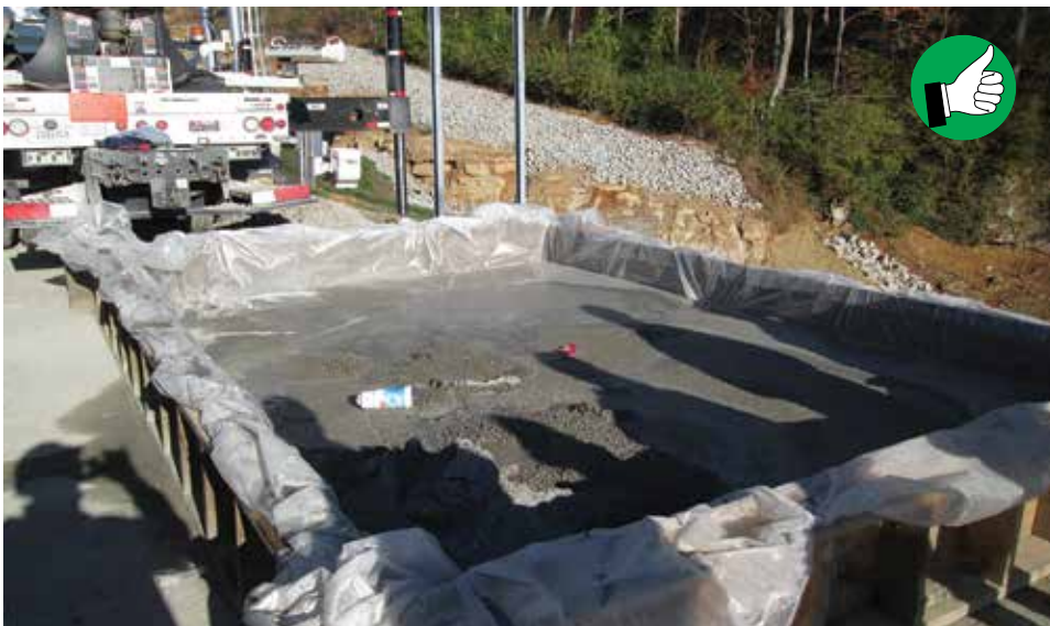
Good Example of an effective plastic lined dumpster washout. However, this washout has reached its capacity.
