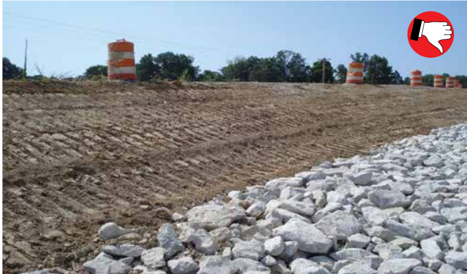
Vertical track marks will contribute to rill erosion.
