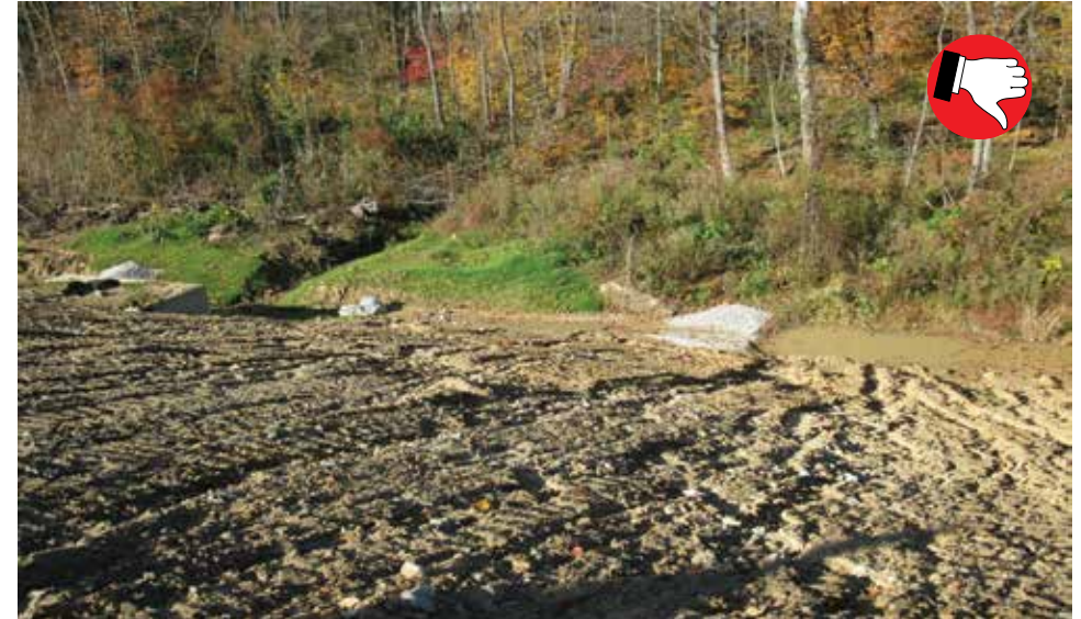
Trap placed too far away from waterway, should have a stable outlet to the creek and needs maintenance.
