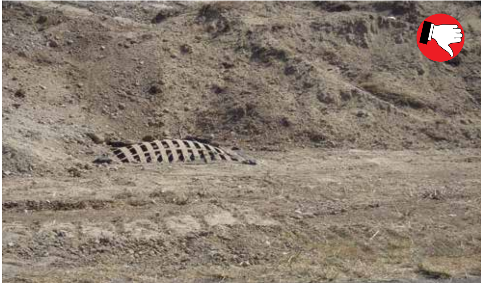
Geotextile placed under inlet is not an acceptable inlet protection measure. Geotextile will clog causing standing water, making measure impossible to maintain without getting muddy water into storm system. Ponding water could cause traffic hazards or muddy construction conditions.
