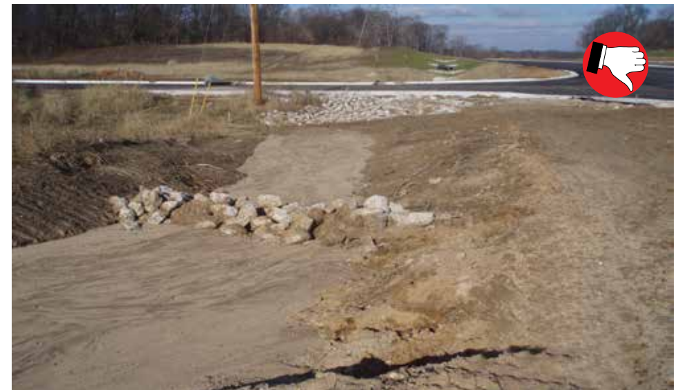
Rock check dam not built to specification. Not shaped correctly, no filter stone, no geotextile. The check dam should be rebuilt.
