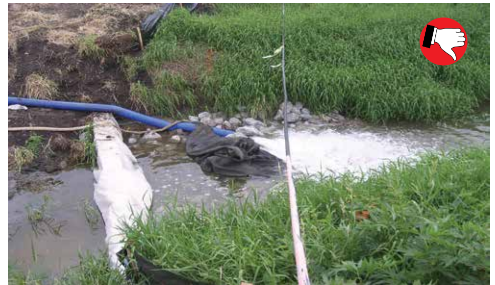
This pump around set up is wrong. Clean water discharging directly into a stream without an energy dissipater is causing erosion.
