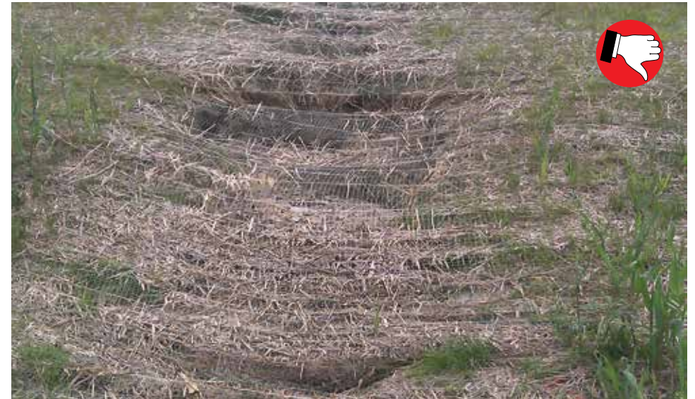
Erosion control blankets will not work if proper soil grading is not completed first. Blankets not installed parallel to direction of water flow.
