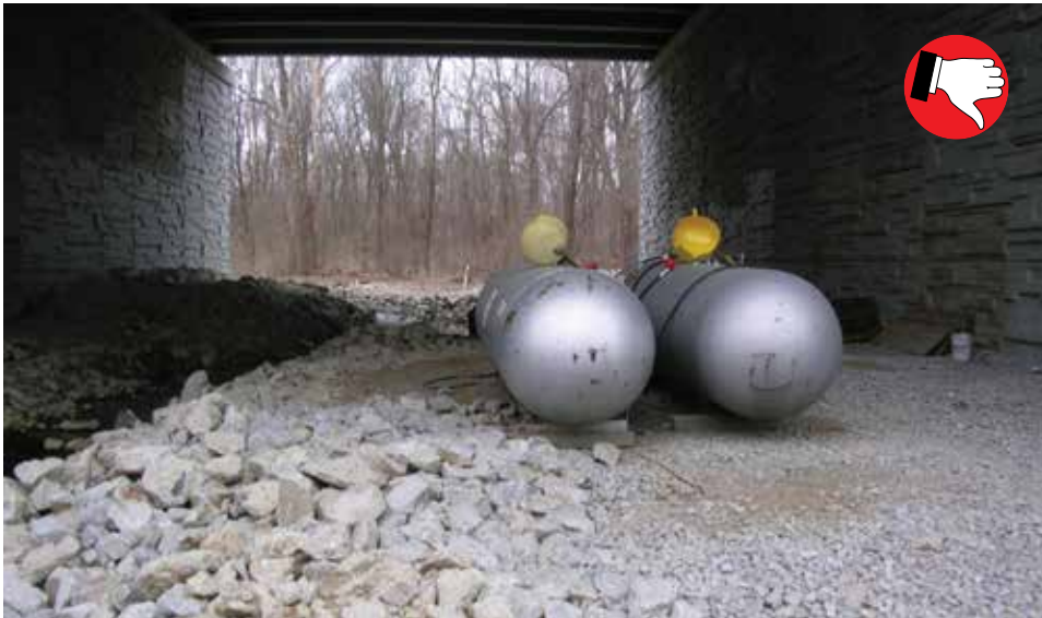
Locate fueling operations, temporary toilets and staging away from waterways and other hot spots.
