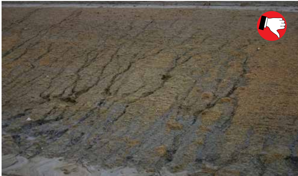
Temporary mulch applied too thin. Slope lacks erosion protection. Mulch and seed application rate should be per Specification.
