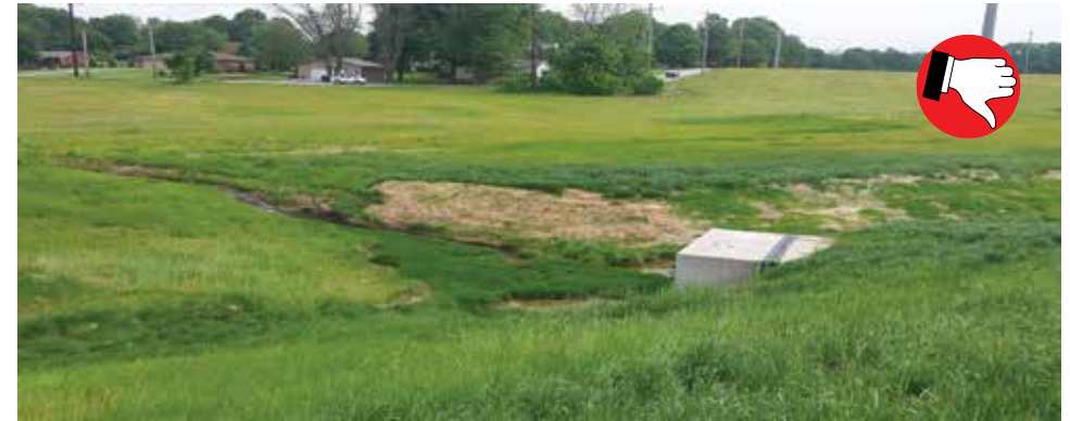
Sod failed because it was installed on a thick bed of straw mulch. An adequate growing surface is needed for the sod to take root.
