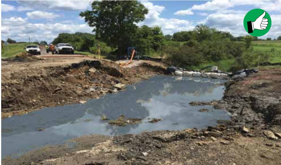
One Ton sand bags and plastic sheeting together makes an effective cofferdam to isolate the waterway during the bridge replacement.
