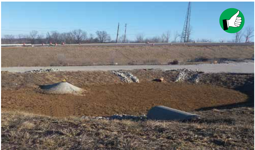
Sediment basin with stable slopes, stable outlets, filter stone and stand pipe.
