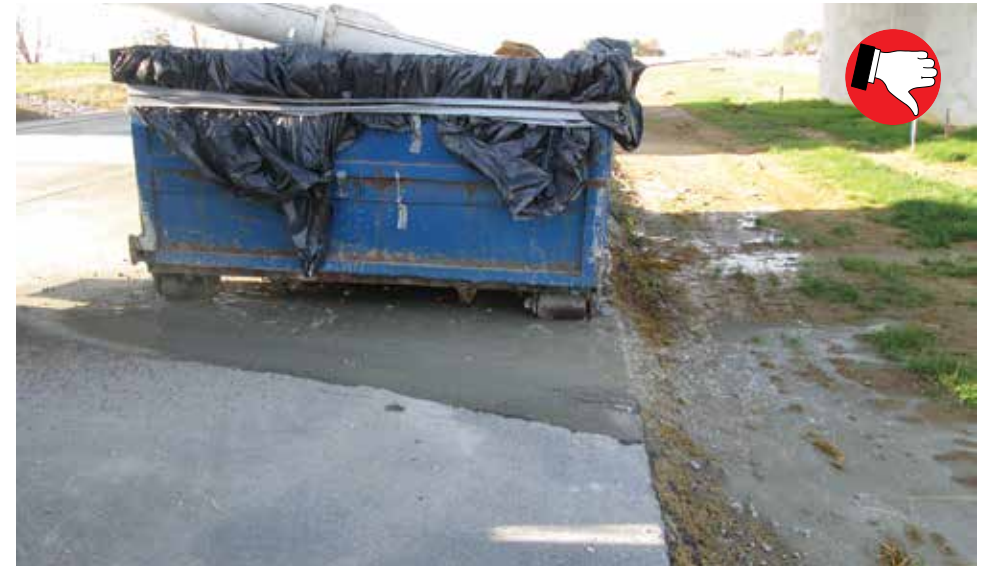
Plastic liner is too thin. Dumpster leaking while driver was washing out. Soil around dumpster contaminated, must be excavated and disposed of as per Standard Specifications 203.
