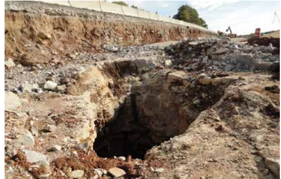
Previously unknown sink hole discovered during construction.
