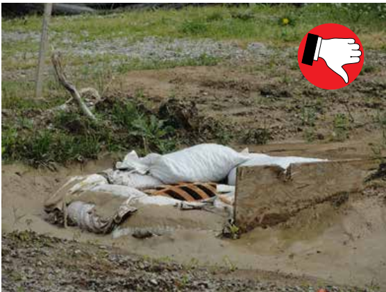
Inappropriate and ineffective inlet protection.
