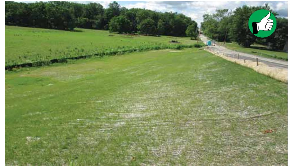
Erosion control blanket and filter sock together are assisting with the permanent seed establishment on this slope.
