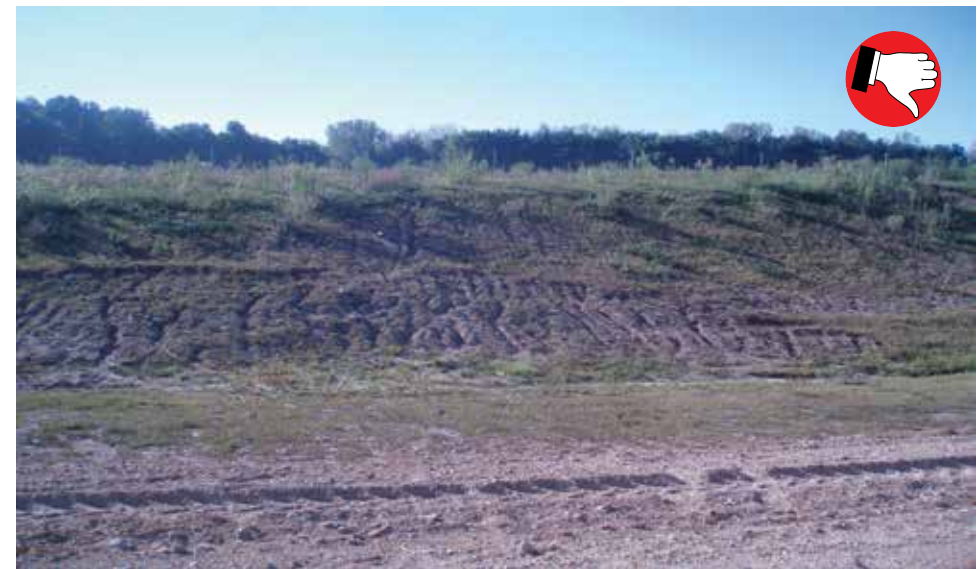
Vertical track marks make erosion worse and creates a series of rills to quickly move water and sediment to the ditch bottom.
