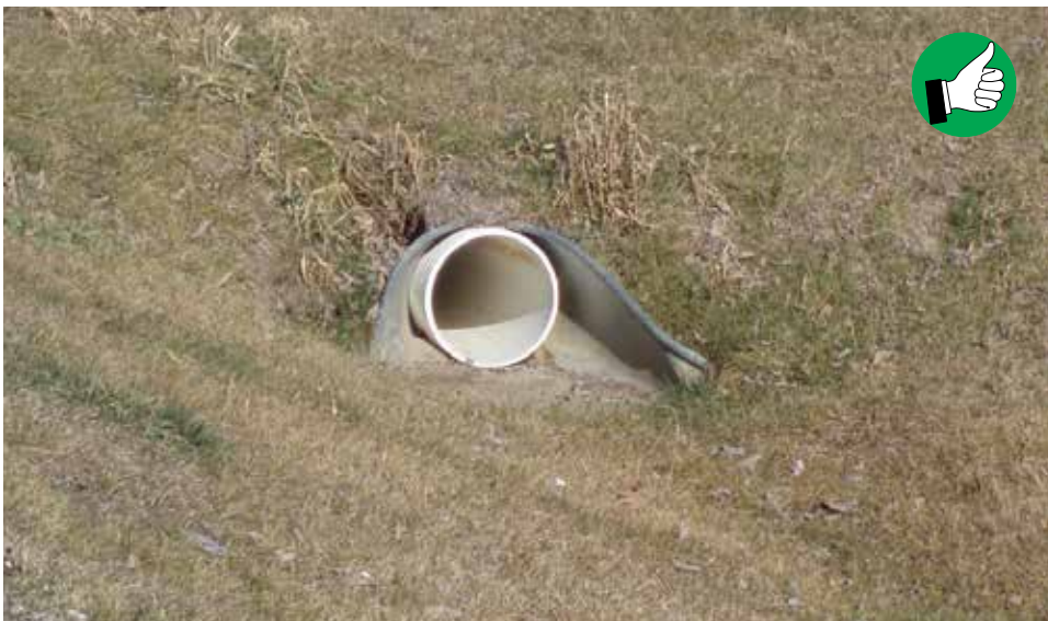
Pipe does not need riprap for permanent inlet protection because permanent vegetation was established for stabilization and velocity is low.
