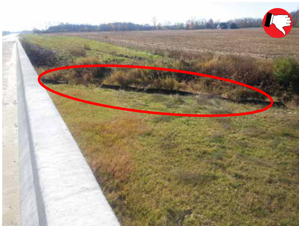
All temporary erosion and sediment control measures must be removed prior to issuing the NOT. Although the site is stable and more than 70 percent uniform density of vegetation, silt fence was left along the creek.
