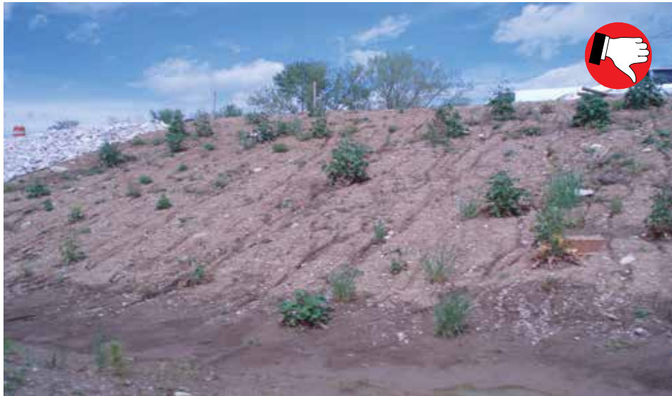
Weeds indicate slope has been unprotected for an extended amount of time. Temporary seed and mulch should have been applied within seven days of inactivity.
