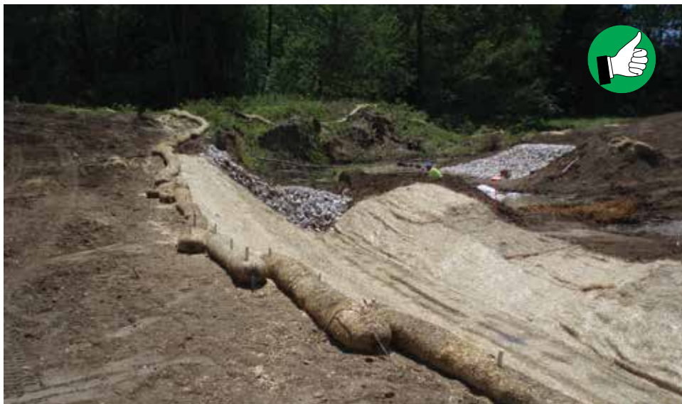
Stable diversion interceptor around a box culver installation. Diverted stream water should flow freely. Riprap should not be placed in channel.
