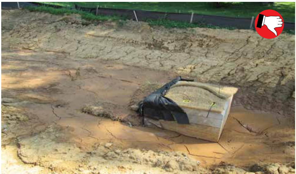
Sediment basins must have stable banks and a stable outlet, this live outfall structure is buried in sediment along with the straw bales being used to protect the structure.
