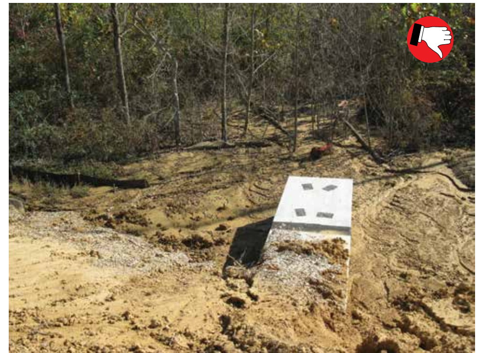
Sediment from construction site filling in a stream. This is a violation of many environmental permits.
