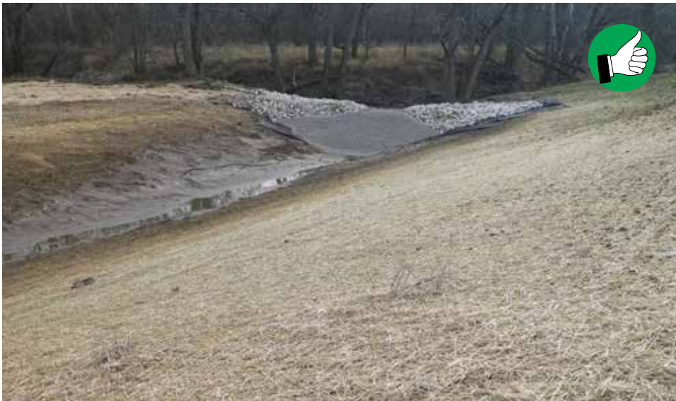
Sediment trap placed at the end of the ditch right before a waterway.
