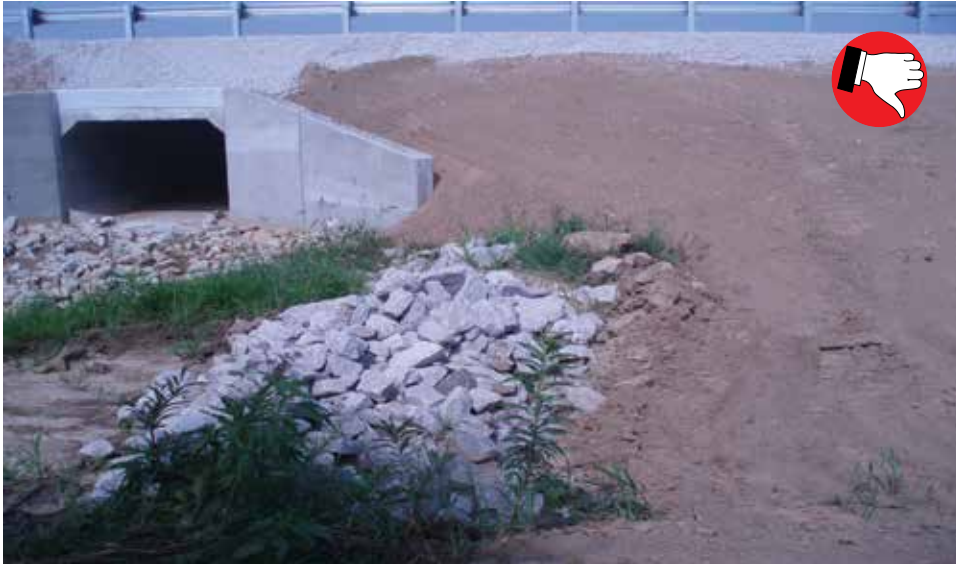
Sediment trap without filter stone allows sediment to travel through riprap and into waterway.
