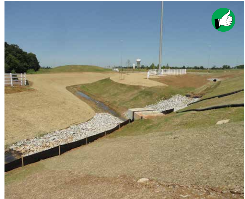
Multiple Storm Water BMPs working together to protect slopes and waterway.
