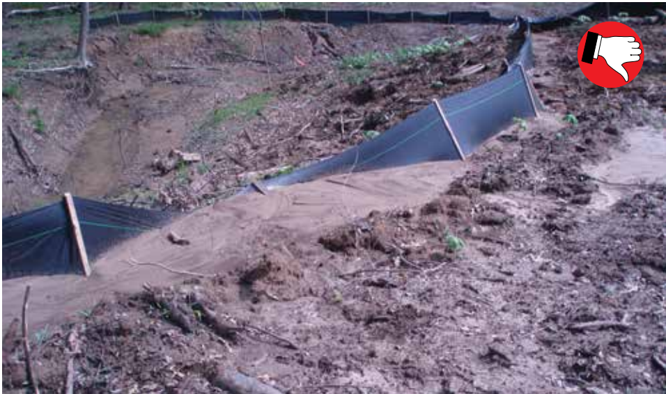
Silt fence is overwhelmed with sediment and requires maintenance.
