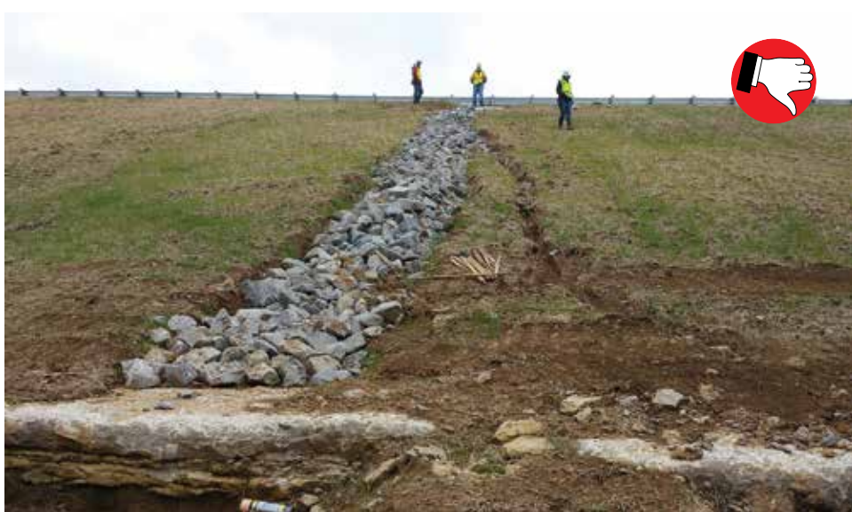
Water is bypassing rock chute.
