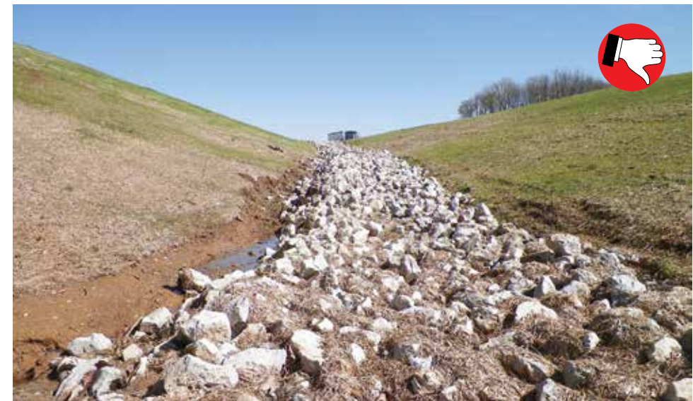
Riprap is not extended far enough up the slope and not shaped correctly, causing scour.
