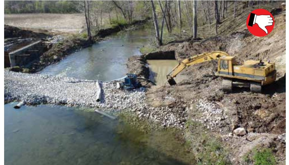
Bare earth is highly erodible and not a suitable barrier to be used for cofferdams. Water infiltration is evident.
