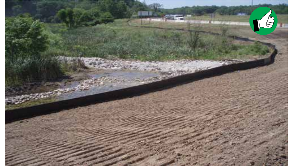
Horizontal track marks create small ridges and valleys to trap seed and mulch and help stabilize a slope.
