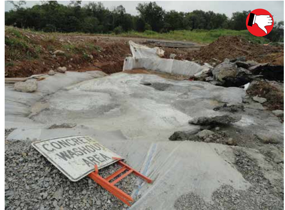
Concrete washout not properly maintained.
