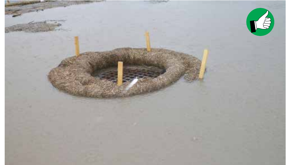
Filter sock inlet protection staked correctly.
