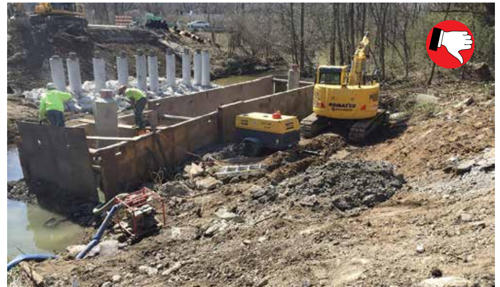
Ineffective sheet piling cofferdam. Sediment off-site in waterway.
