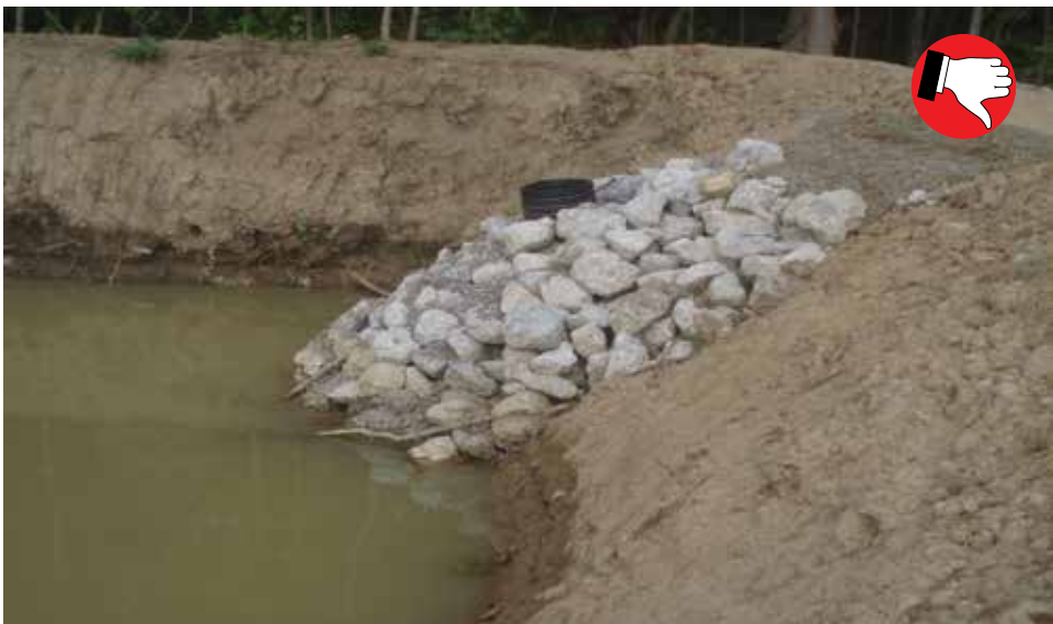
Sediment basin slopes are not stable and no filter stone is used on perforated stand pipe.
