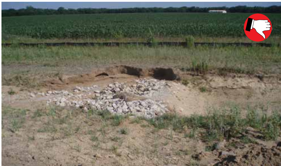
Check dam not shaped correctly causing water to bypass dam and erode slopes.
