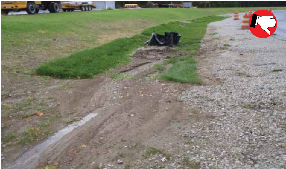
Area upstream of sodded ditch is not stable and causing sedimentation on permanent sod.
