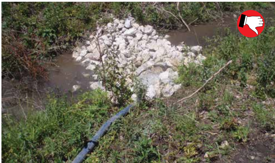
Stable outlet shall not be placed in the stream channel. This is unpermitted fill and a violation of 401/404 permits.
