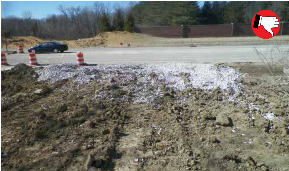
Construction entrance not the minimum 50' long. Tracking onto the roadway will become a safety hazard.
