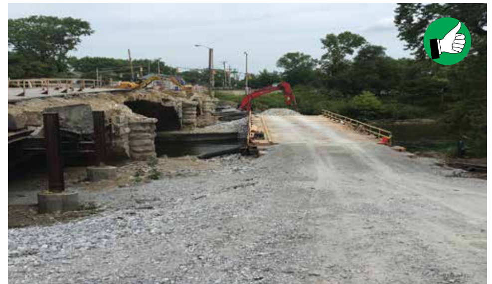
The use of this temporary bridge along with rock and geotextile fabric helps protect this stream from repeated equipment crossing.
