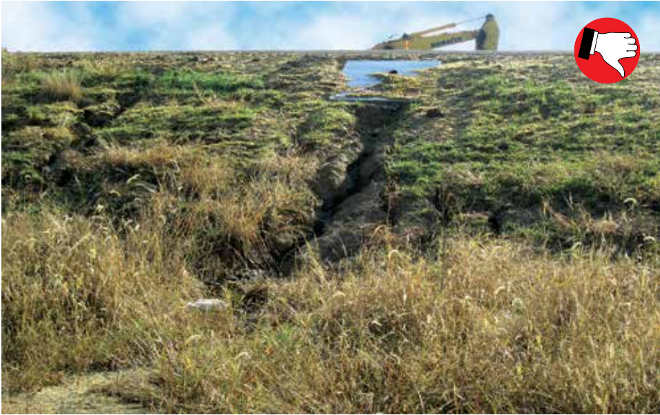
A slope drain would have prevented erosion from the underdrain.
