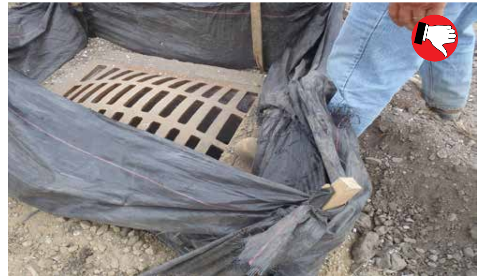
No cross bracing used on inlet protection. Silt fence not trenched properly.
