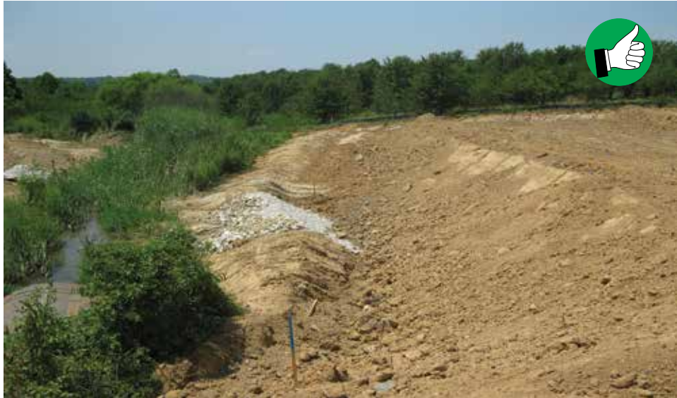
Diversion interceptor directing water to a filter berm.
