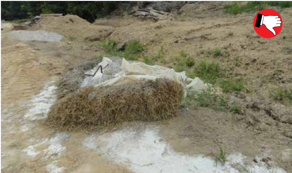
Straw bale containment not allowed on INDOT contracts.
