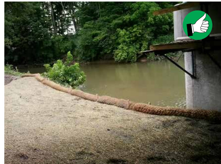
Filter sock and erosion control blanket together providing adequate protection for this stream bank.
