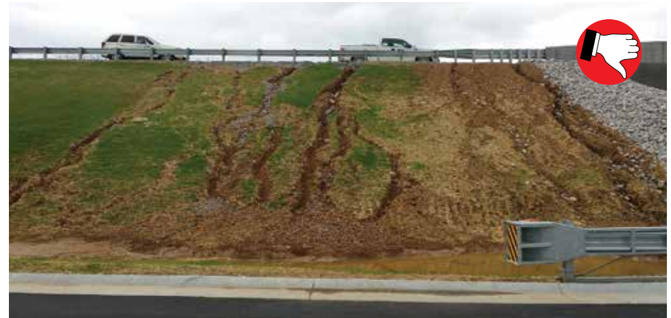
A slope drain would have prevented this erosion caused by water running off bridge super elevation.
