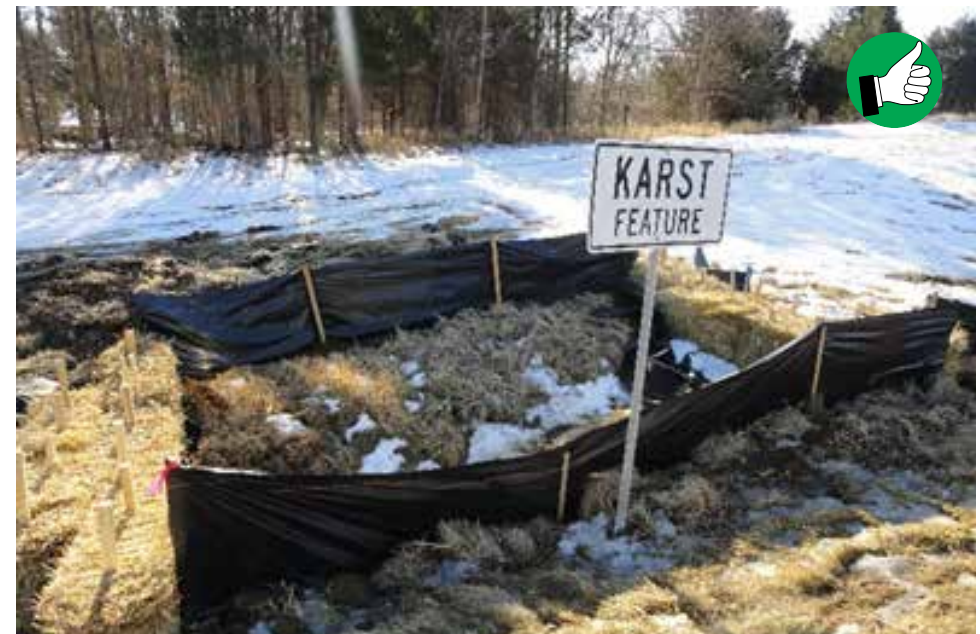
A sink hole being protected during active construction.
