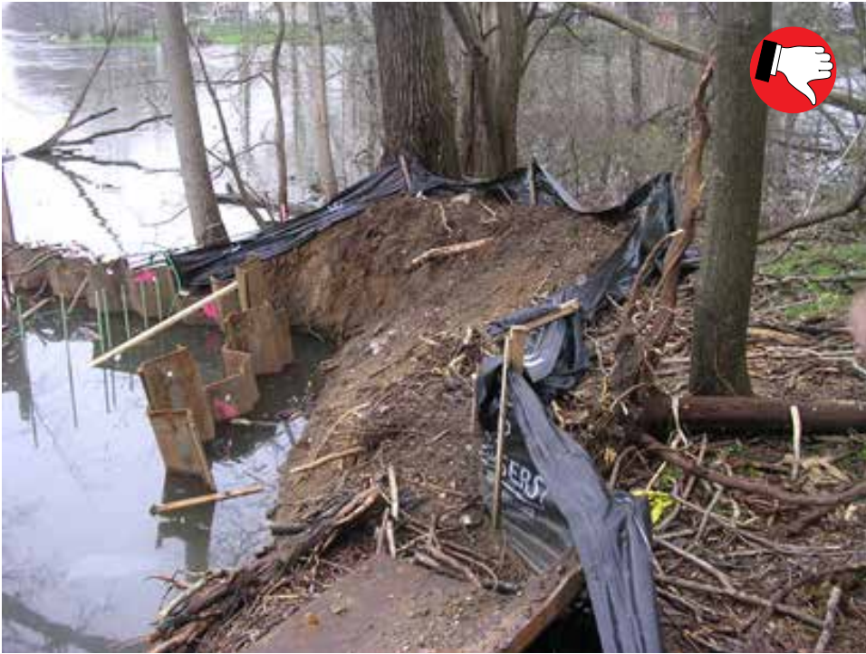
Silt fence does not hold its integrity in areas prone to flooding. INDOT-ES strongly recommends not using silt fence near stream banks. A filter sock is a more appropriate BMP around stream banks.
