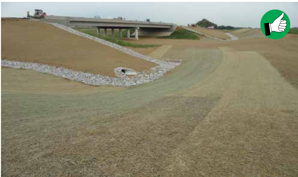
Erosion Control Blanket being used for permanent vegetation establishment and slope protection.
