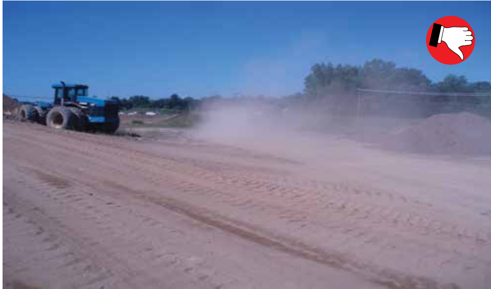
Dust contributes to air pollution, can interfere with drainage and can create traffic hazards.
