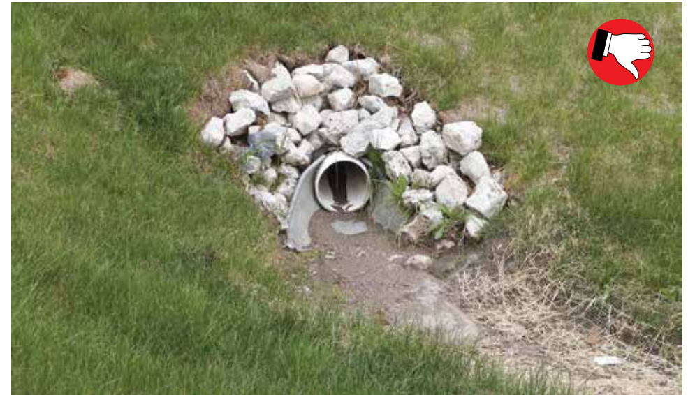
Permanent inlet protection without geotextile fabric and haphazard placement.
