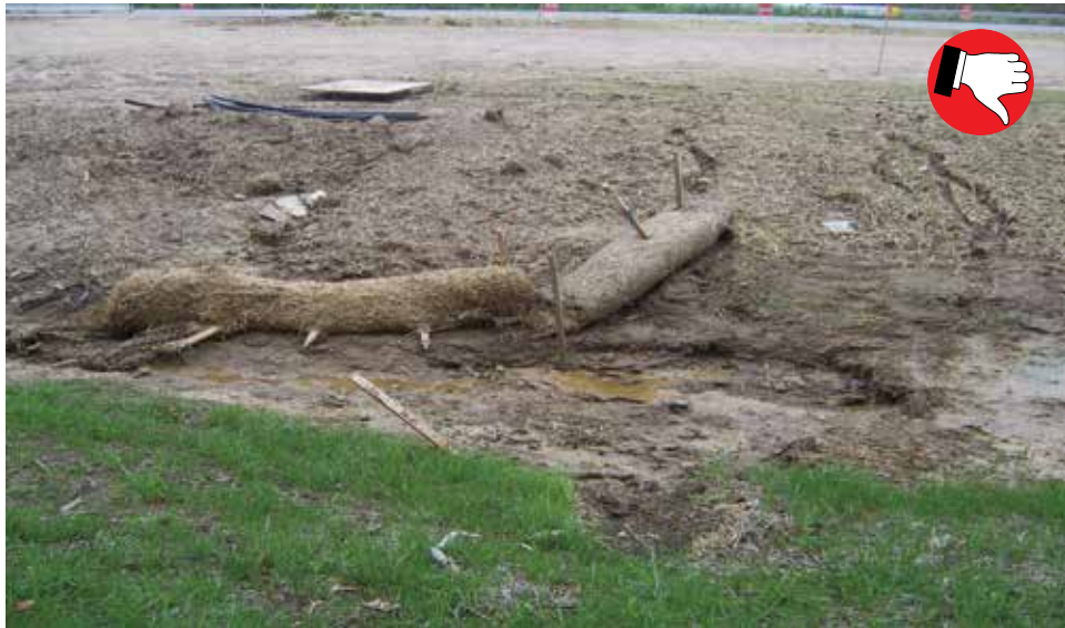
Filter sock used as traversable check dam in the clear zone (good) but installed where water velocity is very high (bad). No geotextile was used and only one filter sock was used (verses three in a pyramid).
