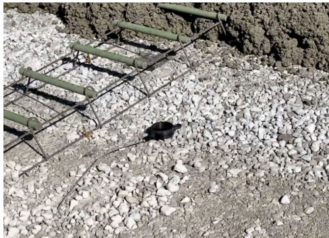
Figure 3 Example of typical Strength Meter installation (Courtesy Dr. Luna Lu, Purdue University)
