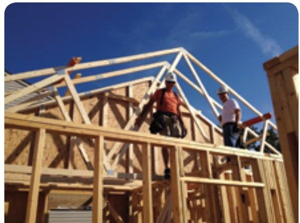
Construction of a home at 8803 Taggart Drive in Camby for the Casillas family
