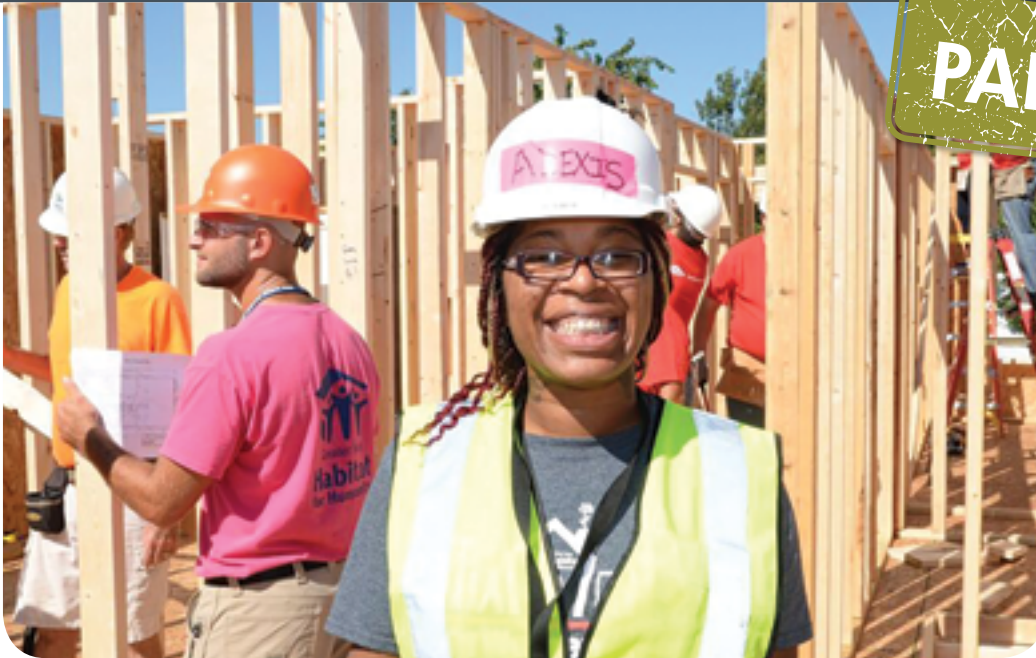
Alexis Hardin is pictured at the construction of her home on 3122 Broadway Street in Indianapolis
