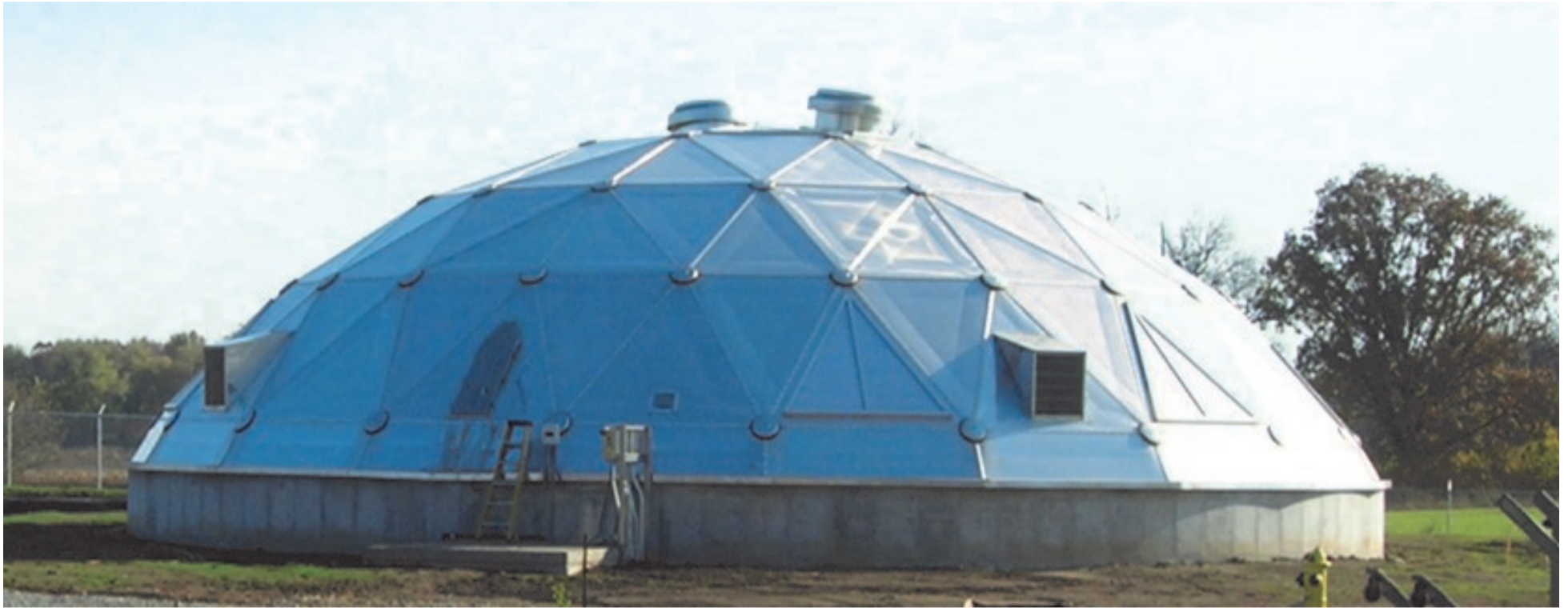
Bargersville's backwash recycle tank.
