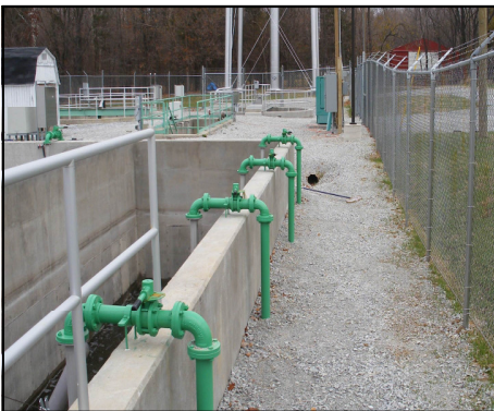
The new aeration tank at Hartsville's wastewater treatment plant
