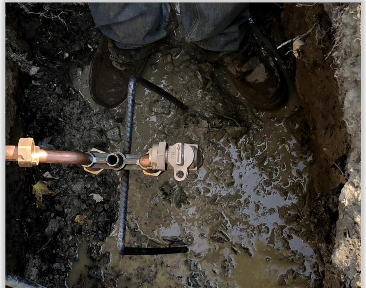
New Water Meter installed in Centerville, IN—part of the Town's Water Distribution Improvements Project
