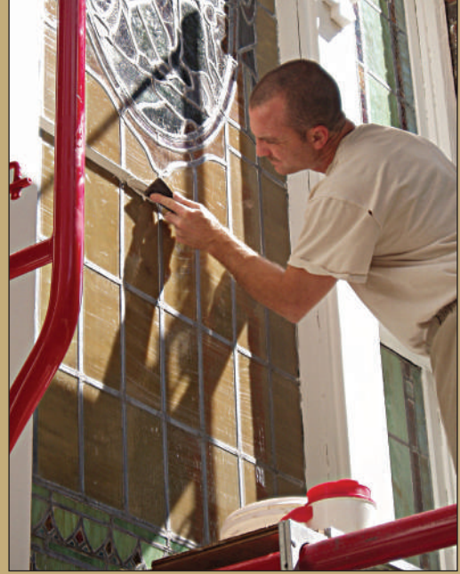
A resident works to restore a chapel window to its original beauty. Residents use the chapel for worship services, weddings, and theatrical performances. It's also used as a gathering place for facility-wide "town meetings," which include residents and staff. Plainfield Re-Entry Educational Facility
