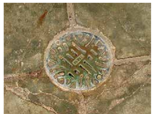
Filled in floor drain.
