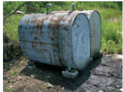
Release of fluids from above ground storage tanks in poor condition with no label.
