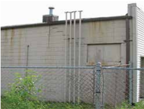
Vent lines for a UST.
