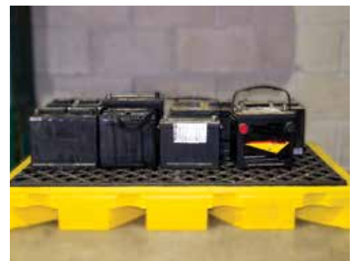
Batteries stored inside with secondary containment.
