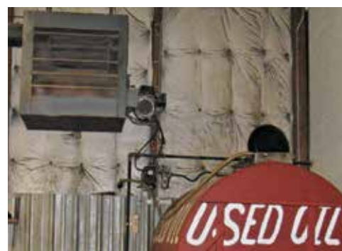
Space heater with labeled used oil storage tank.
