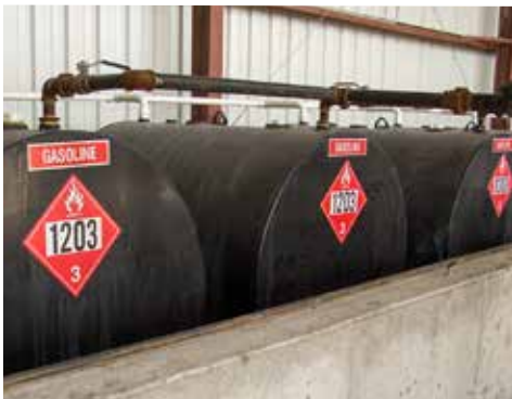
Properly labeled and stored fluids in stationary secondary containment.
