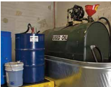
Properly labeled and stored fluids.
