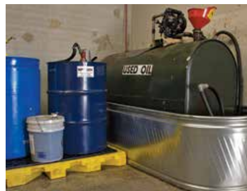
Used oil storage tank in secondary containment.
