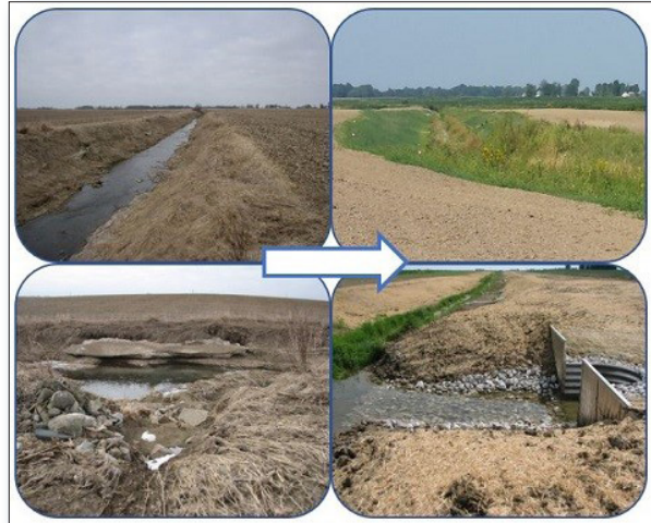
Figure 2. Before (left) and after (right) showing BMP implementation on Stump Ditch. The two-stage ditch increases bank stability while improving drainage and ecological functions.
