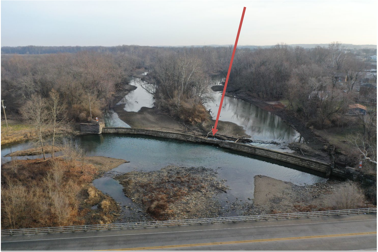
Figure 15. Thompson Mill Dam looking upstream. Note breach in the middle part of the dam.
