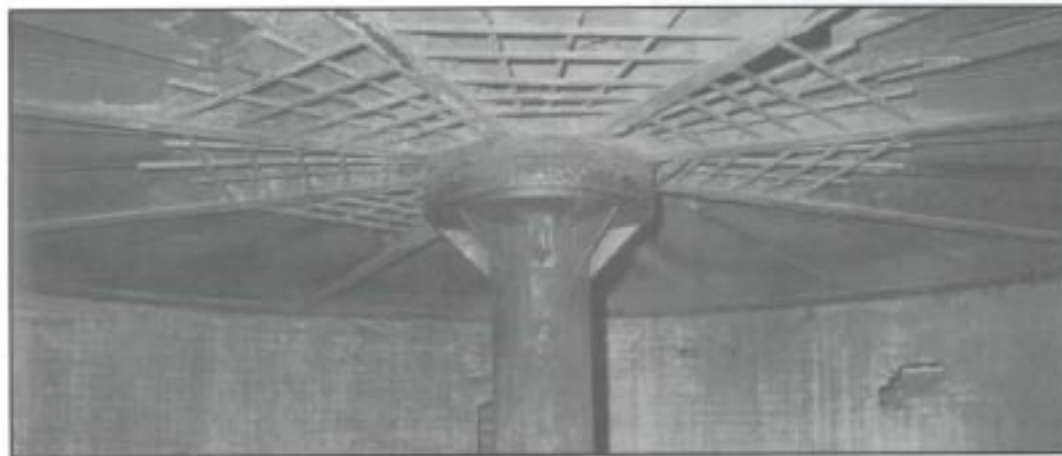
Central shaft with main bearing ring and supporting ribs in the basement, 1968. This jail was the only rotary jail built to rest on a central column; the others were suspended from the supports.
