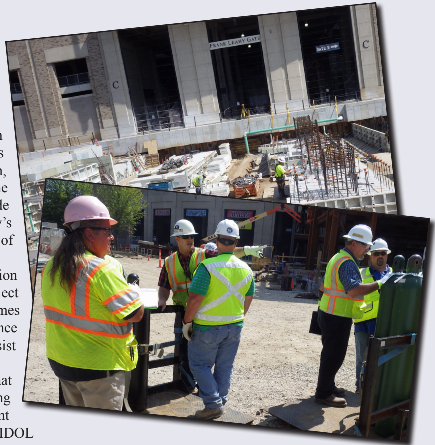
Top photo: Construction crews perform work onsite at the University of Notre Dame Campus Crossroads Project in South Bend. (Photo by John Grimes) Photo 2: IOSHA Construction Safety Division compliance safety and health officers Ellen Osborne and Dave Zeigenbein walk the jobsite. (Photo by John Grimes.)
