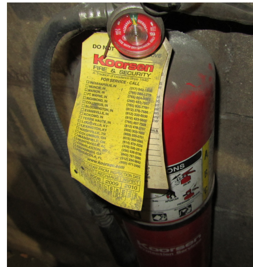
IOSHA Top Ten Most Violated Standards, number 9, Fire Protection: Fire extinguisher is nearly two years past the due date for the required annual service. (Photo taken by IOSHA Compliance Safety and Health Officer Jeanne Hedge)
