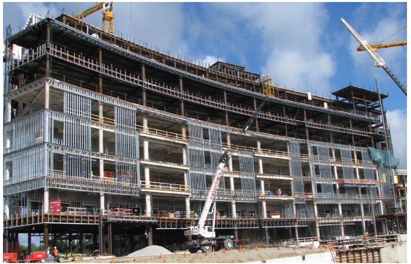
Parkview Regional Medical Center: This photo was taken to reference the progress of the construction underway at the Parkview Regional Medical Center, in Fort Wayne, Indiana. The Indiana Department of Labor is actively engaged in a strategic occupational safety and health partnership with Weigand/Pepper JV. (Photo taken and submitted by Sheryl Wiser, Safety Manager - Fox Contractors)
