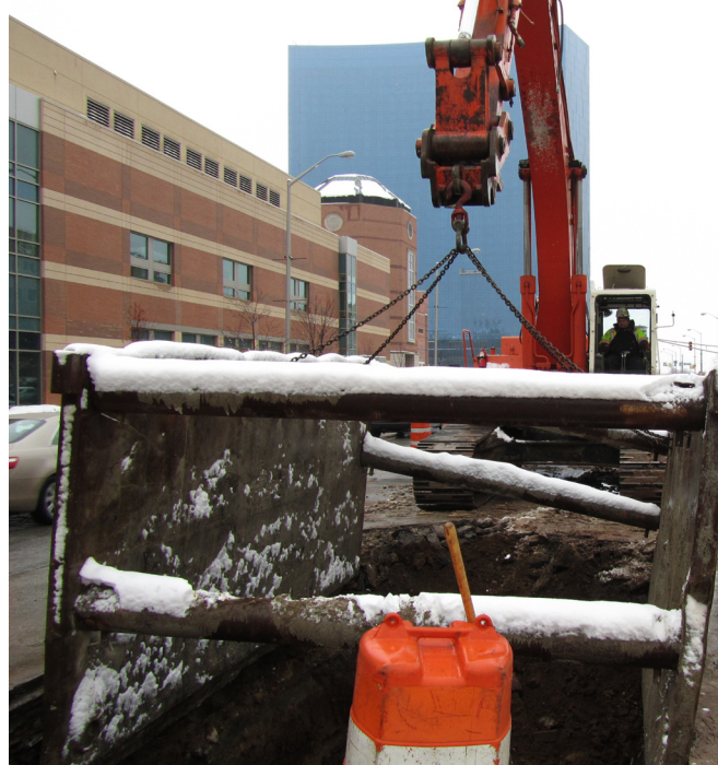
A trench box is placed in a trench during construction on Washington Street in Indianapolis, Indiana. (Photo taken and submitted by Deputy Commissioner Jeff Carter)
