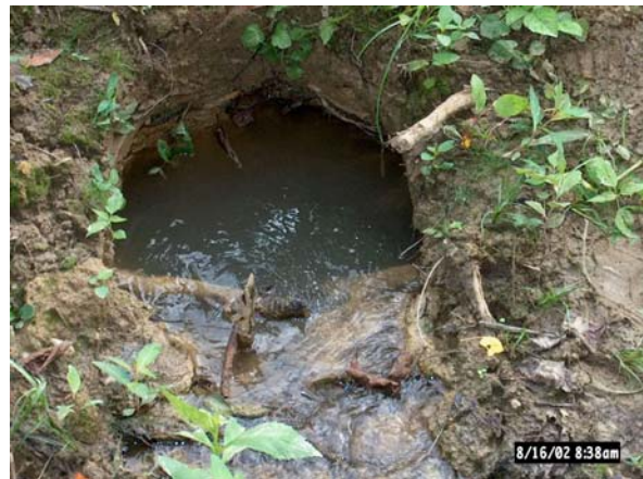
Figure 2 - Boil near toe of embankment (12-inches diameter)
