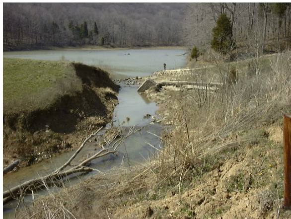
Figure 6 - Apparent seepage along this concrete spillway caused total erosion of the structure.
