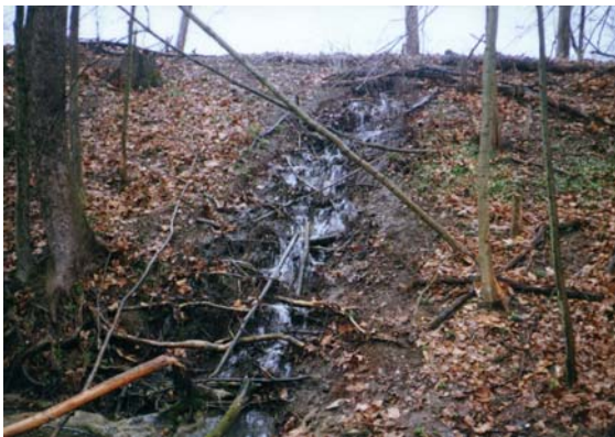
Figure 2 – Seepage through tree roots
