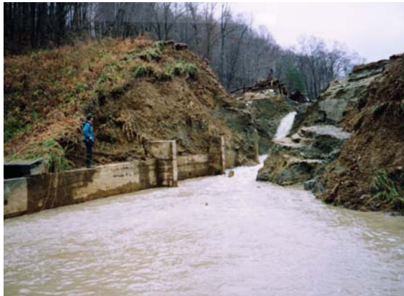
Figure 1 – Earth dam failure
