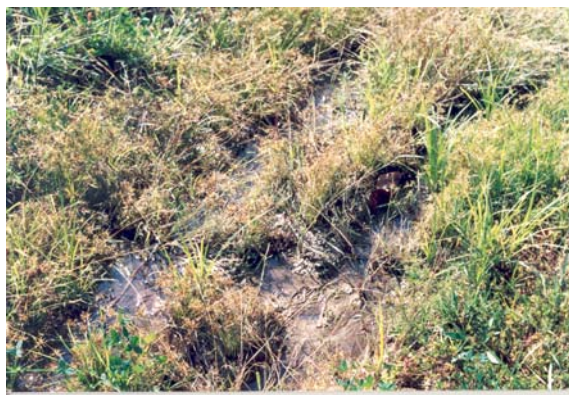
Figure 3 – Seepage flows on vegetated embankment
