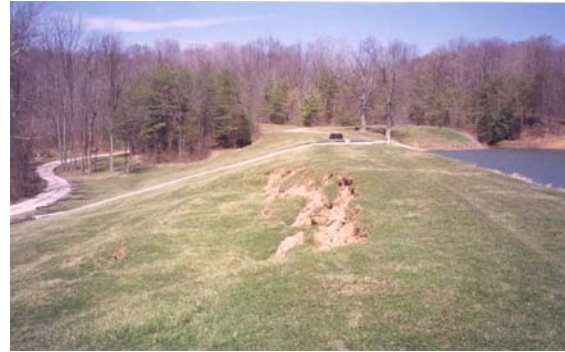
Figure 3 – Structural failure resulting in a slump condition
