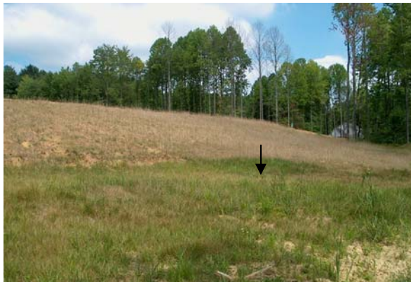
Figure 1 - Seepage at embankment toe caused sloughing
