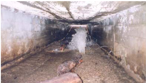
Figure 4 – Rupture of concrete spillway conduit
