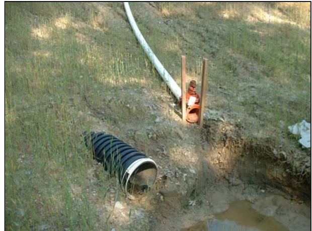
Figure 2 - Plastic pipe used as the principal spillway; the use of this type of plastic pipe is not recommended
