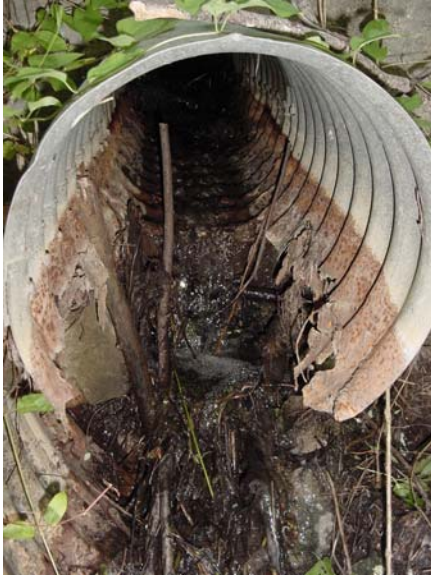
Figure 3 – Corrosion of corrugated metal pipe
