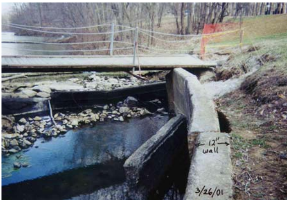
Figure 1 – Concrete Wall Displacement
