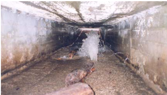
Figure 2 - Rupture of concrete spillway conduit
