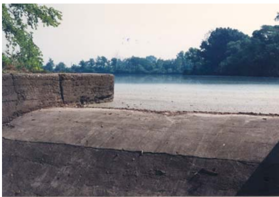
Figure 1 – Concrete spalling and cracking
