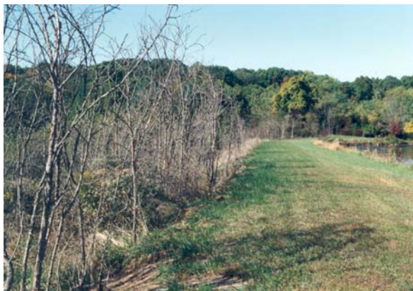
Figure 1 – Trees and brush on dam embankment
