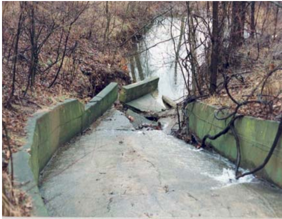
Figure 3 – Concrete spillway cracking and undermining
