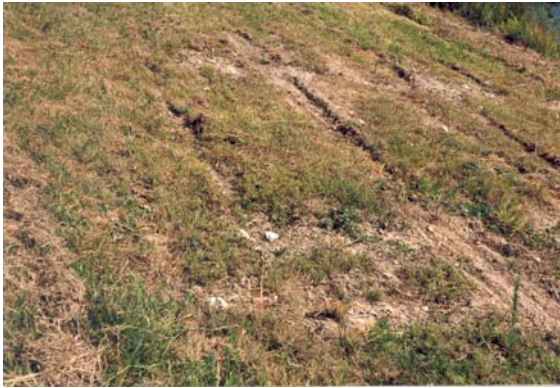
Figure 1 – Rill and gully erosion
