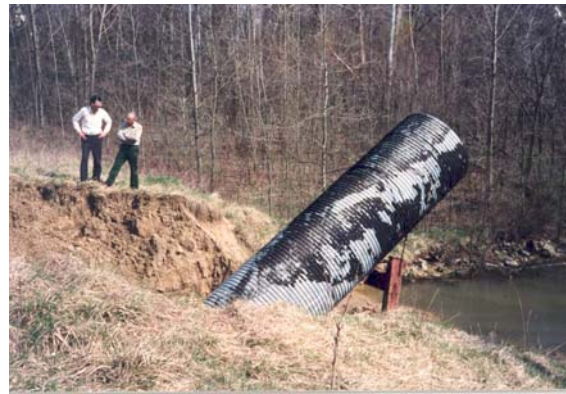
Figure 1 – Undermining of principal spillway conduit
