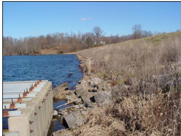
Figure 1-5 Embankment dam with a concrete riser is a common type of dam requiring inspection in Indiana.
