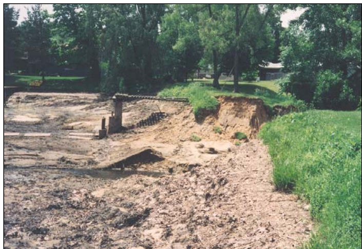
Figure 1-4 Erosive discharge from an uncontrolled dam breach severely impacted the downstream areas.
