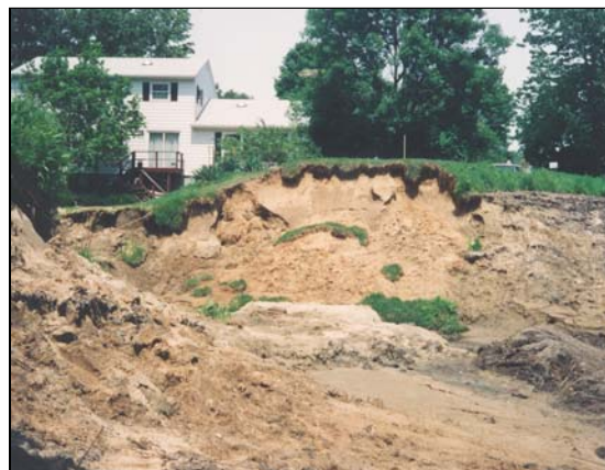
Figure 1-3 The dam owner is responsible for repairing this damage downstream of the dam.
