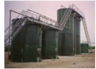
Crude oil tank battery
