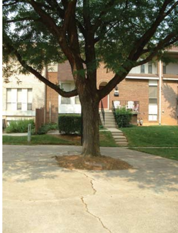
Figure 16. Tree roots cause adjacent pavement to crack.
