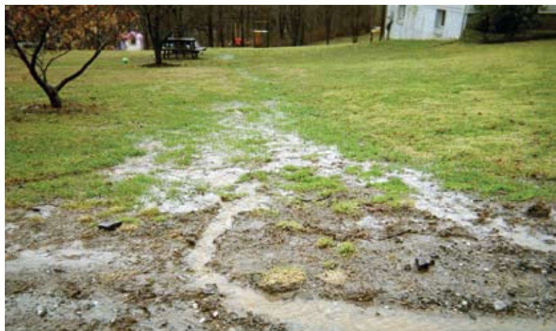
Figure 12. Concentrated flow at this over-capacity site must be dealt with before planting.
