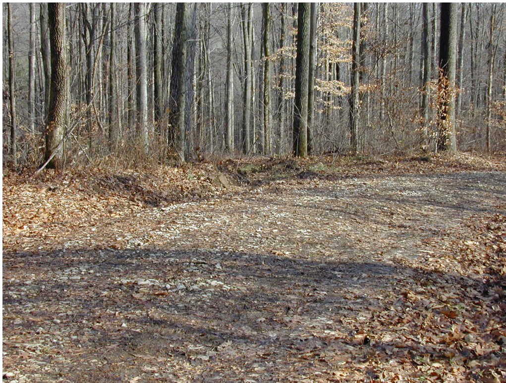
Crowning and cutouts promote good drainage and stable permanent access roads. Photo by Duane McCoy, DNR
