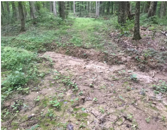
An effective water bar conveying runoff and sediment from a skid trail and diverting the flow onto the forest duff layer, where water will infiltrate the soil, the sediment will be filtered and the water will become groundwater. Photo by Jennifer Sobecki, DNR
