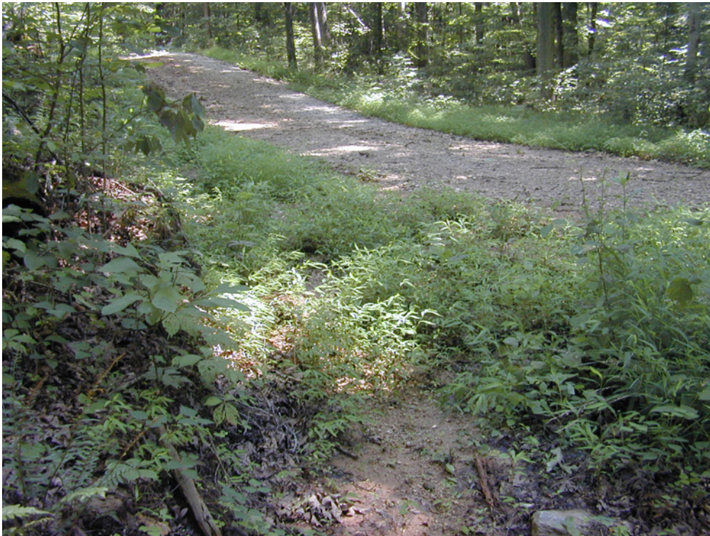
Effective cutout on a permanent access road. Photo by Duane McCoy, DNR
