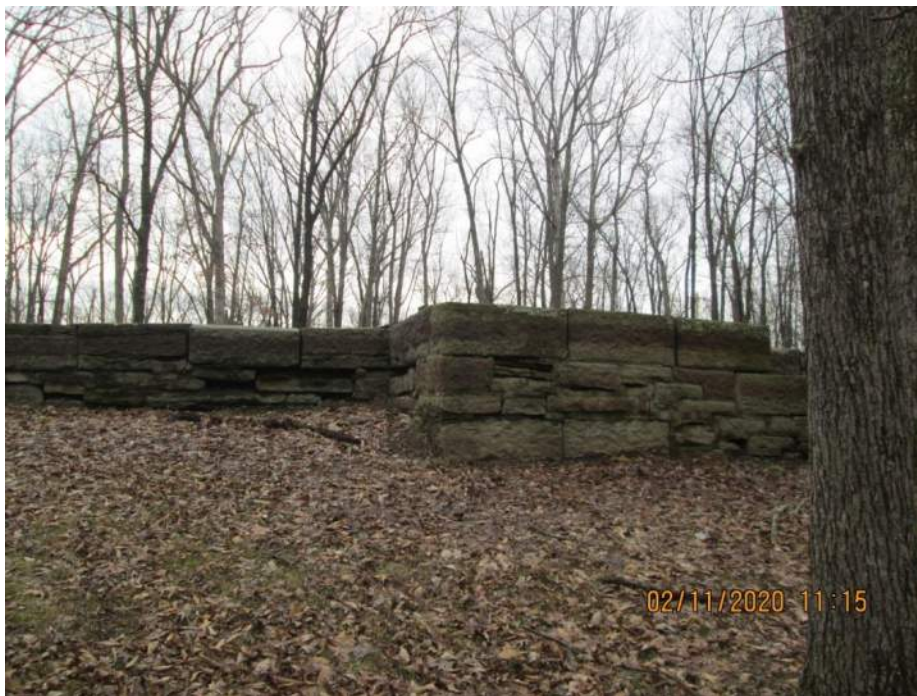
13+50 to 13+75 Delamination Block separation - Stairs
