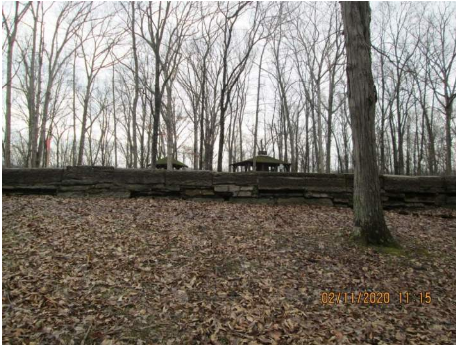
13+75 to 14+00 Delamination Wall Leaning to North
