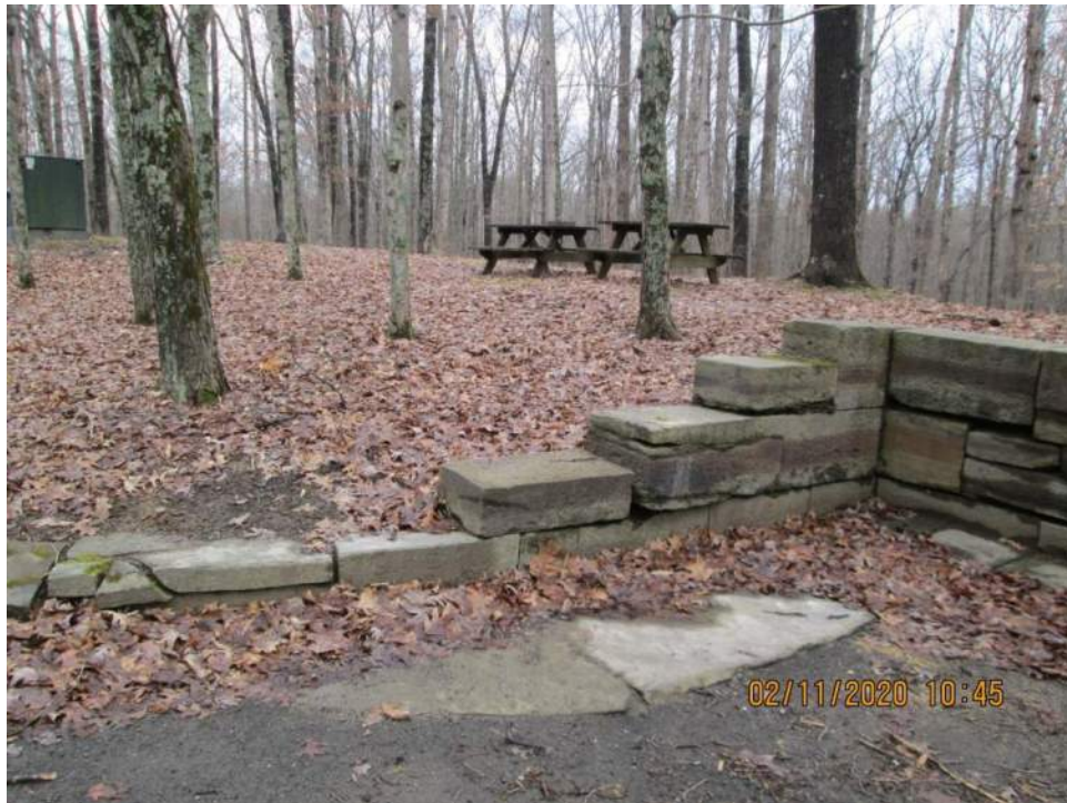
10+00 to 10+30 Minor Delamination
