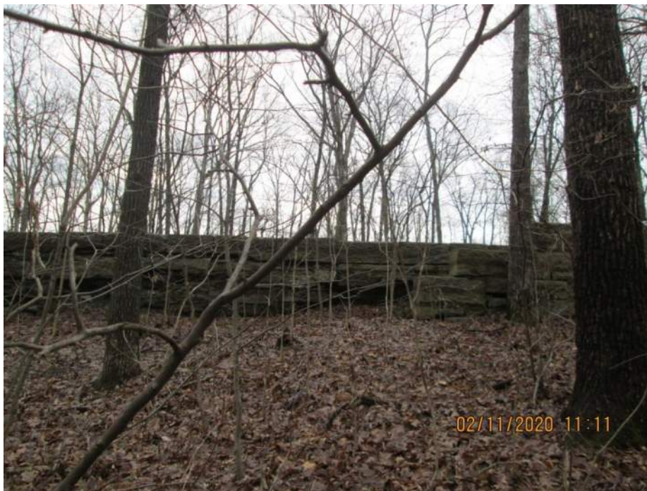
12+50 to 12+75 Block separation – Delamination - Wall Collapse Drainageway at 12+75 following foot path to North
