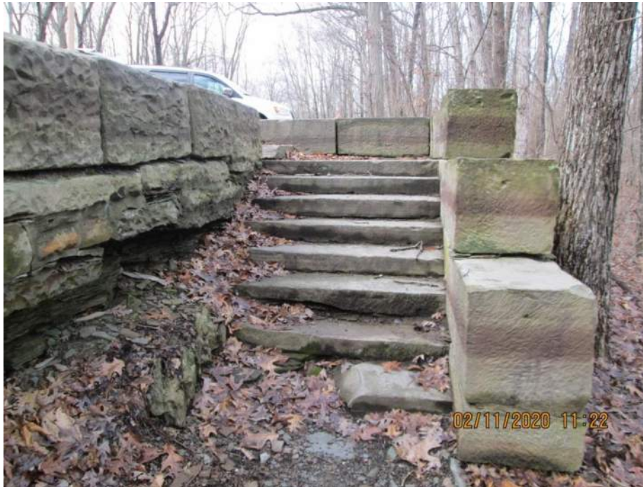
12+50 to 12+75 Detail Delamination – Broken Steps Drainageway at 12+75 following foot path to North
