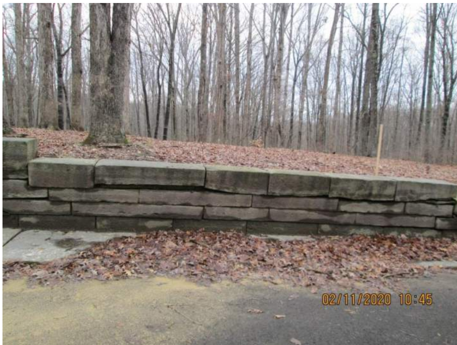
10+30 to 10+50 Minor Delamination Minor Leaning to the South
