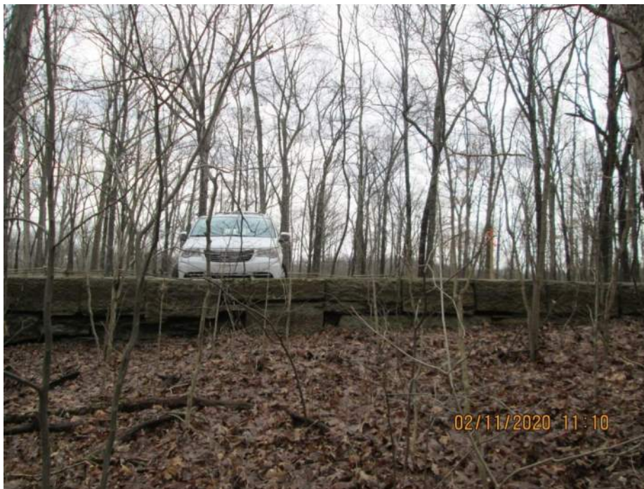
12+00 to 12+25 Block separation – Delamination Isolated Collapse
