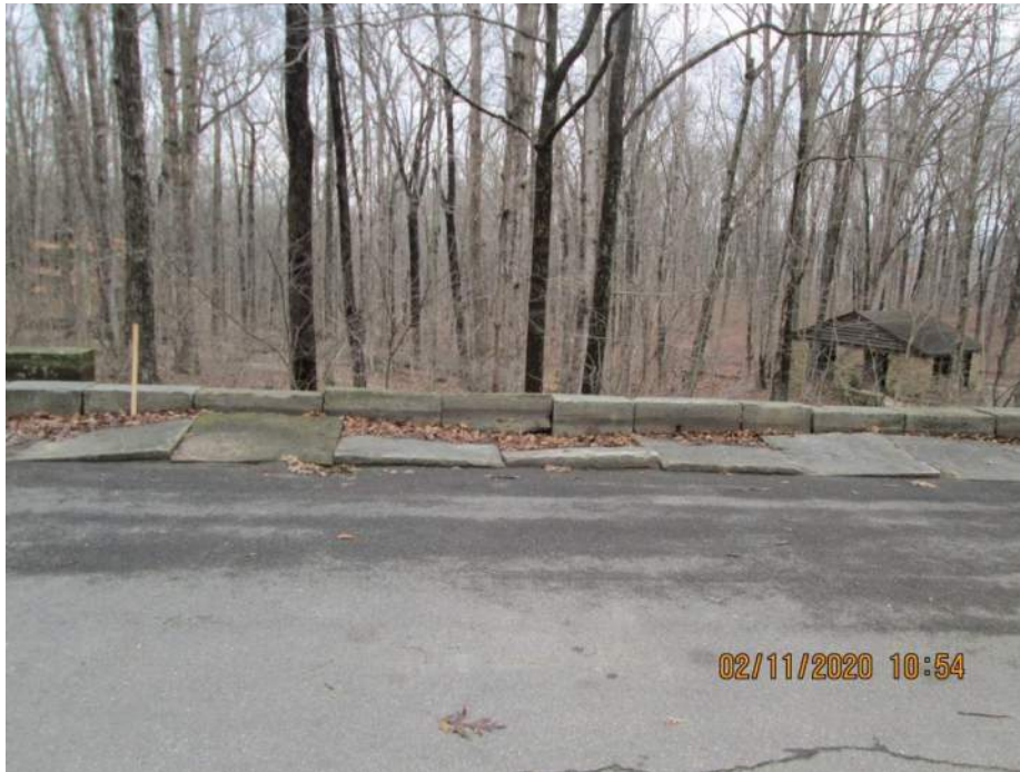
12+50 to 12+75 Block separation Wall leaning to North
