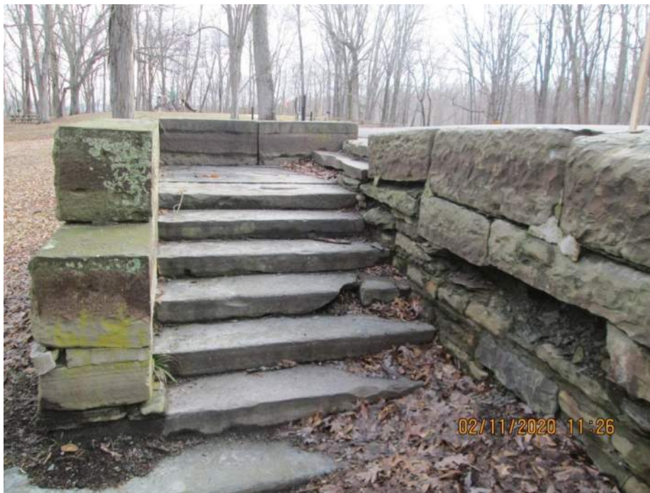
13+50 to 13+75 Detail Delamination Block separation - Stairs
