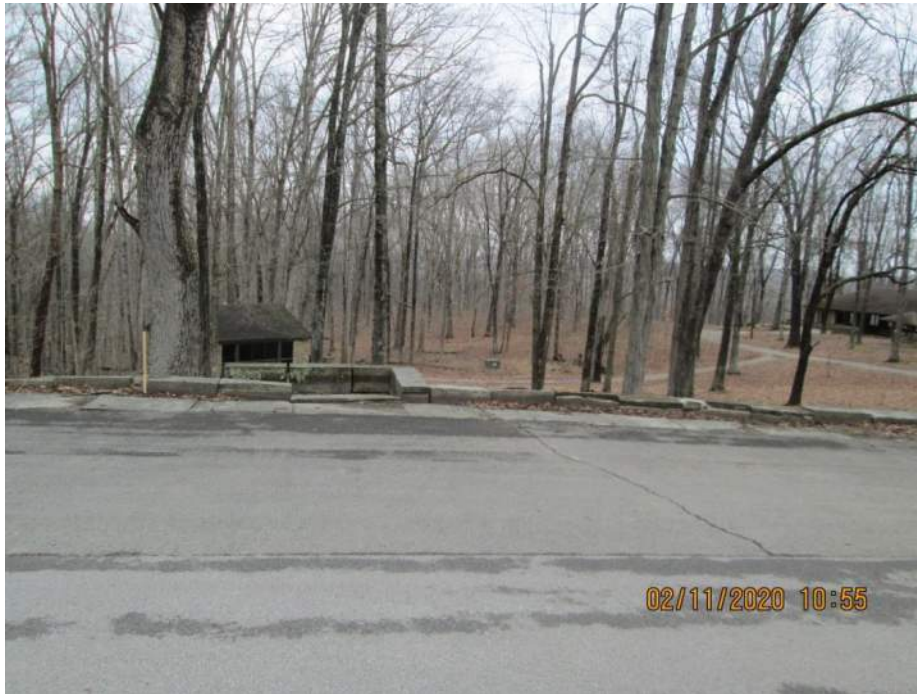
13+50 to 13+75 Block separation - Stairs Wall leaning to North
