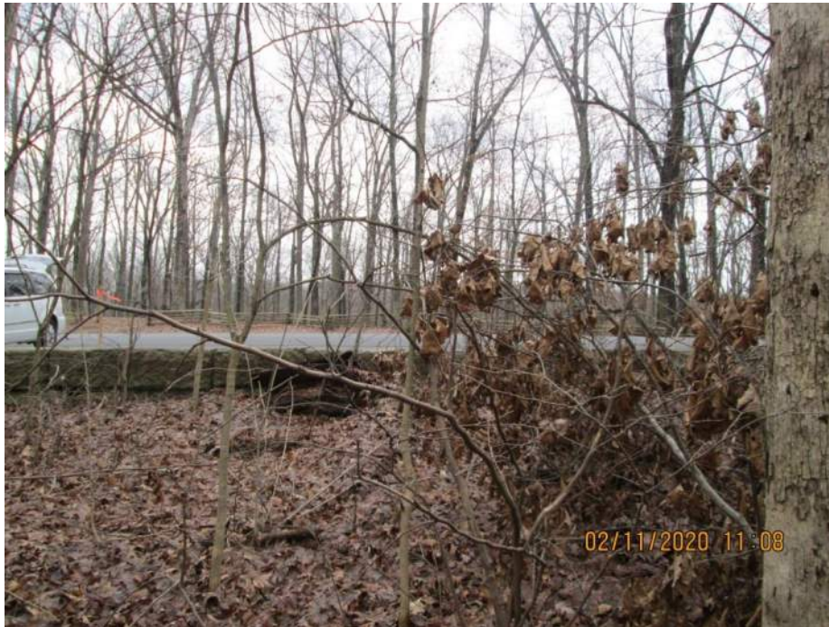
11+75 to 12+00 Wall at Grade – Tree Uprooted
