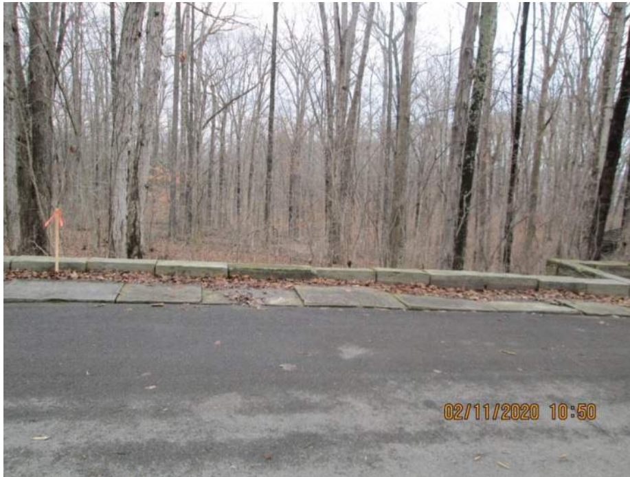
12+00 to 12+25 Blocks and Wall leaning to the North
