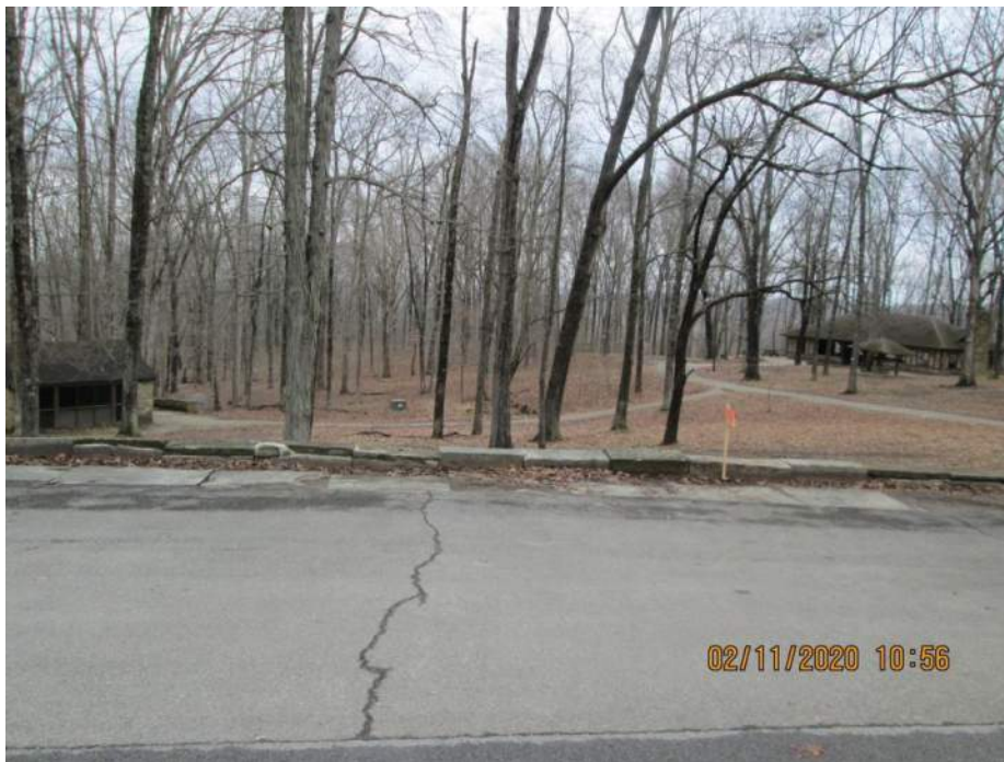
13+75 to 14+00 Block separation North to South Wall leaning to South
