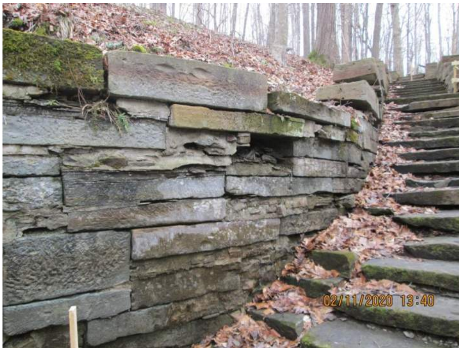
10+28 to 10+40 Delamination - Old Patching 7 steps split
