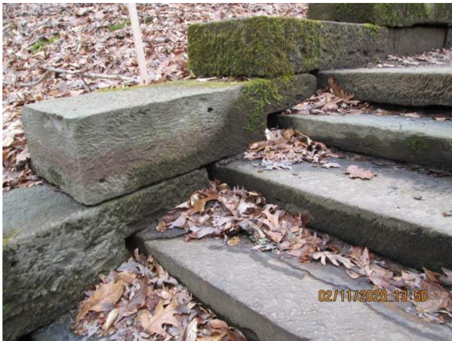
10+75 to 10+85 Isolated landing fragmentation
