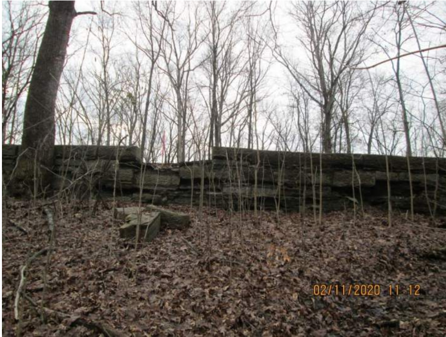
12+75 to 13+00 Block separation - Delamination Wall Collapse
