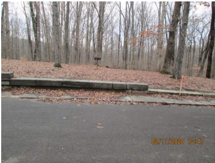
10+75 to 11+00 One block delamination Wall returns to Grade
