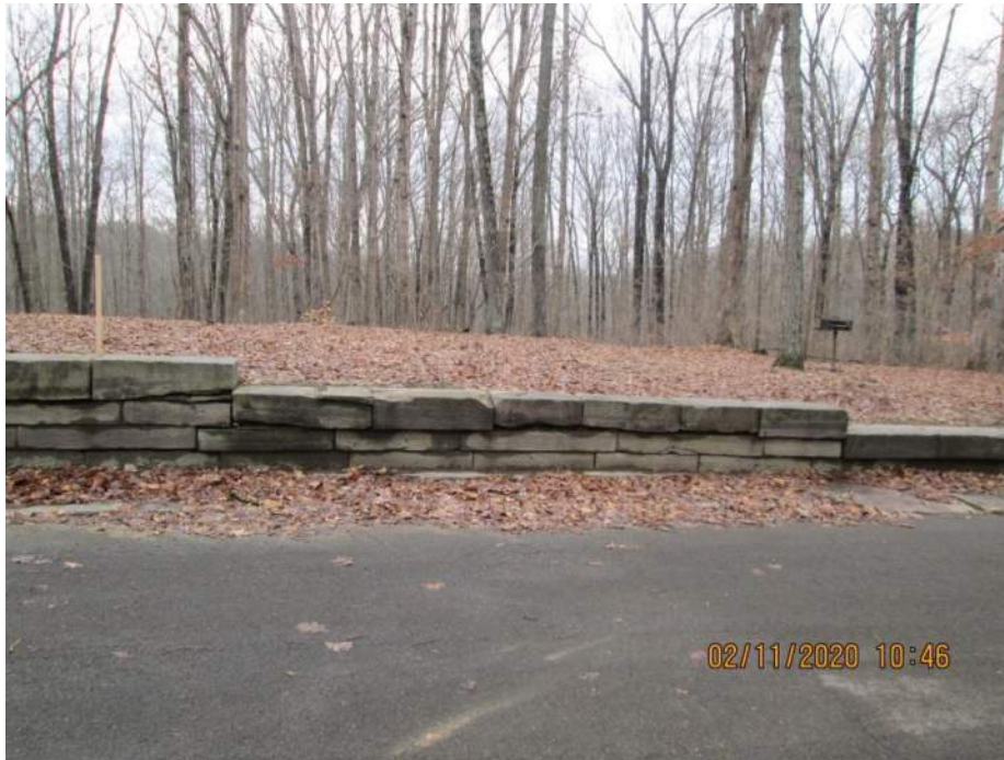
10+50 to 10+75 Minor Delamination
