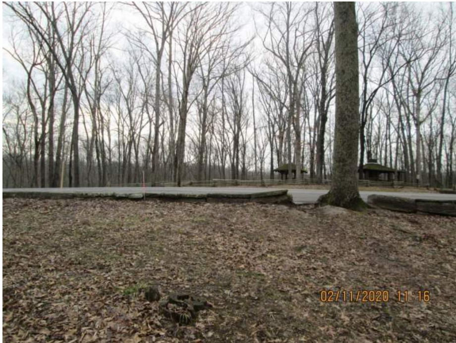
14+25 to 14+50 Wall Heaved - Block Shifting Wall at Grade
