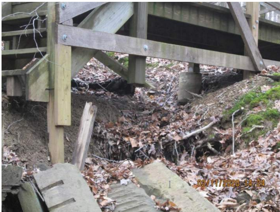
11+00 to 11+20 Wall failure due to drainage - Debris on hillside 4 feet drainage scour
