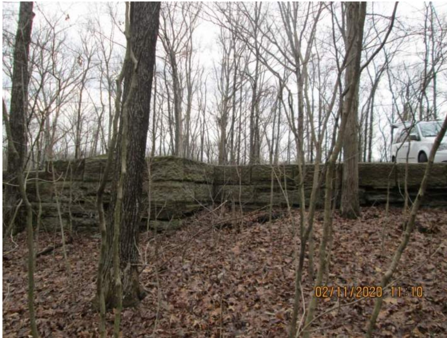
12+25 to 12+50 Block separation - Delamination Isolated Collapse - Stairs – Stone Cracked
