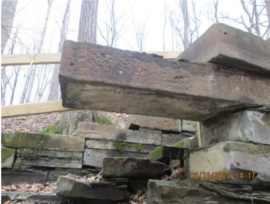
10+45 to 10+66 Total wall failure - Debris on hillside 4 exposed layers under landing
