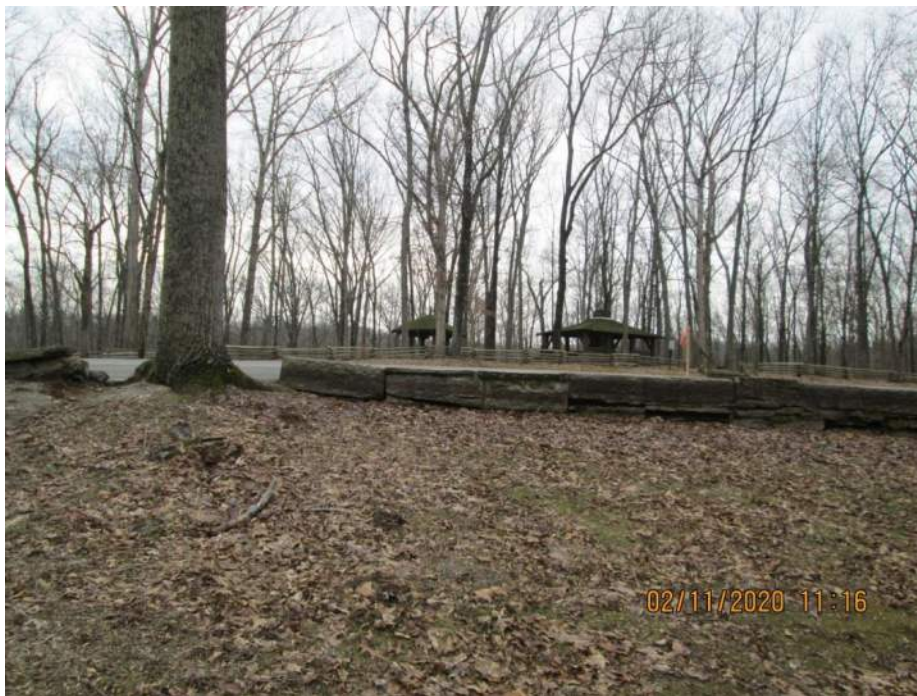
14+00 to 14+25 Block Separation - Delamination Tree in Wall - Heaving at tree
