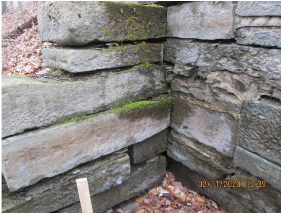
10+05 to 10+28 Landing and Bend - Landing Stone Missing Isolated Delamination - Wall wedged over Walkway
