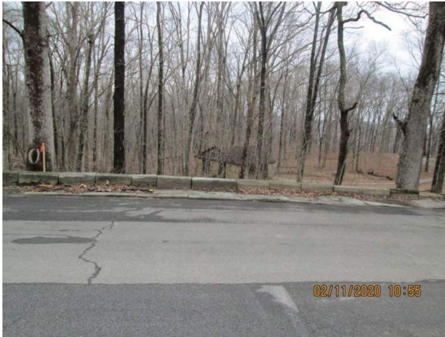
13+00 to 13+25 Block separation Wall leaning to North
