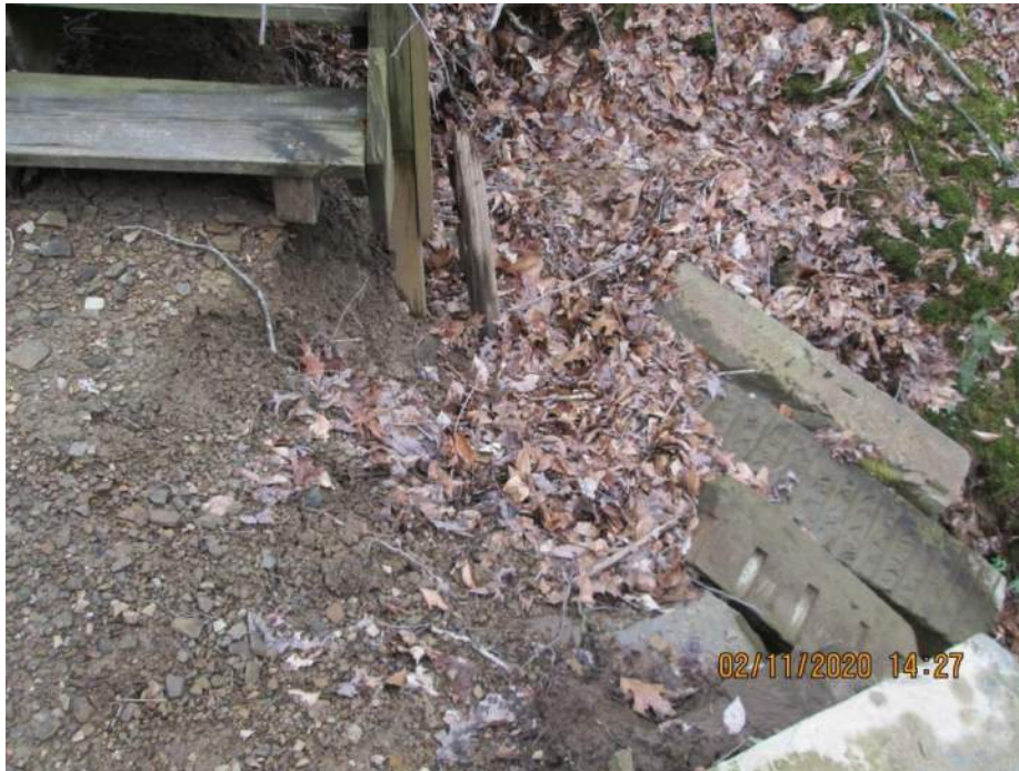
11+00 to 11+20 Wall failure due to drainage - Debris on hillside 4 feet drainage scour
