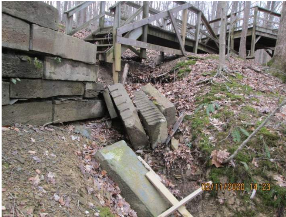
11+00 to 11+20 Wall failure due to drainage - Debris on hillside 4 feet drainage scour
