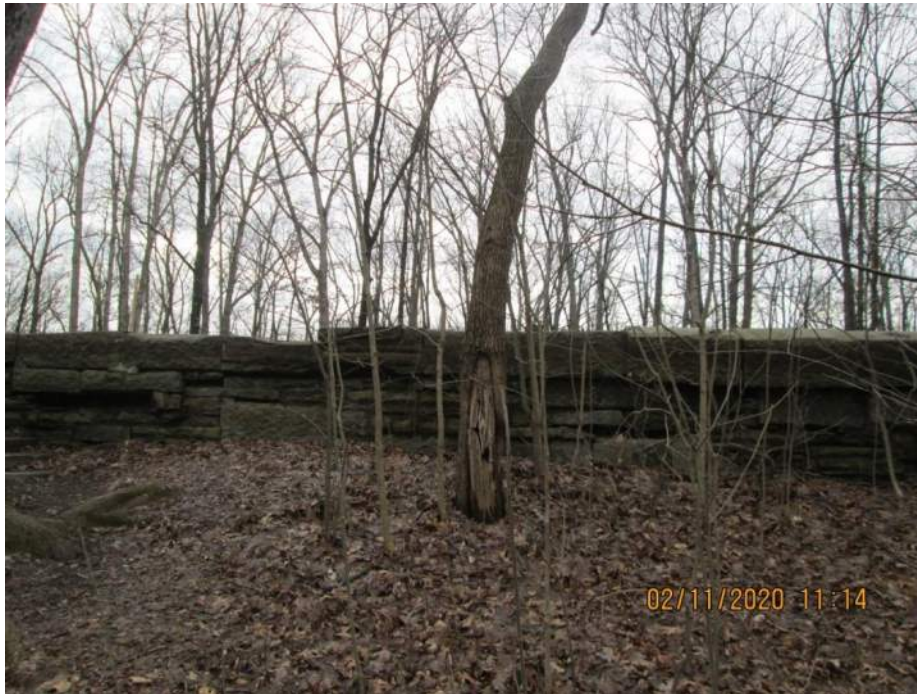
13+25 to 13+50 Delamination – Wall collapse Wall Leaning to North
