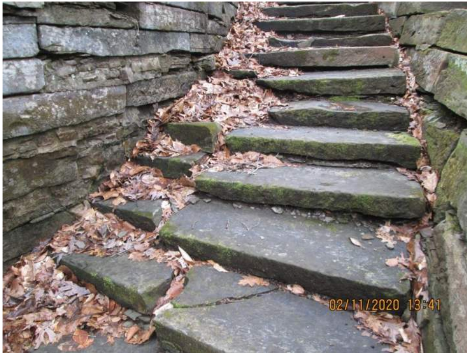
10+28 to 10+40 Delamination - Old Patching 7 steps split
