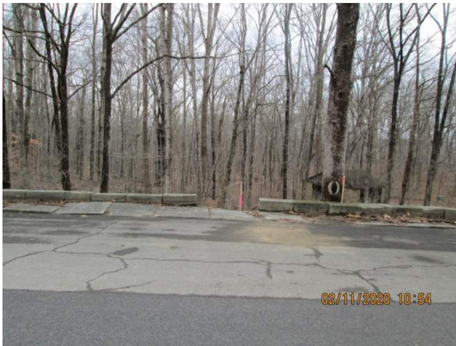
12+75 to 13+00 Wall collapse Block separation
