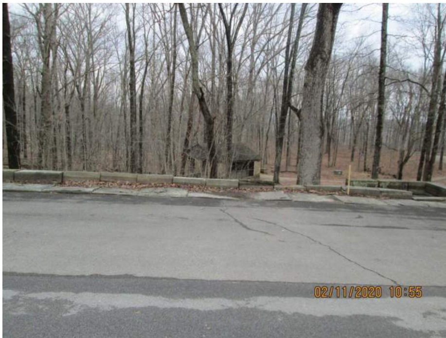
13+25 to 13+50 Block separation - Delamination Wall leaning to North
