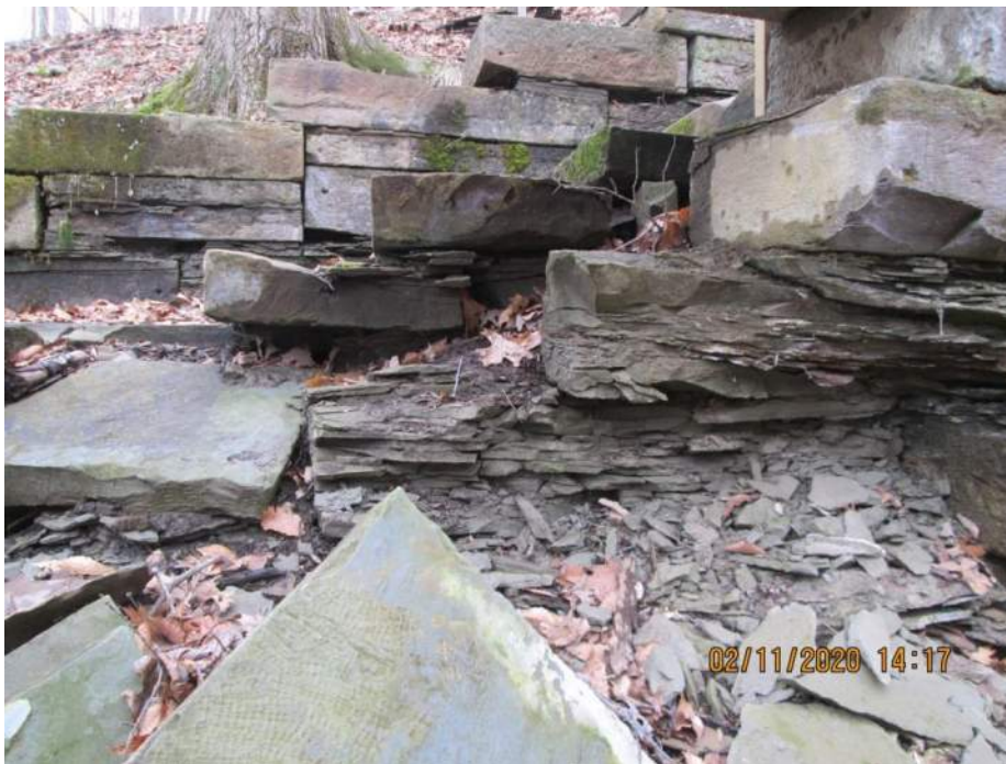
10+45 to 10+66 Total wall failure - Debris on hillside 4 exposed layers under landing
