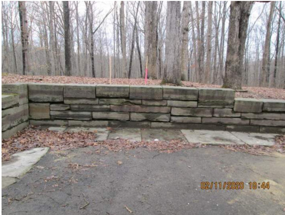
10+00 to 10+30 Minor Delamination
