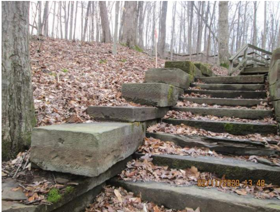
10+75 to 10+85 Isolated landing fragmentation
