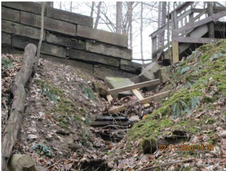
11+00 to 11+20 Wall failure due to drainage - Debris on hillside 4 feet drainage scour
