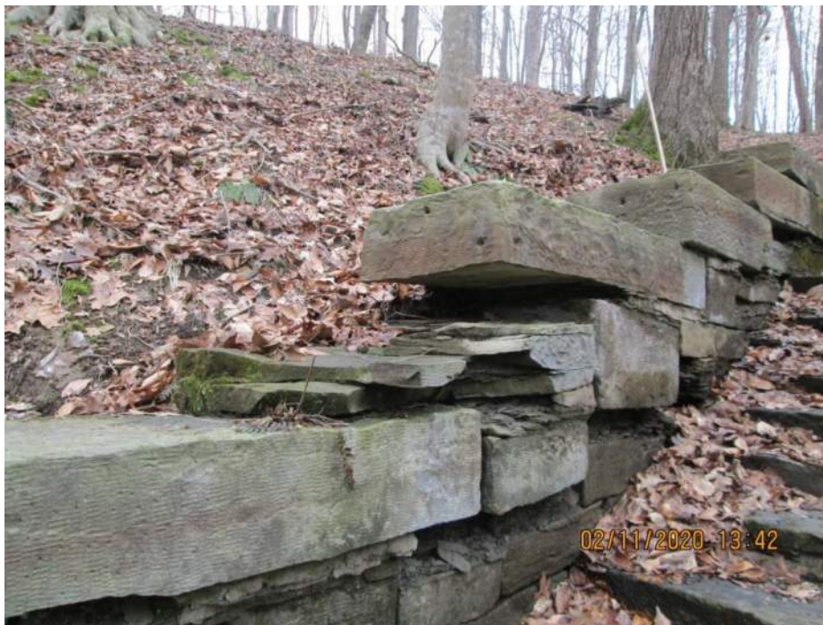
10+40 to 10+50 Excessive Delamination – Steps delaminated Wall wedged over Walkway
