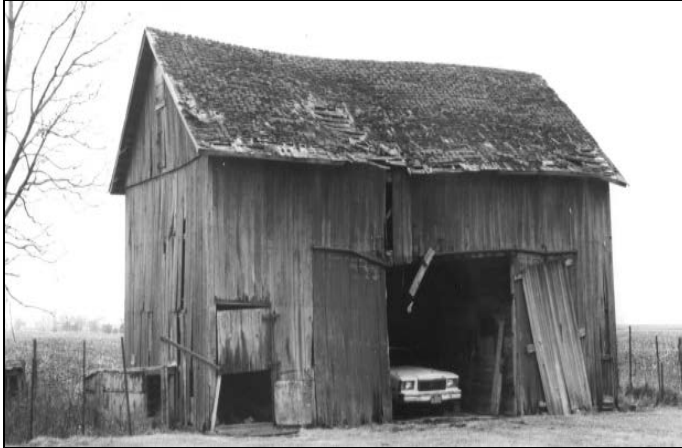
Poor Condition Foundation-Uneven and severely cracked Structure-Unstable Walls-Extremely loose Roof-Unstable
