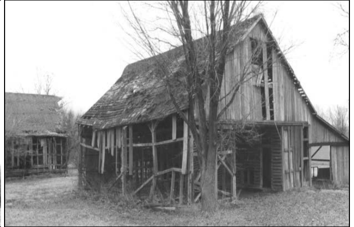
Very Poor Condition Foundation-Crumbled Walls-Limited to lone Structure-Rotted or missing Roof-Collapsing
