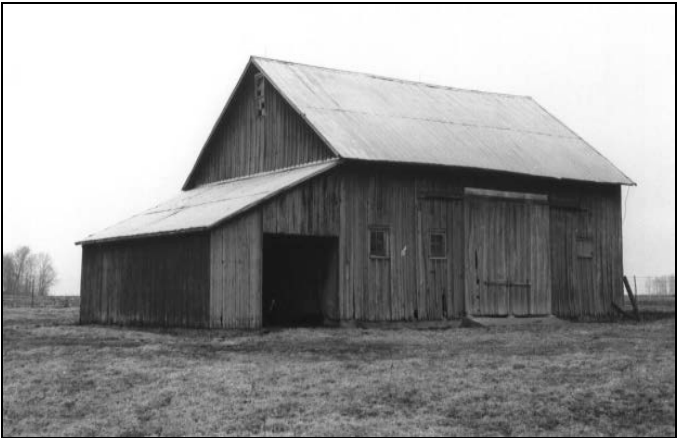
Fair Condition Foundation-Cracked Walls-Intact Structure-Stable Roof-Stable
