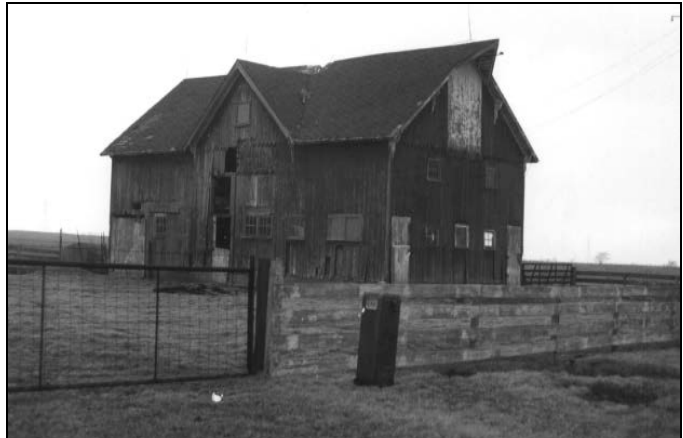
Poor Condition Foundation-Severely cracked Walls-Loose Structure-Weakened Roof-Fairly stable
