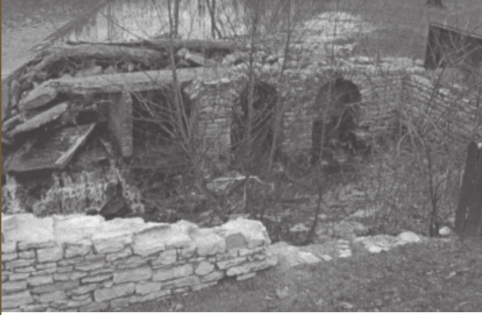
Photograph documenting the grain and sawmill site features at the Markle Mill in Vigo County (Cantin 2004:39).
