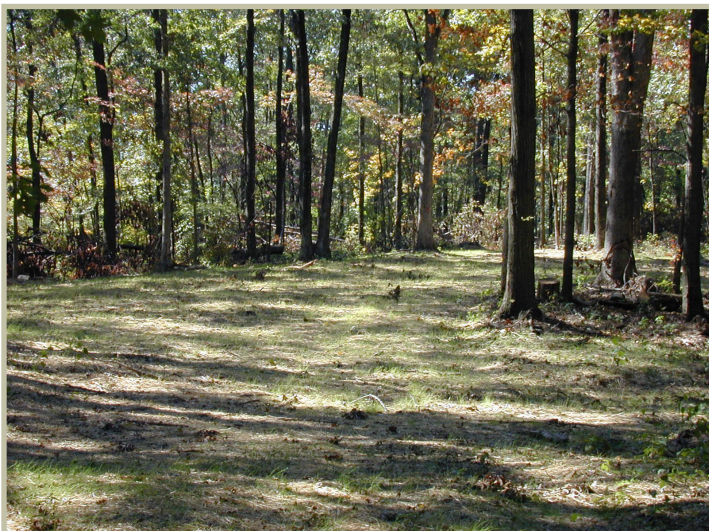
Seed and straw on a skid trail stabilize and protect soil until new vegetation can be established.
