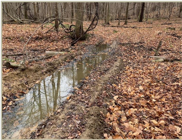
There are multiple issues with this stream crossing. The culvert is too small, causing a backup of water on the upstream side. Water was not diverted from the trail, and the trail was not armored as it crossed the stream, so there is ponding and very muddy conditions on the crossing.
