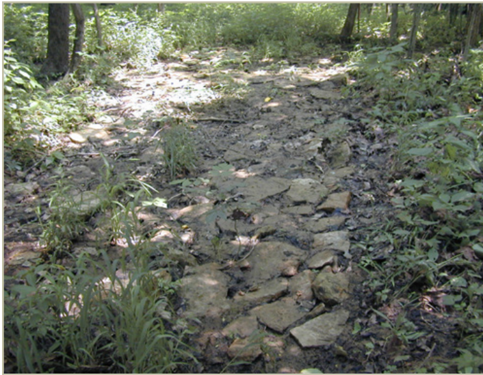
This stream crossing is lined with flat rocks that protect the approaches and stream bed.
