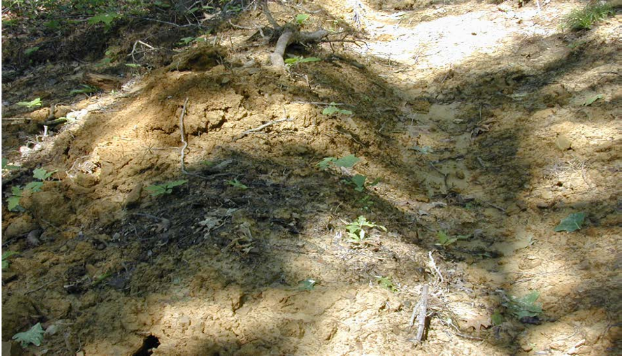
An effective water bar conveying runoff from a skid trail and diverting the flow onto the forest duff layer, where it will infiltrate, remove sediment and return to groundwater.
