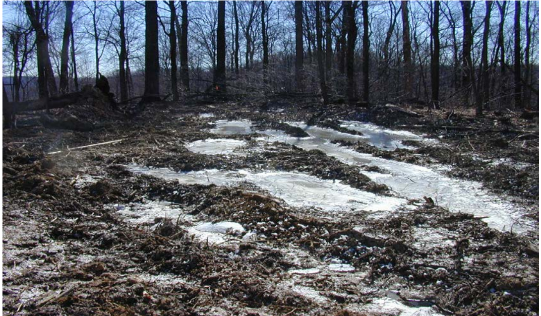
Log landing that was used during a wet period, causing rutting and the site to collect runoff.
