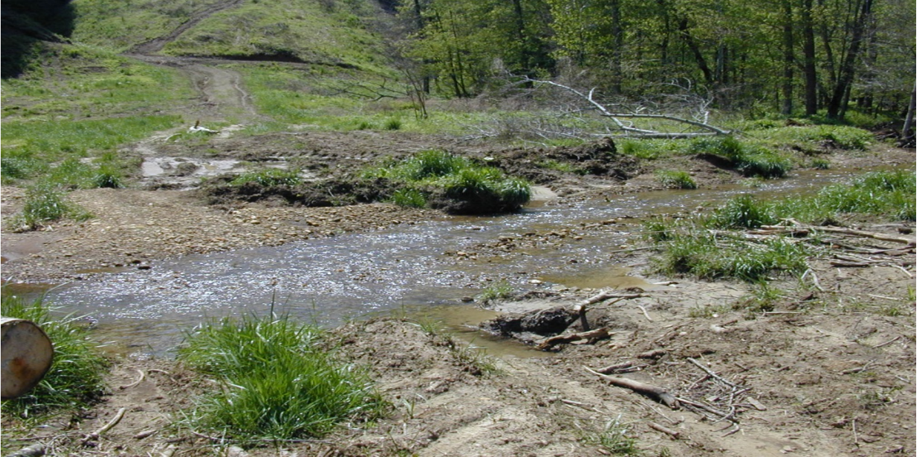
On a private site: No water diversions before stream crossing. No stream bank stabilization/revegetation.
