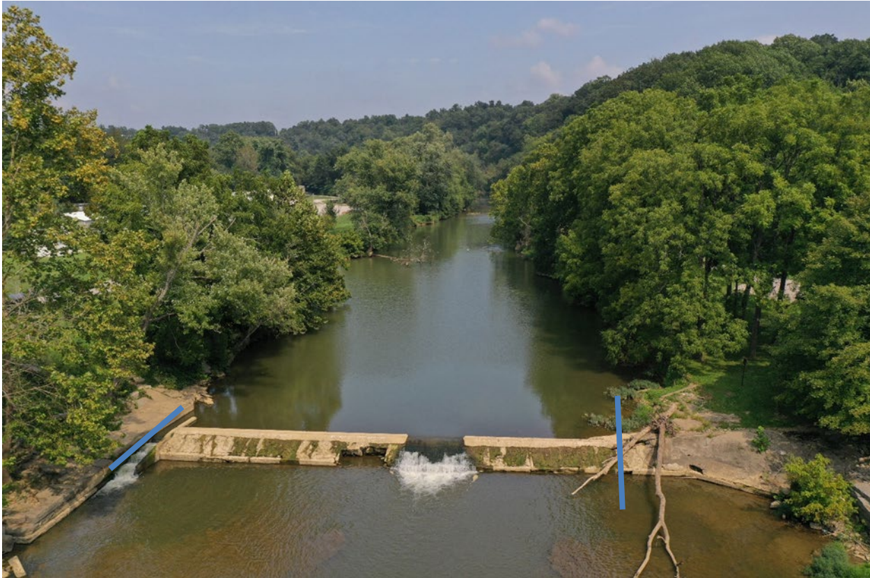
Figure 18. Drone picture from downstream the dam looking upstream. Photo taken 24 August 2023. Corydon (Gupta) dam, Corydon Indiana. Between the blue lines (left and right) indicate the approximate area of the dam that will be removed.
