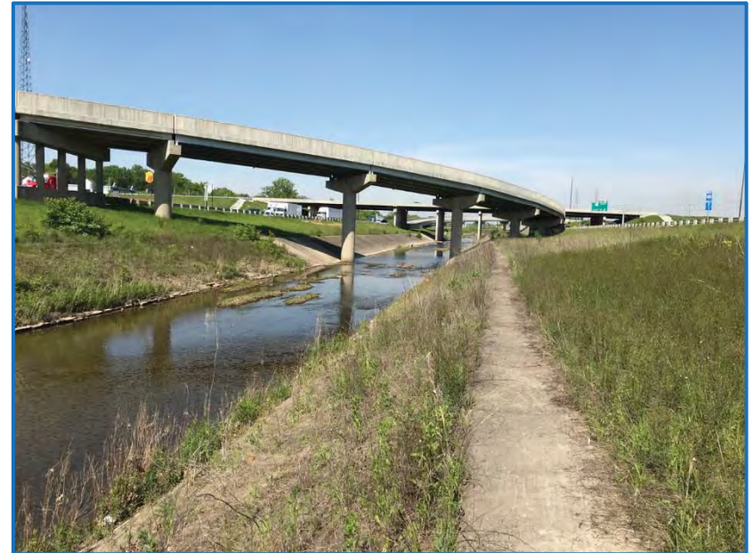
Photo 14 – View downstream of Lick Creek in the median of I-465 east of East Street facing northeast (5-14-19).
