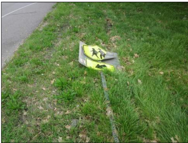
Fallen Pedestrian Crossing Sign on the SE Corner
