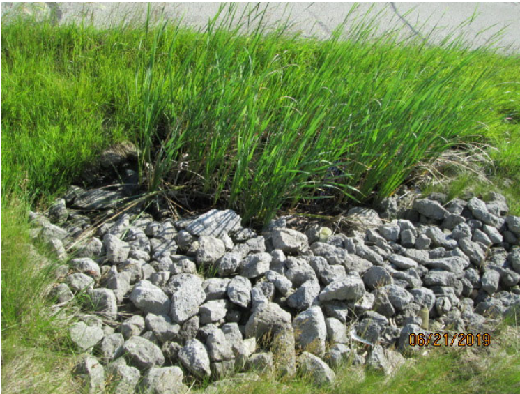
Photo 17: Southwest Quadrant Looking northeast towards US 30 at riprap with cattails in RSD-2.
