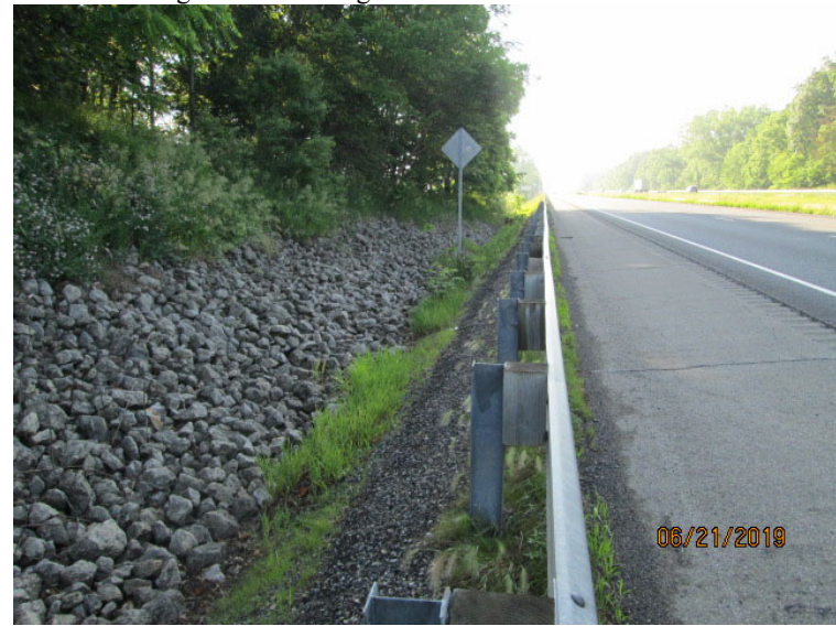
Photo 4: Northeast Quadrant Looking southeast along the north side of US 30 at RSD-1.
