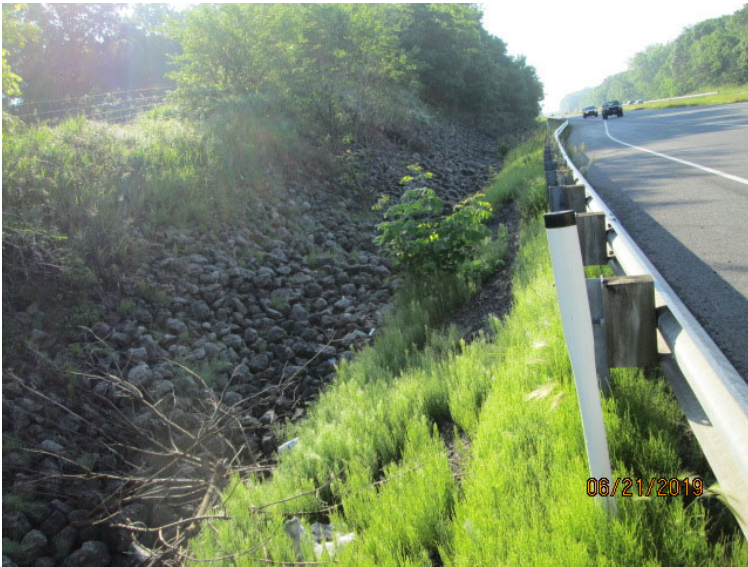
Photo 1: Northeast Quadrant Looking southeast along the north side of US 30 at RSD-1.
