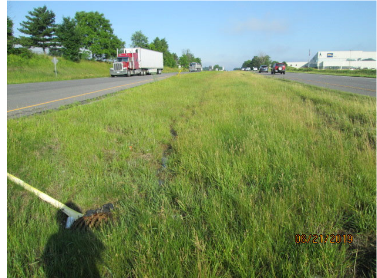
Photo 11: Western Median Looking northwest in the median on the west side of the intersection of US 30/CR 500 E. Shown inlet is Structure No. 100 on plans.
