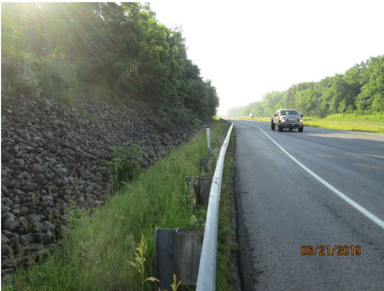
Photo 2: Northeast Quadrant. Looking southeast along the north side of US 30 at RSD-1.
