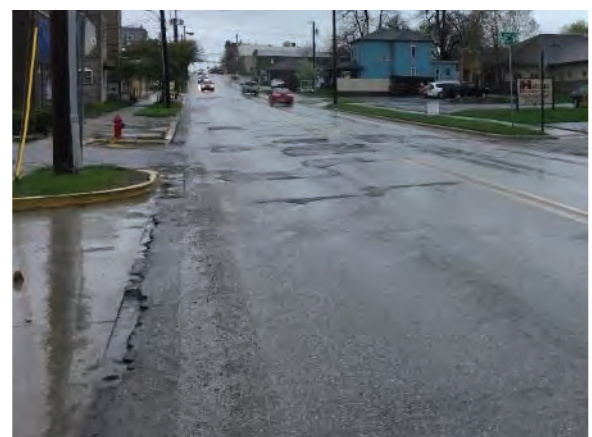
Figure 4: Looking south at a typical view of the pavement condition on Jackson Street.
