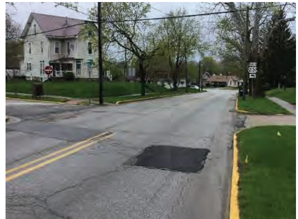
Figure 2: Looking northwest at the typical pavement condition of Bloomington Street within the Eastern Enlargement Historic District.
