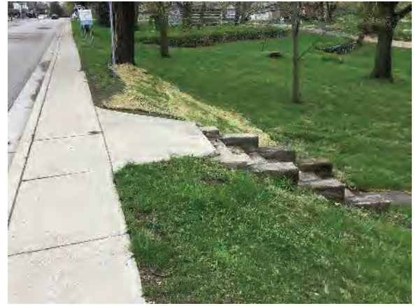
Figure 11: Looking northeast at contemporary concrete landing to be replaced in kind and concrete steps to be avoided.
