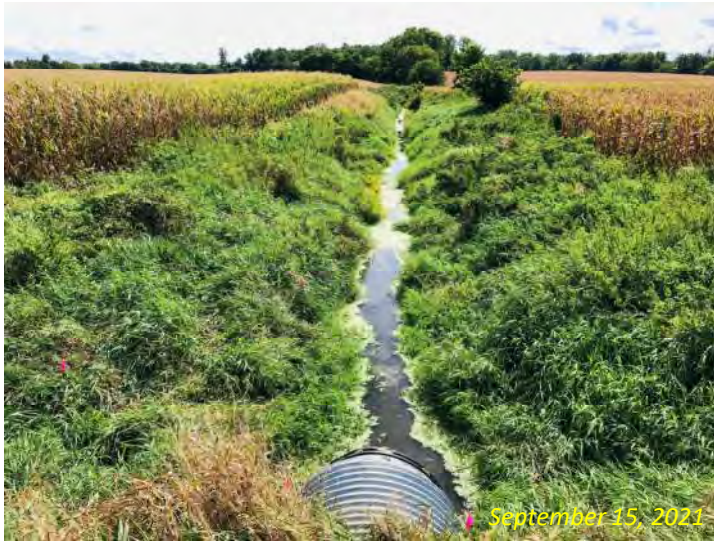
Photo 11: View south from the small structure along the south side of SR 8. UNT to Rimmel Branch is also shown.
