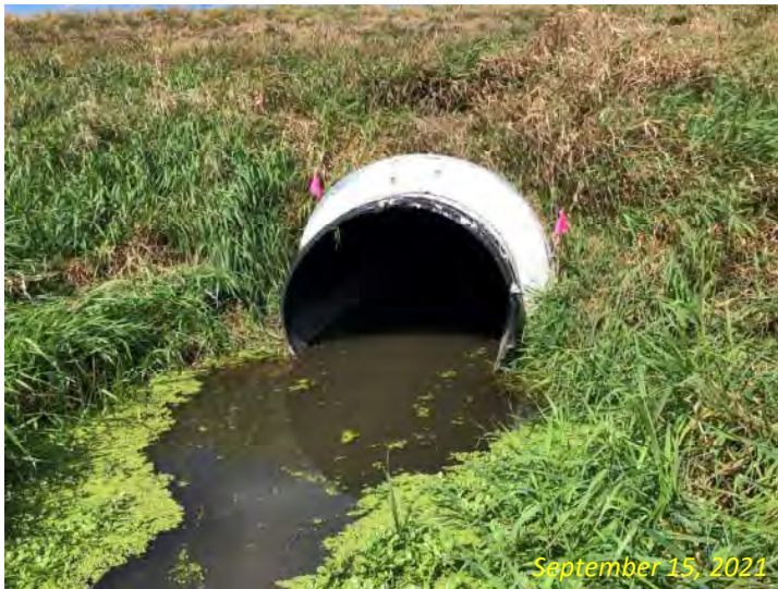
Photo 7: View north (upstream) along UNT to Rimmel Branch on the south side of SR 8. Structure CV 008-057-47.08 is also shown.
