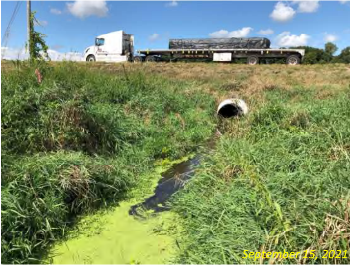
Photo 5: View north (upstream) along UNT to Rimmel Branch on the south side of SR 8. Structure CV 008-057-47.08 is also shown.
